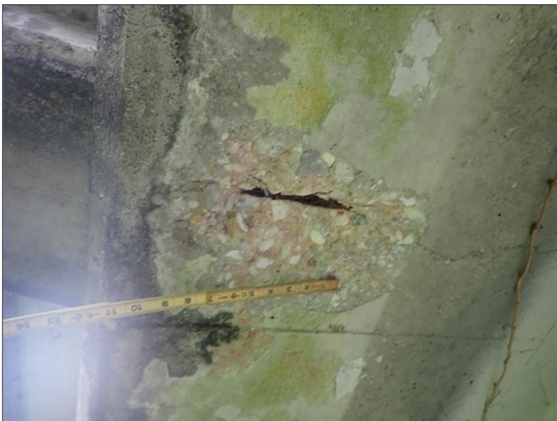
Span 2 Deck: (PAR) RIGHT OVERHANG SOFFIT AT RAIL POST 2, 1 FOOT DIAMETER X 1.5 INCHES DEEP SPALL WITH EXPOSED REBAR. 5 PERCENT SECTION LOSS.
