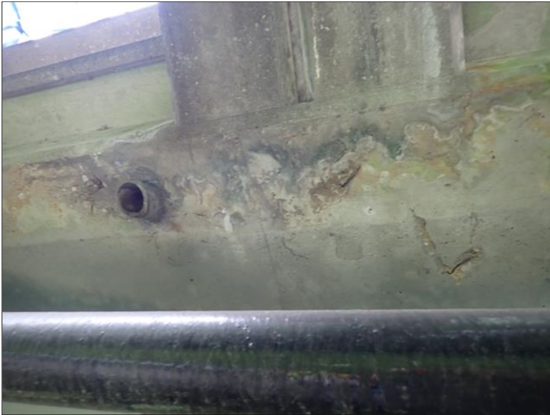
Span 1 Deck: TWO (2) 12 INCHES DIAMETER X 1/2 INCH DEEP DELAMINATIONS/SPALLS, UNDERSIDE OF WEST OVERHANG, AT DRAIN 6.
