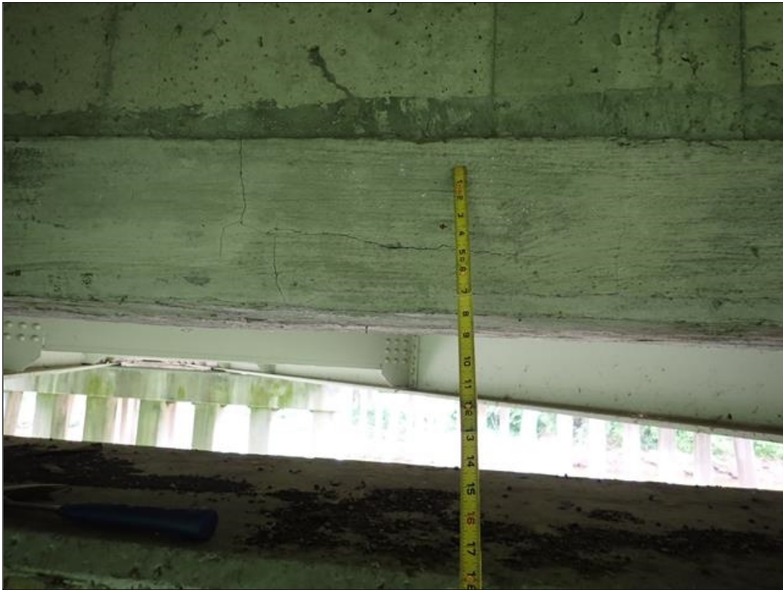
Span 2 Deck: 9 FEET LONG X 1 FOOT HIGH CONCRETE PATCH, BAY 2 END DIAPHRAGM, AT BENT 2. PATCH EXHIBITS UP TO 1/8 INCH WIDE X 5 FEET LONG CRACK IN THE BOTTOM FACE WITH A 5 FEET LONG X 5 INCHES WIDE UNSOUND CONCRETE AND UP TO 0.02 INCH WIDE VERTICAL CRACKS IN FRONT FACE, SCATTERED.
