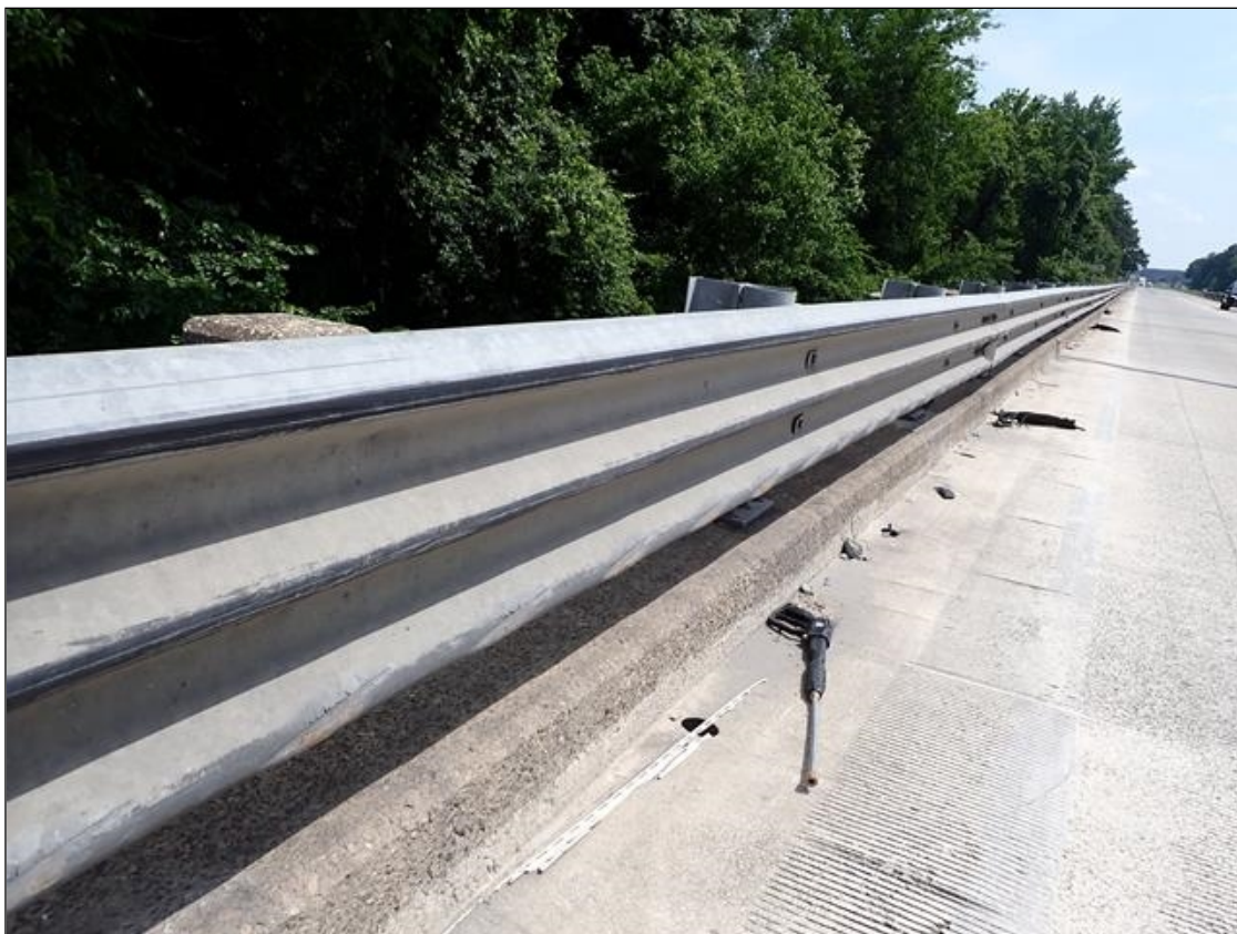
Span 1 Left Retrofit Bridge Rail: (PAR) IMPACT DAMAGE WITH SCRAPE MARKS AND DENTS UP TO 1 INCH DEEP IN RETROFIT RAIL AT SCATTERED LOCATIONS
