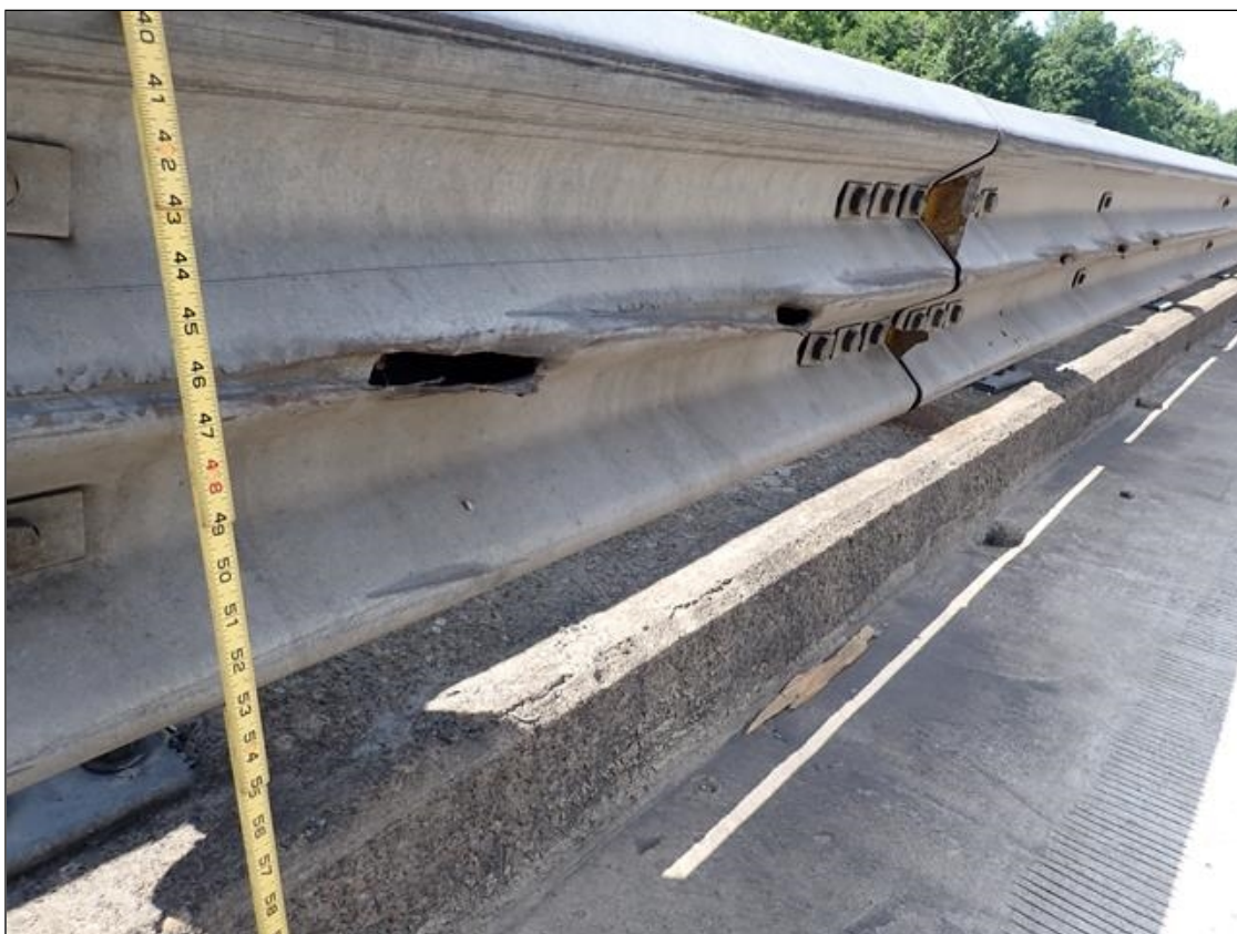
Span 7 Right Retrofit Bridge Rail: (PAR) IMPACT DAMAGE WITH SCRAPE MARKS AND THROUGH HOLES UP TO 4 INCH X 2 INCH IN RETROFIT RAIL AT SCATTERED LOCATIONS
