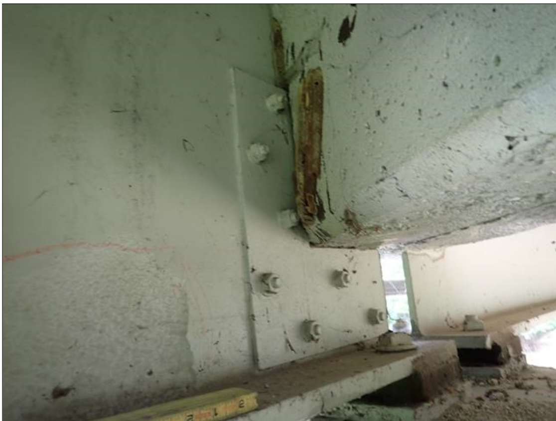
Span 3 Beam 1: at bent 3, web repair plate (3/8 inch thick x 18 inch x 15 inch)
