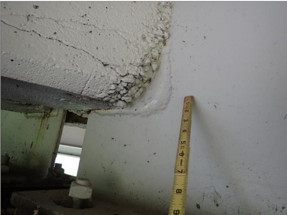
Span 6 Beam 2: (PAR) at bent 6, web adjacent to end diaphragm, painted over section loss (7/16 inch average remaining x 7 inch x 8 inch) with corrosion reactivating
