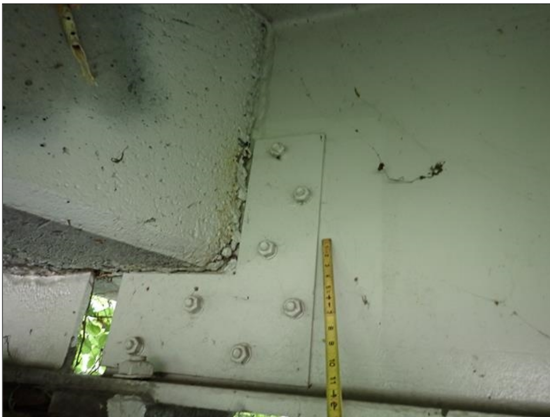
Span 8 Beam 1: (PAR) at bent 7, web adjacent to end diaphragm, painted over section loss (1/2 inch average remaining x 1 inch x 10 inch)
