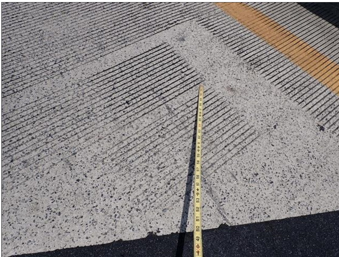
Span 1 Deck: UP TO 5 FEET LONG X 1/32 INCH WIDE LONGITUDINAL AND DIAGONAL CRACKS IN BOTH TRAVEL LANES, SCATTERED.
