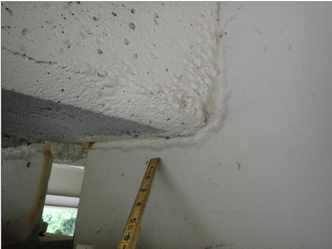
Span 5 Beam 3: (PAR) at bent 4, web adjacent to end diaphragm, painted over section loss (7/16 inch average remaining x 8 inch x 8 inch) with corrosion reactivating
