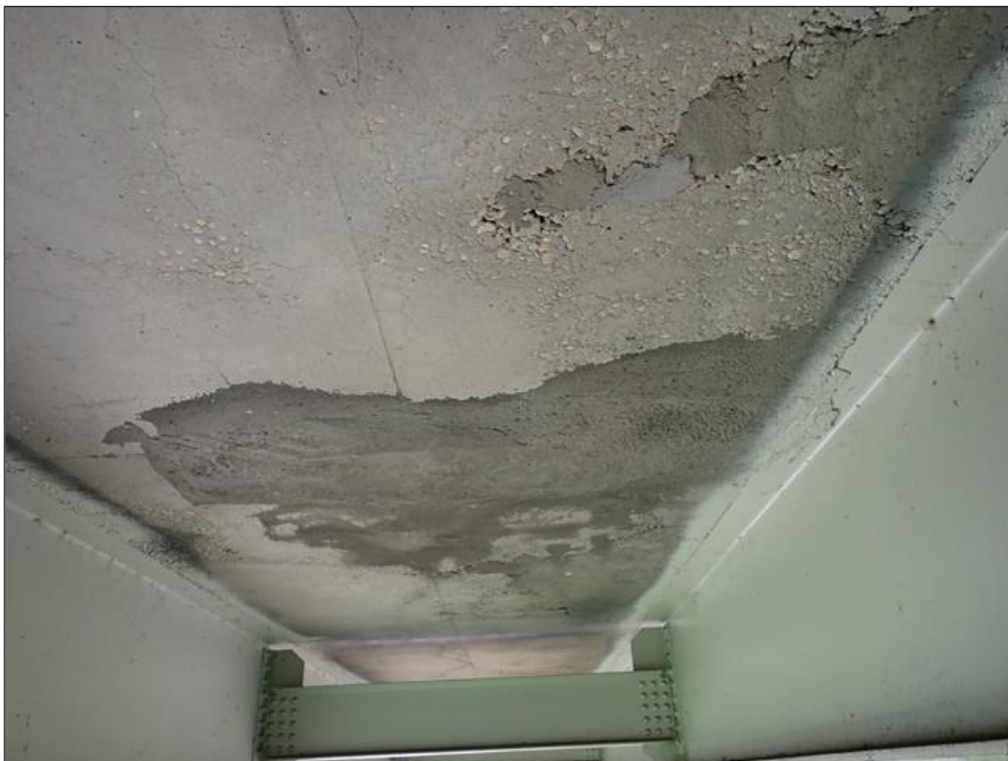
Span 7 Deck: 75 SQUARE FEET OF PATCHED AREA, UNDERSIDE OF DECK, AT RANDOM THROUGHOUT ALL BAYS.
