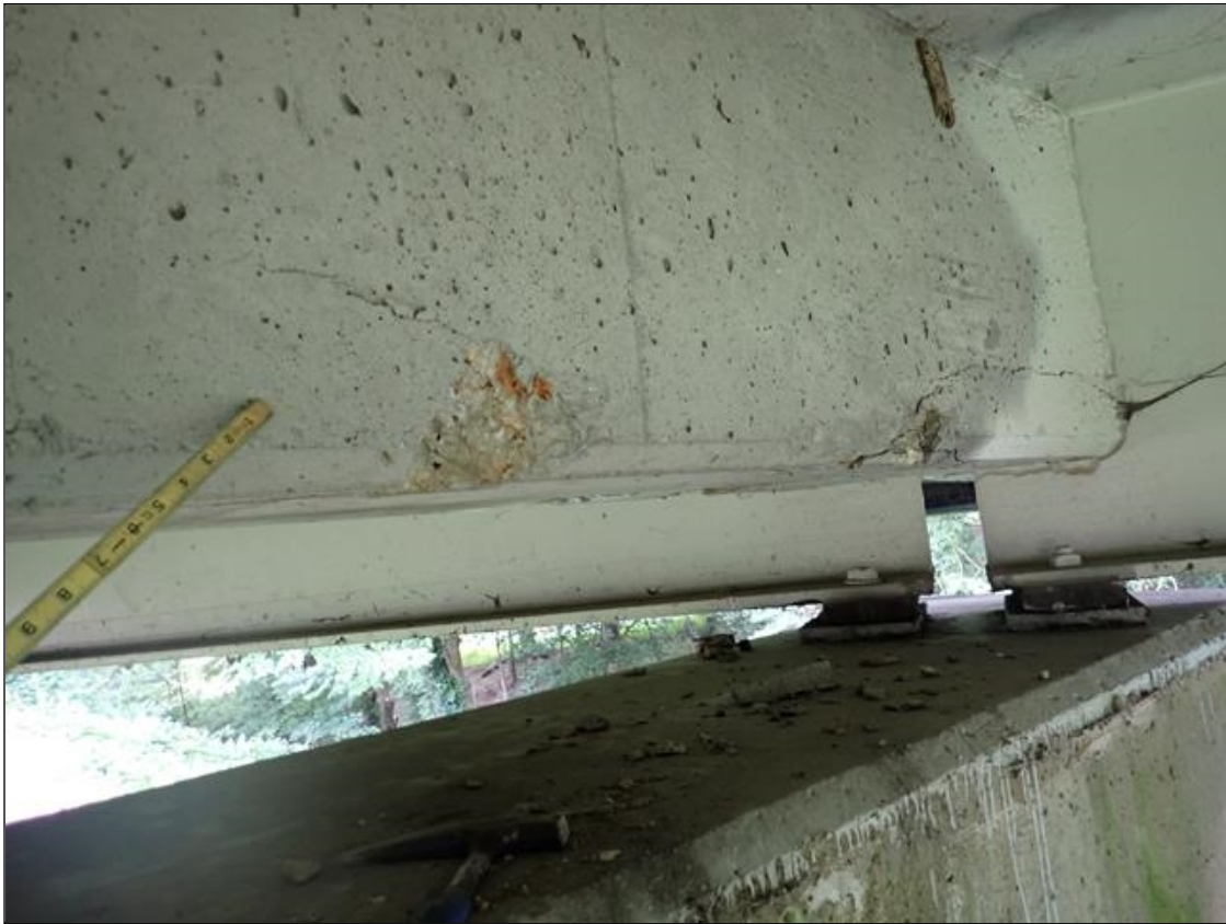
Span 2 Deck: TWO (2) AREAS OF UNSOUND CONCRETE UP TO 2.5 FEET LONG X 1 FOOT HIGH WITH SPALLING UP TO 5 INCHES DIAMETER X UP TO 4 INCHES DEEP IN END DIAPHRAGM IN BAY 1 AT BENT 1.
