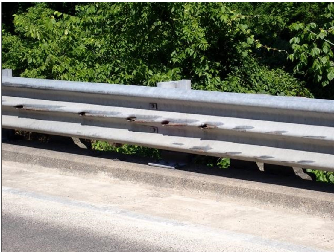
Span 8 Left Retrofit Bridge Rail: (PAR) IMPACT DAMAGE WITH SCRAPE MARKS AND THROUGH HOLES IN RETROFIT RAIL AT SCATTERED LOCATIONS
