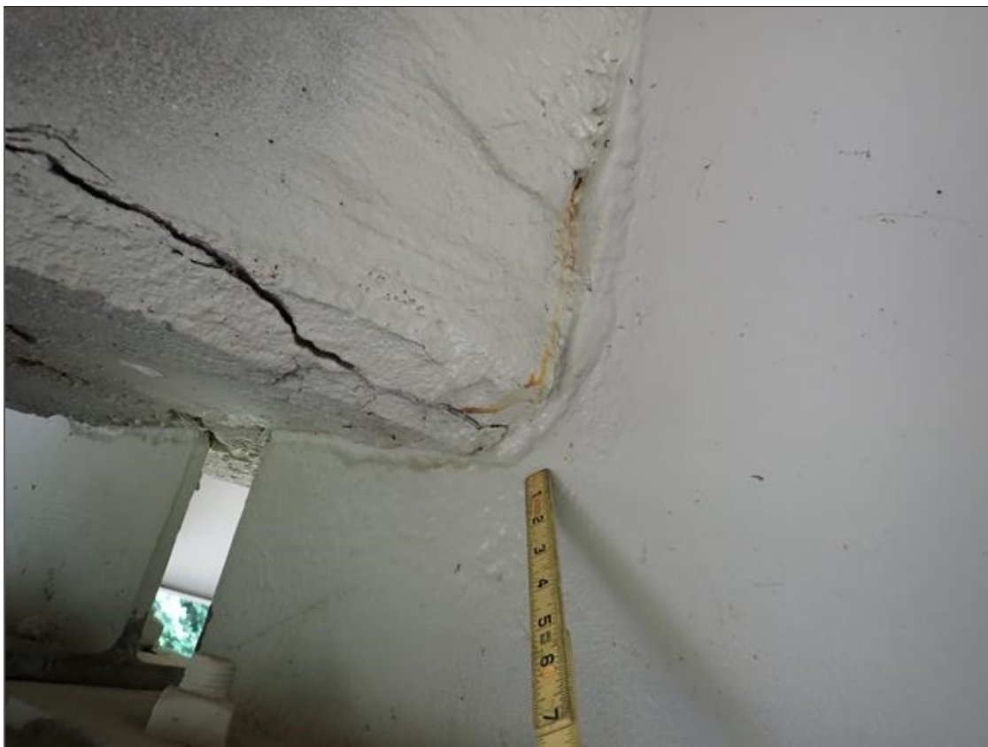
Span 5 Beam 2: (PAR) at bent 4, web adjacent to end diaphragm, painted over section loss (7/16 inch average remaining x 8 inch x 12 inch) with corrosion reactivating
