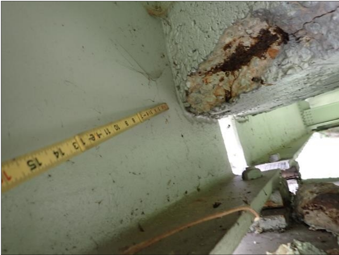
Span 2 Beam 4: (PAR) at bent 1, web adjacent to end diaphragm, painted over section loss (7/16 inch average remaining x 8 inch x 4 inch) with corrosion reactivating
