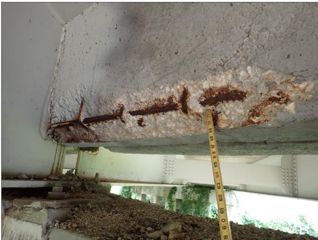
Span 6 Deck: (PAR) 4 FEET WIDE X 10 INCHES LONG X UP TO 6 INCHES HIGH AREA OF UNSOUND CONCRETE AND SPALL WITH EXPOSED REINFORCEMENT IN BAY 3 END DIAPHRAGM AT BENT 6. 10 PERCENT SECTION LOSS IN EXPOSED REBAR.
