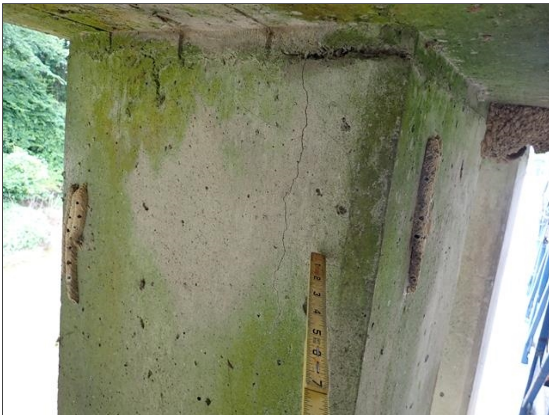
Bent 4 Pile 2: UP TO 1 FOOT LONG VERTICAL HAIRLINE CRACK, EAST AND SOUTH FACES, BEGINNING AT CAP.
