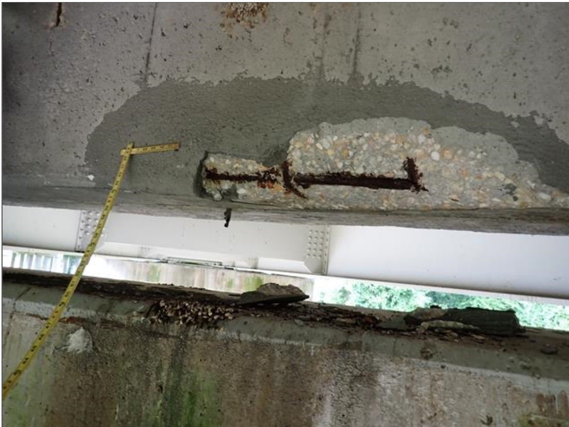
Span 6 Deck: (PAR) bay 2 end diaphragm at bent 5, failed patch/delamination (6 foot x 16 inch x 3 inch deep) with exposed rusted rebar (approximately 100 percent section loss)
