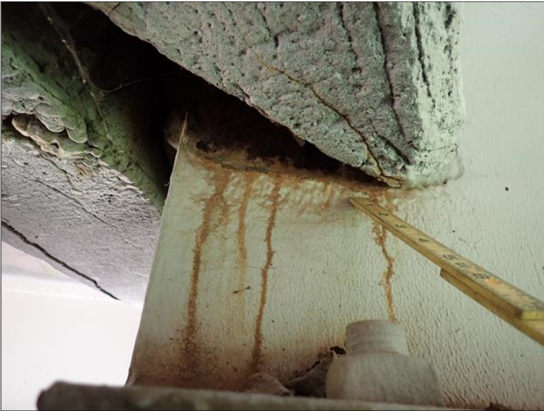
Span 7 Beam 2: (PAR) at bent 6, web adjacent to end diaphragm, corrosion with section loss (7/16 inch average remaining x 7 inch x 10 inch)
