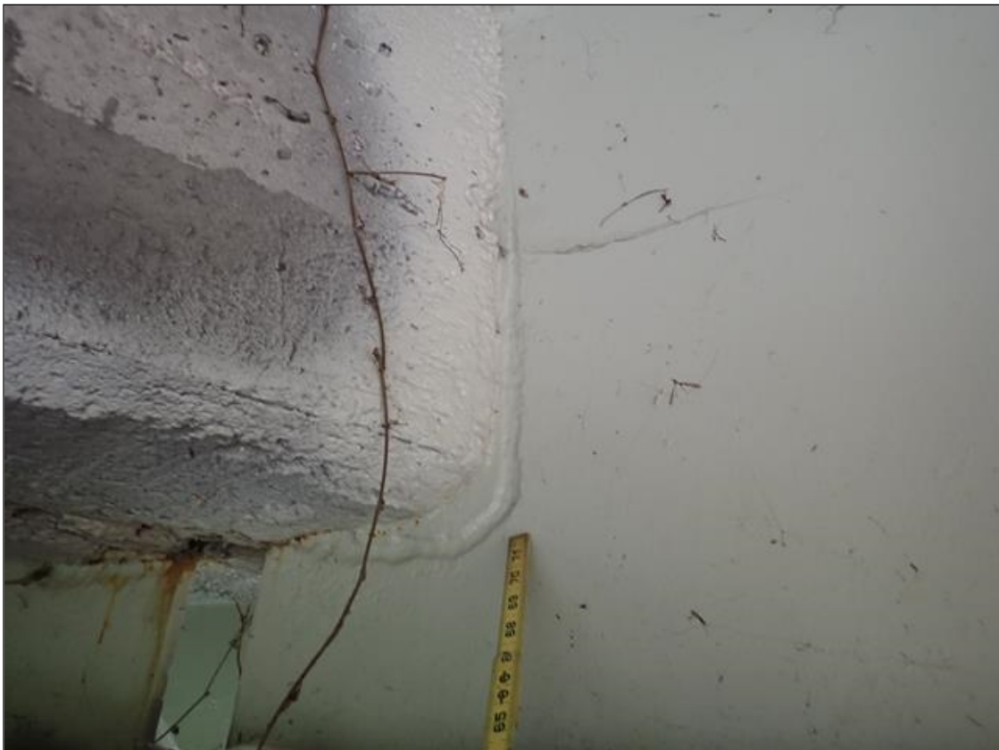
Span 7 Beam 3: (PAR) at bent 7, web adjacent to end diaphragm, painted over section loss (7/16 inch average remaining x 7 inch x 1 inch) with corrosion reactivating
