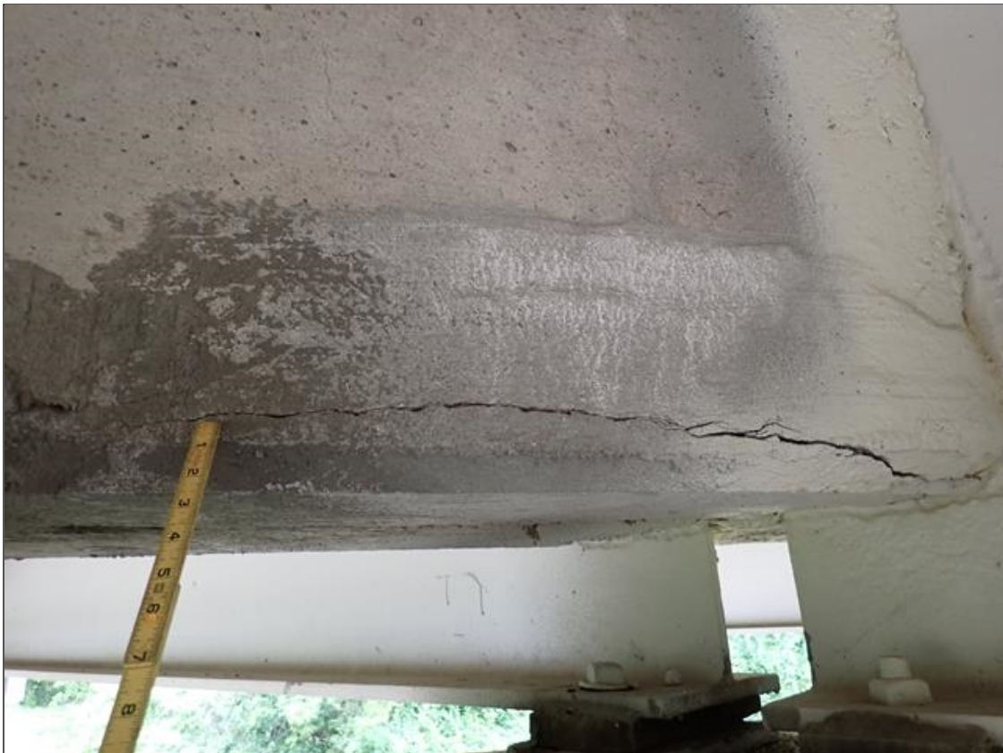
Span 5 Deck: 3 FEET LONG X 11 INCHES HIGH UNSOUND CONCRETE PATCH WITH 1/8 INCH WIDE HORIZONTAL CRACK, BAY 2 END DIAPHRAGM, NEXT TO BEAM 2, AT BENT 4.
