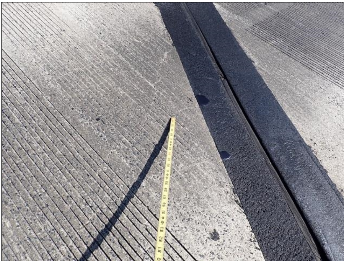
Span 8 Deck: UP TO 0.05 INCH WIDE X 8 FEET LONG DIAGONAL CRACKS EXTENDING FROM EXPANSION JOINT AT END BENT 2.
