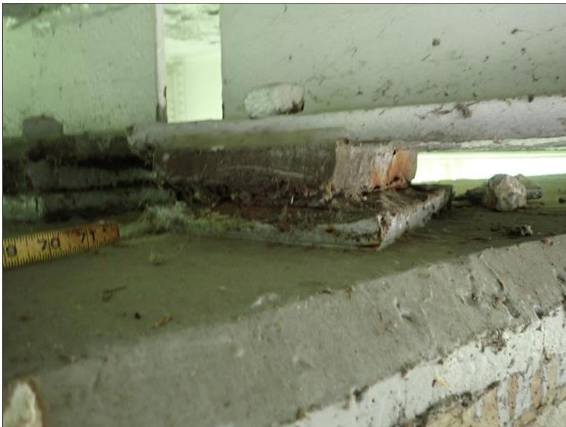
Span 1 Far Bearing 2: painted over section loss (approximately 85 percent remaining) with corrosion reactivating
