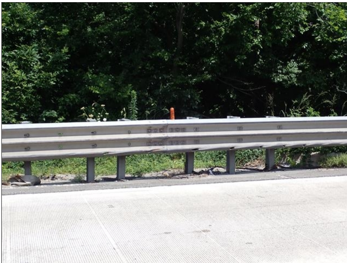
(PAR) southwest guardrail starting at bridge, impact damage (25 foot) with holes (up to 4 inch x 3 inch)
