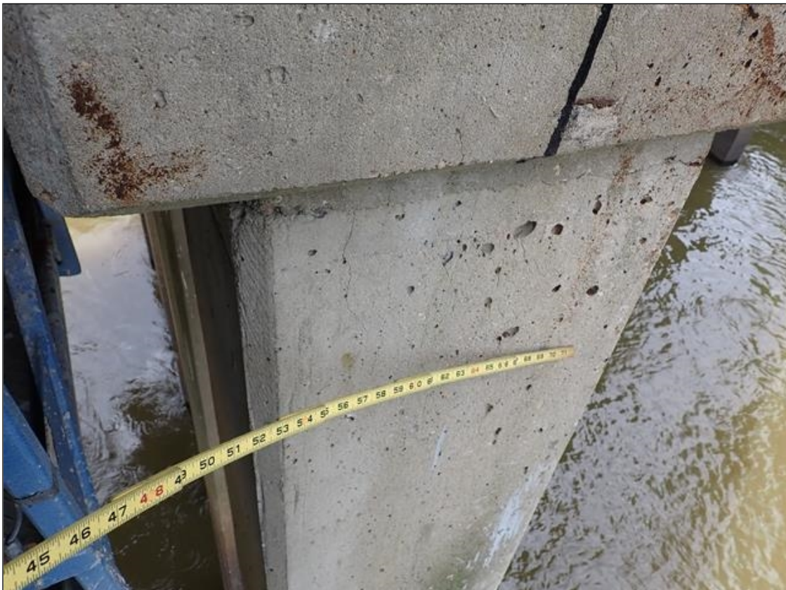
Bent 4 Pile 1: UP TO 5 FEET LONG X 0.02 INCH WIDE VERTICAL CRACKS, IN ALL FACES FACE BEGINNING AT CAP.
