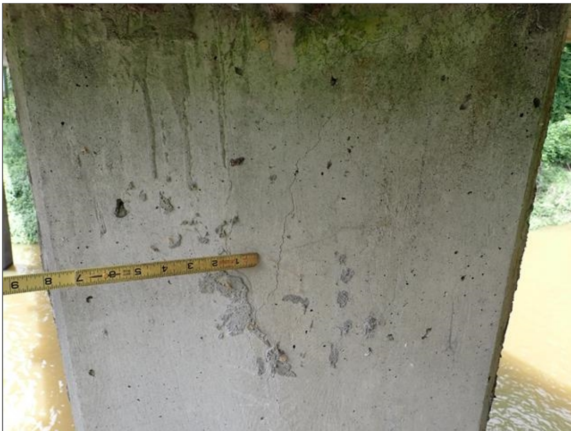
Bent 4 Pile 6: north face near cap, vertical crack (1/32 inch x 28 inch)
