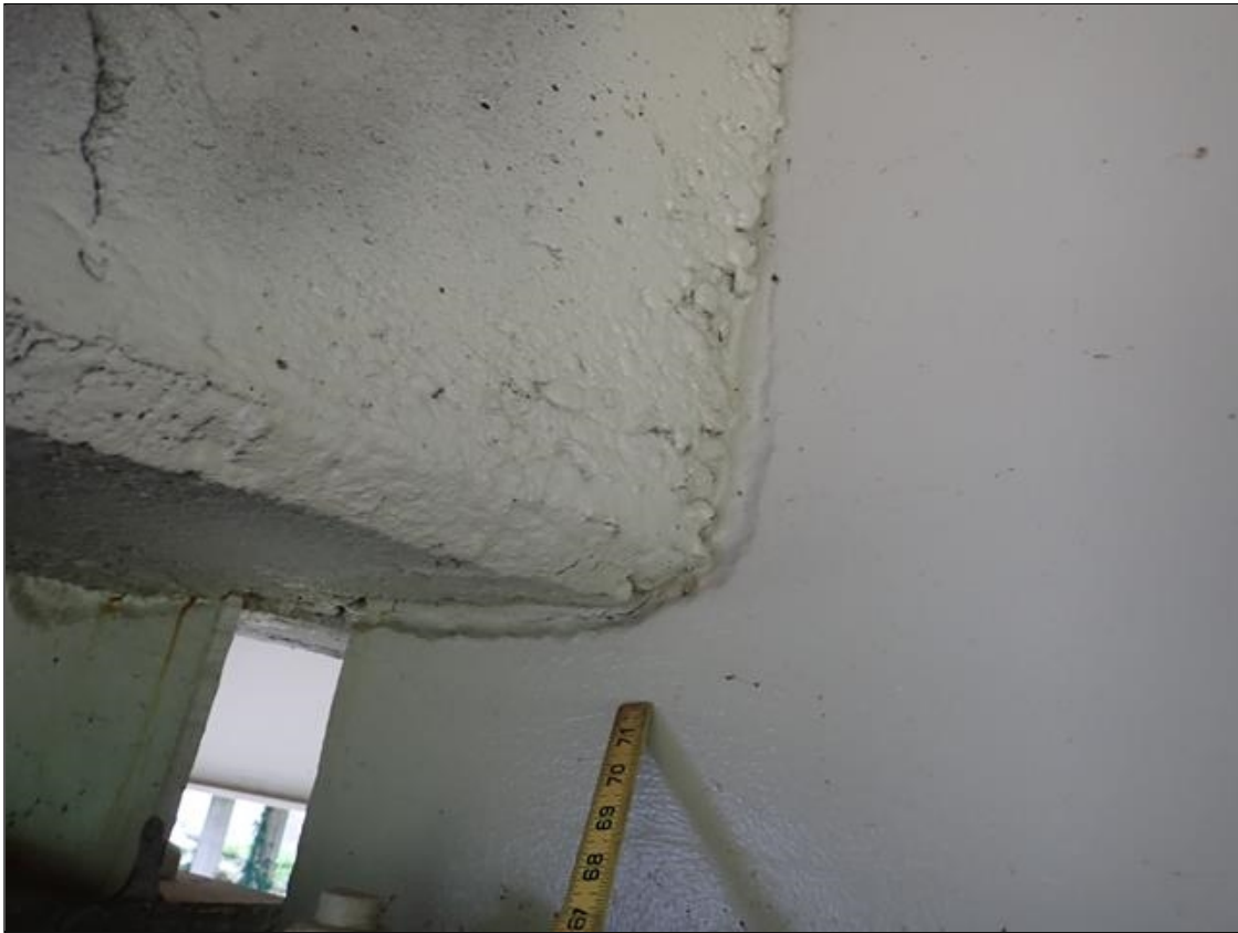
Span 5 Beam 3: (PAR) at bent 5, web adjacent to end diaphragm, painted over section loss (7/16 inch average remaining x 7 inch x 7 inch) with corrosion reactivating
