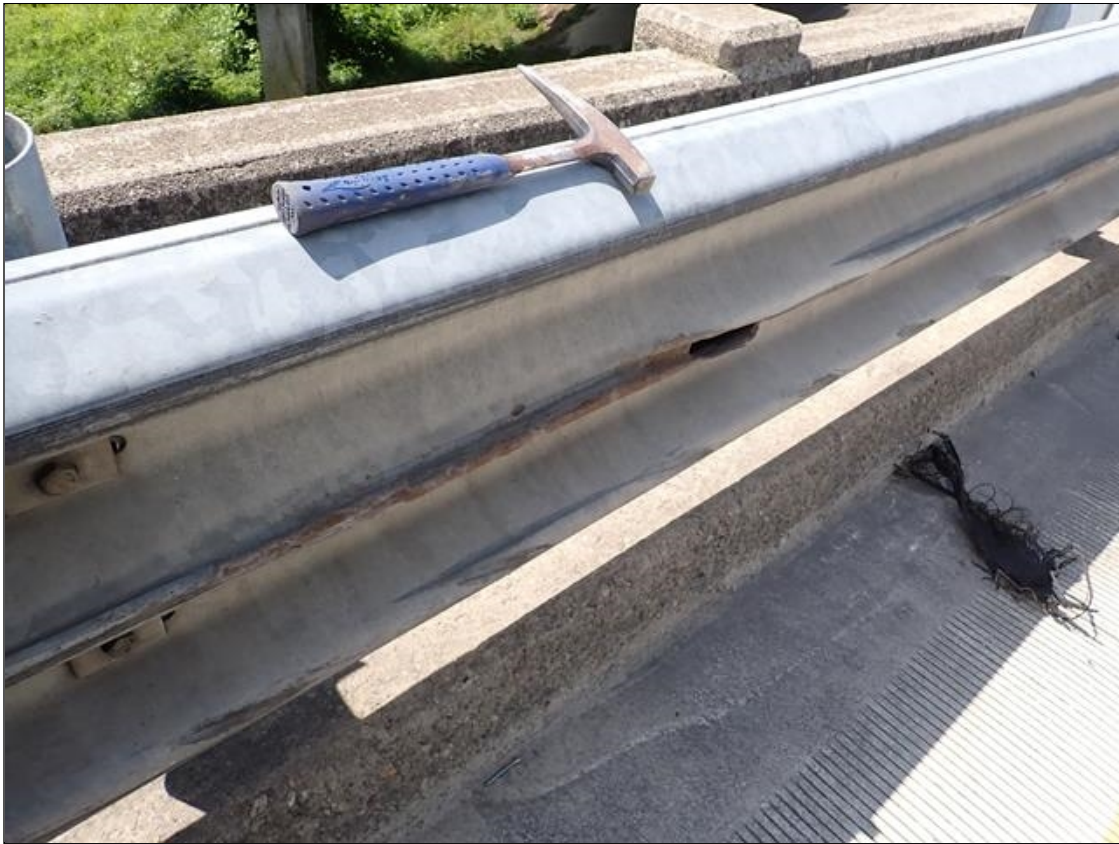
Span 1 Right Retrofit Bridge Rail: (PAR) IMPACT DAMAGE WITH SCRAPE MARKS AND THROUGH HOLES UP TO 4 INCH X 2 INCH IN RETROFIT RAIL AT SCATTERED LOCATIONS
