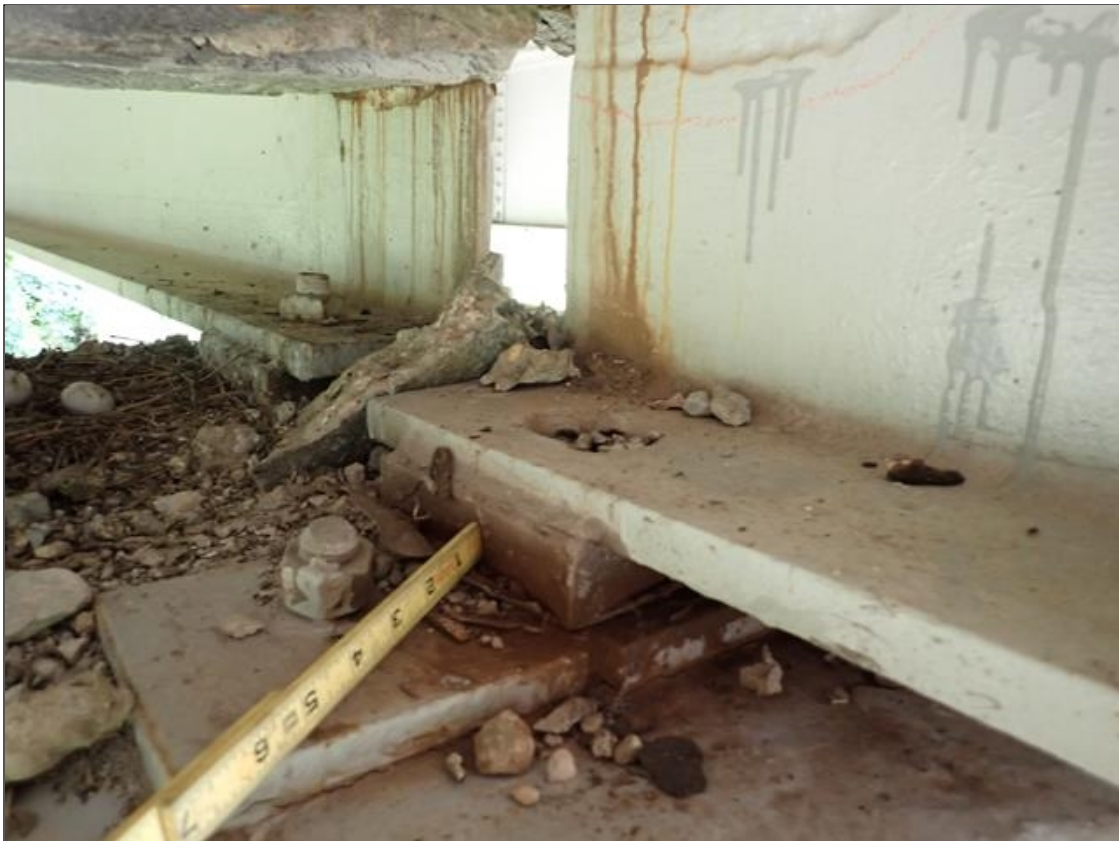
Span 6 Far Bearing 3: BOTH ANCHOR BOLTS, MISSING; BEARING ASSEMBLY HAS WELDED REPAIR WITH NEW ANCHOR BOLT.
