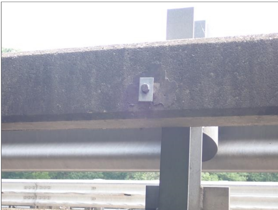
Span 1 Left Bridge Rail: 6 INCH DIAMETER SOUND PATCHES AT ANCHOR BOLT CONNECTIONS TO RETROFIT RAIL
