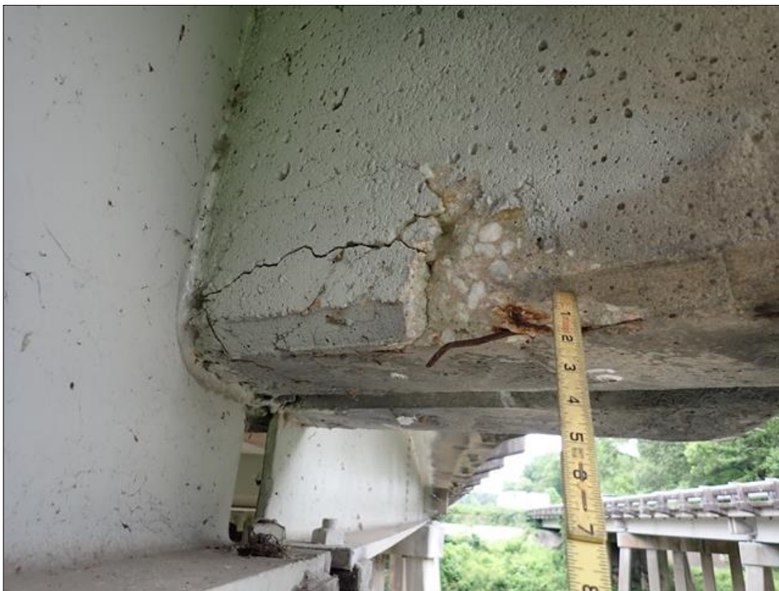
Span 3 Deck: 4 INCHES HIGH X 1 FOOT LONG AREA OF UNSOUND CONCRETE WITH SPALL 4 INCHES DIAMETER X 1 INCH DEEP WITH 1/8 INCH WIDE CRACKS AND EXPOSED STEEL IN END DIAPHRAGM AT BENT 3 UNDER RIGHT OVERHANG.
