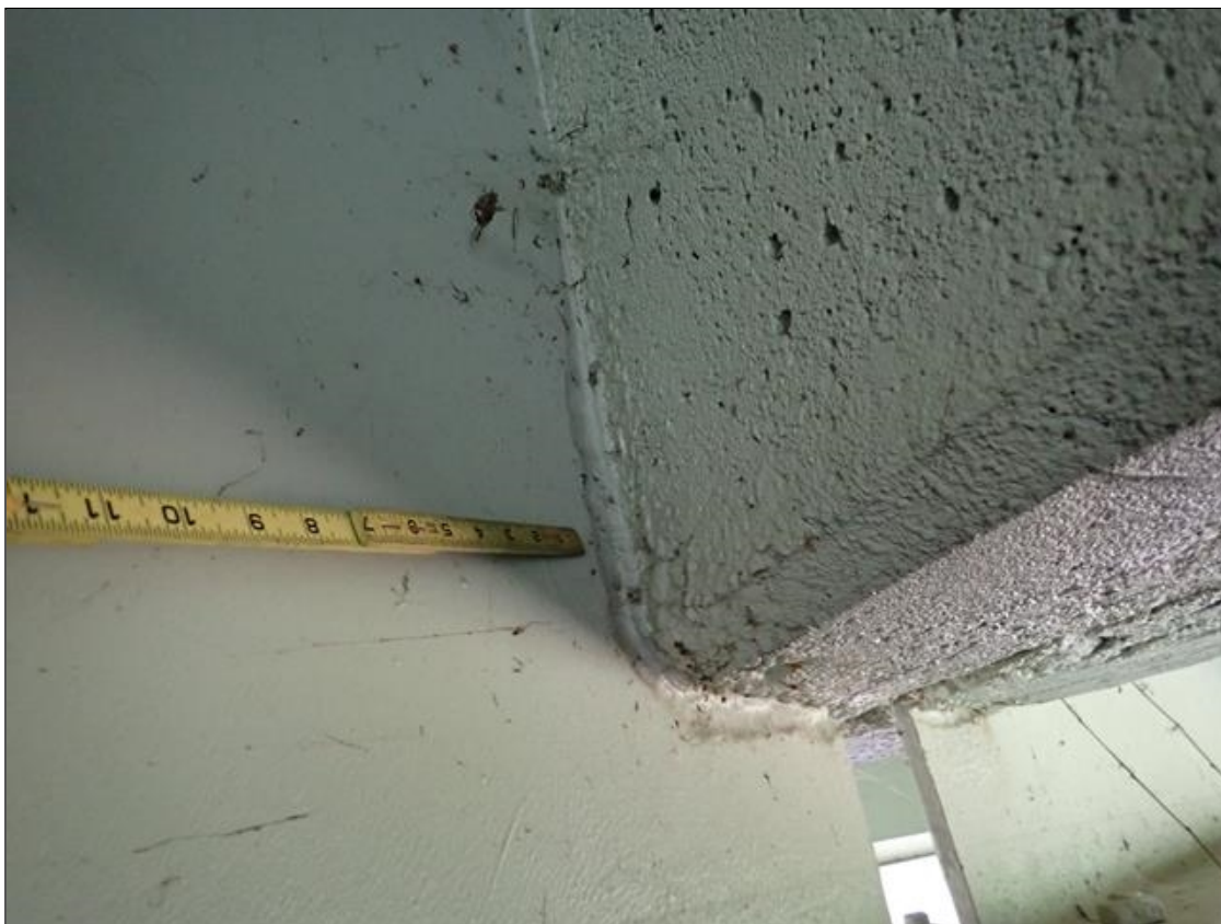
Span 8 Beam 2: (PAR) at bent 7, web adjacent to end diaphragm, painted over section loss (7/16 inch average remaining x 8 inch x 10 inch) with corrosion reactivating
