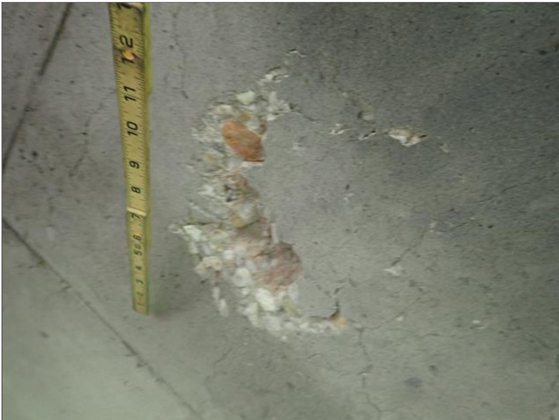
Span 1 Deck: underside of deck in bay 2, adjacent to 1st intermediate diaphragm from end bent 1, spall/delamination (8 inch diameter x 1 inch deep)
