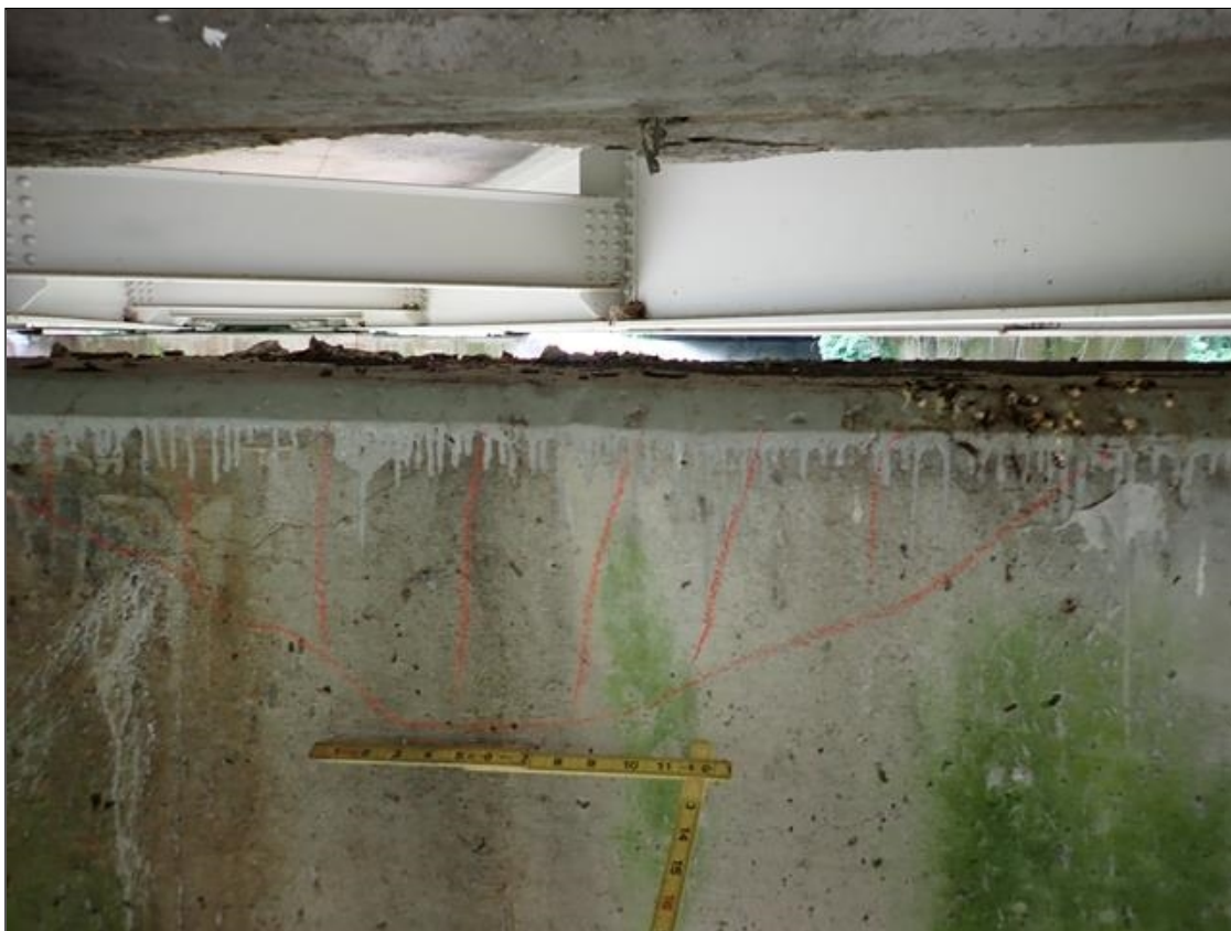
Bent 5 Cap 1: south face in bay 2, delamination (30 inch x 12 inch)
