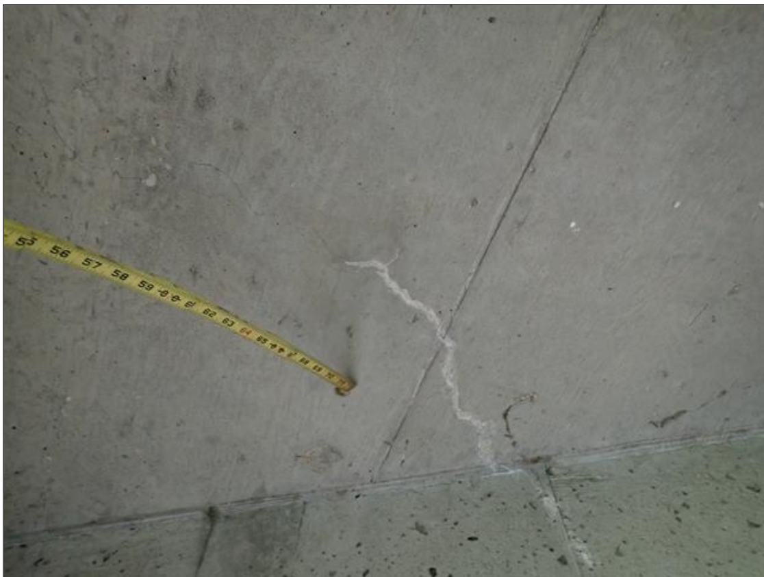
Span 8 Deck: underside of deck, map cracks (up to 1/64 inch) and transverse cracks (up to 1/32 inch x 3 foot) some with efflorescence at random
