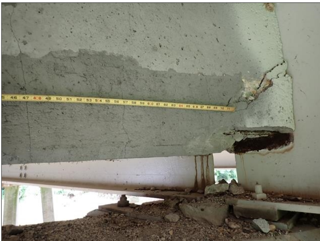
Span 7 Deck: bay 3 end diaphragm at bent 6, failed patch (5 foot x 19 inch x 4 inch deep) with exposed rusted rebar
