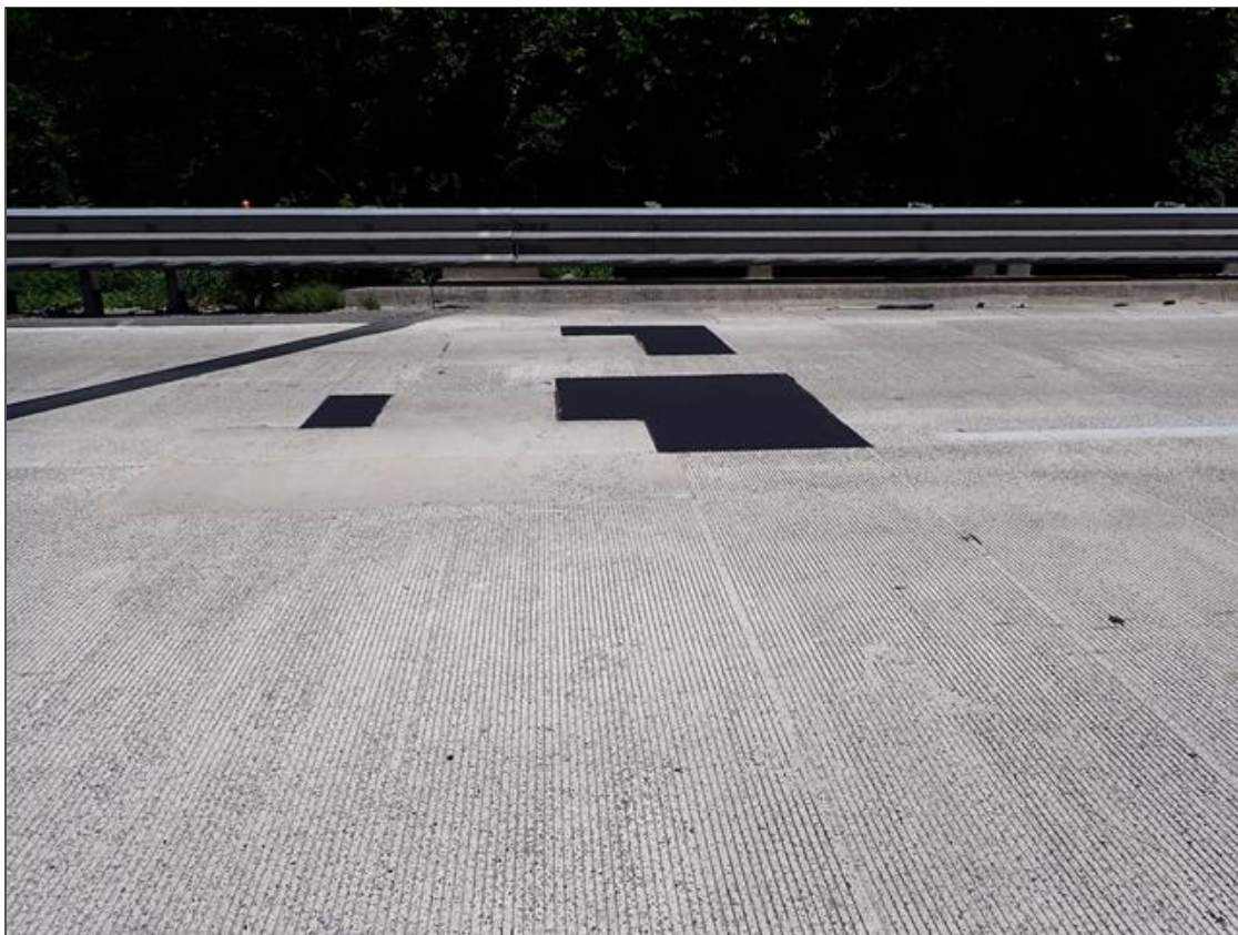
Span 1 Deck: NEAR END BENT 1 IN BOTH LANES PATCHES UP TO 6 FEET X 6 FEET WITH CRACKS (HAIRLINE)
