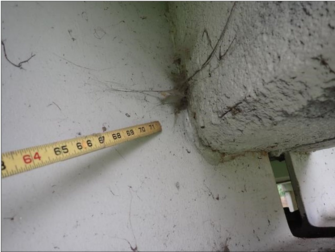
Span 2 Beam 4: (PAR) at bent 2, web adjacent to end diaphragm, painted over section loss (1/2 inch average remaining x 4 inch x 15 inch) with corrosion reactivating
