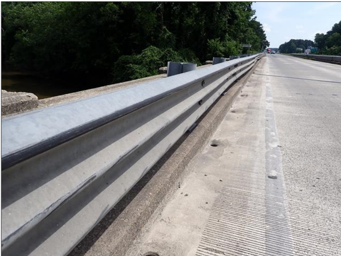
Span 5 Left Retrofit Bridge Rail: (PAR) IMPACT DAMAGE WITH SCRAPE MARKS AND DENTS UP TO 1 INCH DEEP IN RETROFIT RAIL AT SCATTERED LOCATIONS
