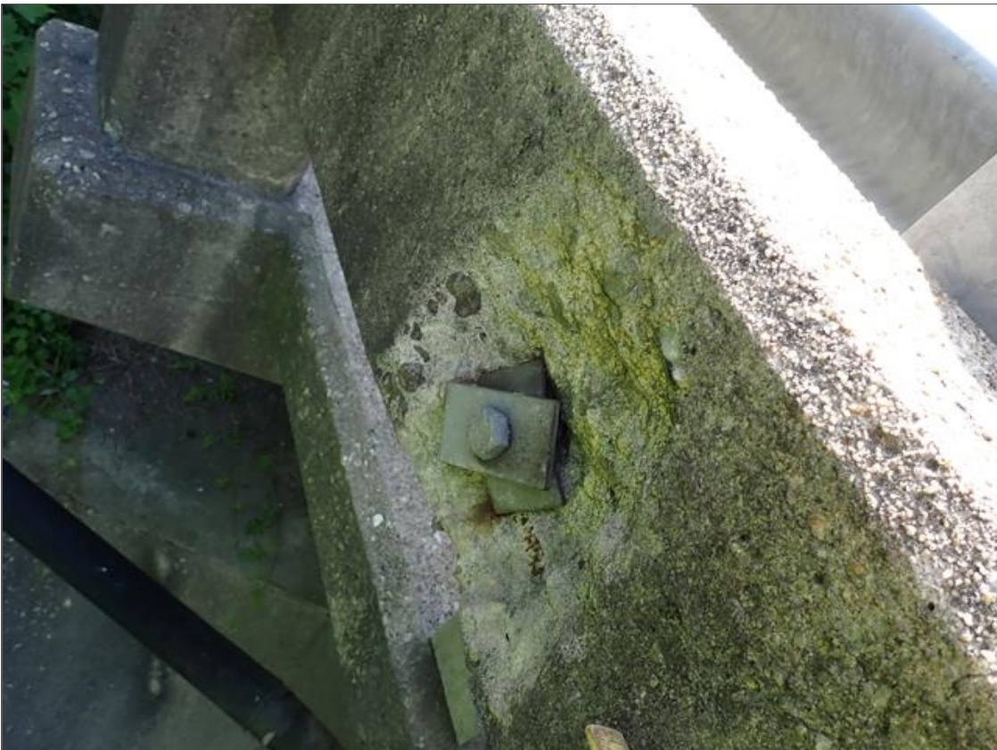
Span 8 Left Bridge Rail: BETWEEN POSTS 7 AND 8 FROM BENT 7, 6 INCH DIAMETER X 1.5 INCH DEEP SPALLS IN EXTERIOR FACE AT ANCHOR BOLT CONNECTION TO RETROFIT RAIL
