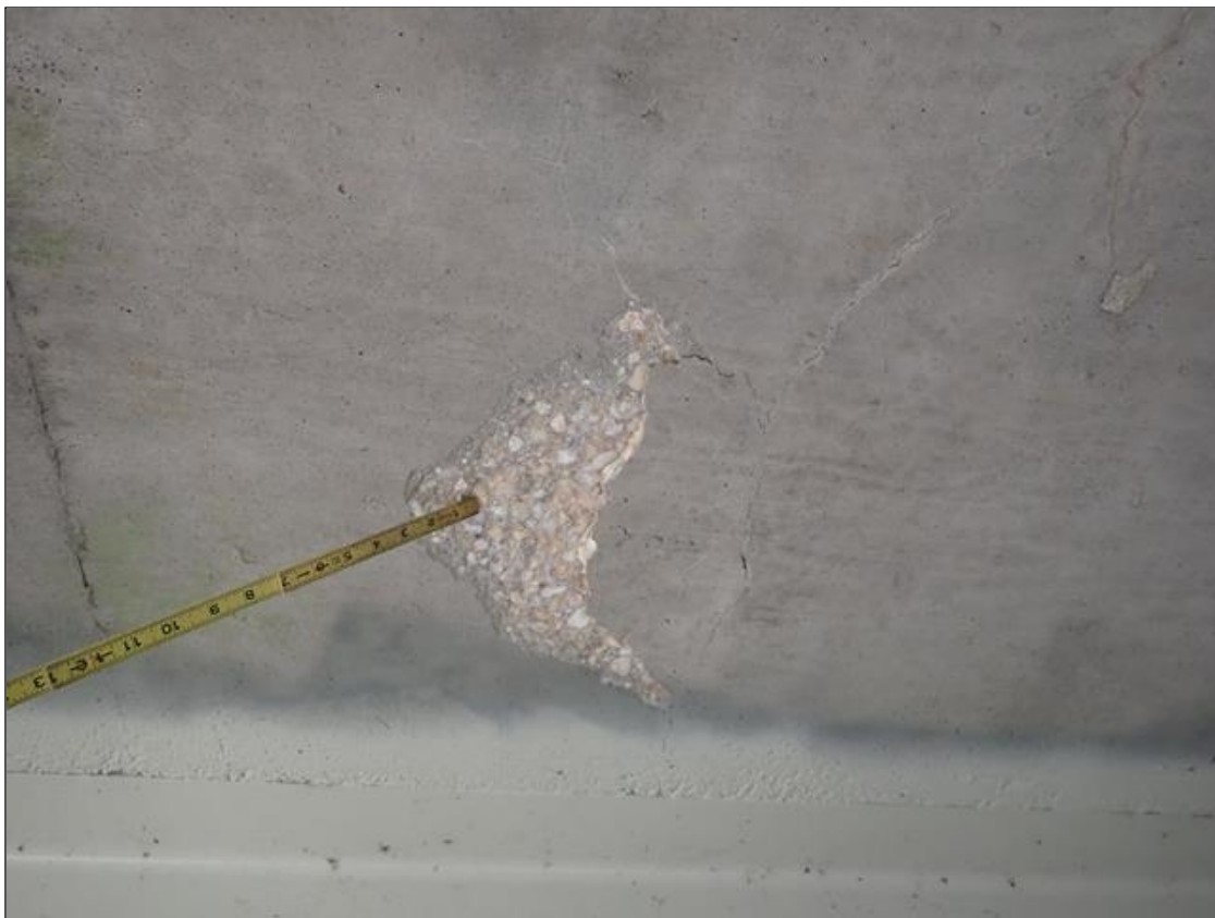
Span 6 Deck: BAY 1 NEAR BENT 6 AREA OF SPALL/DELAMINATION 18 INCHES DIAMETER X 1/2 INCH DEEP.
