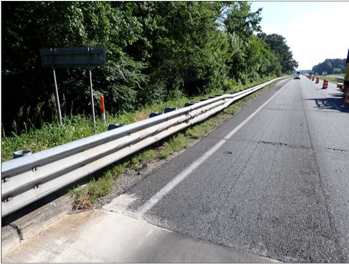
northwest guardrail transition
