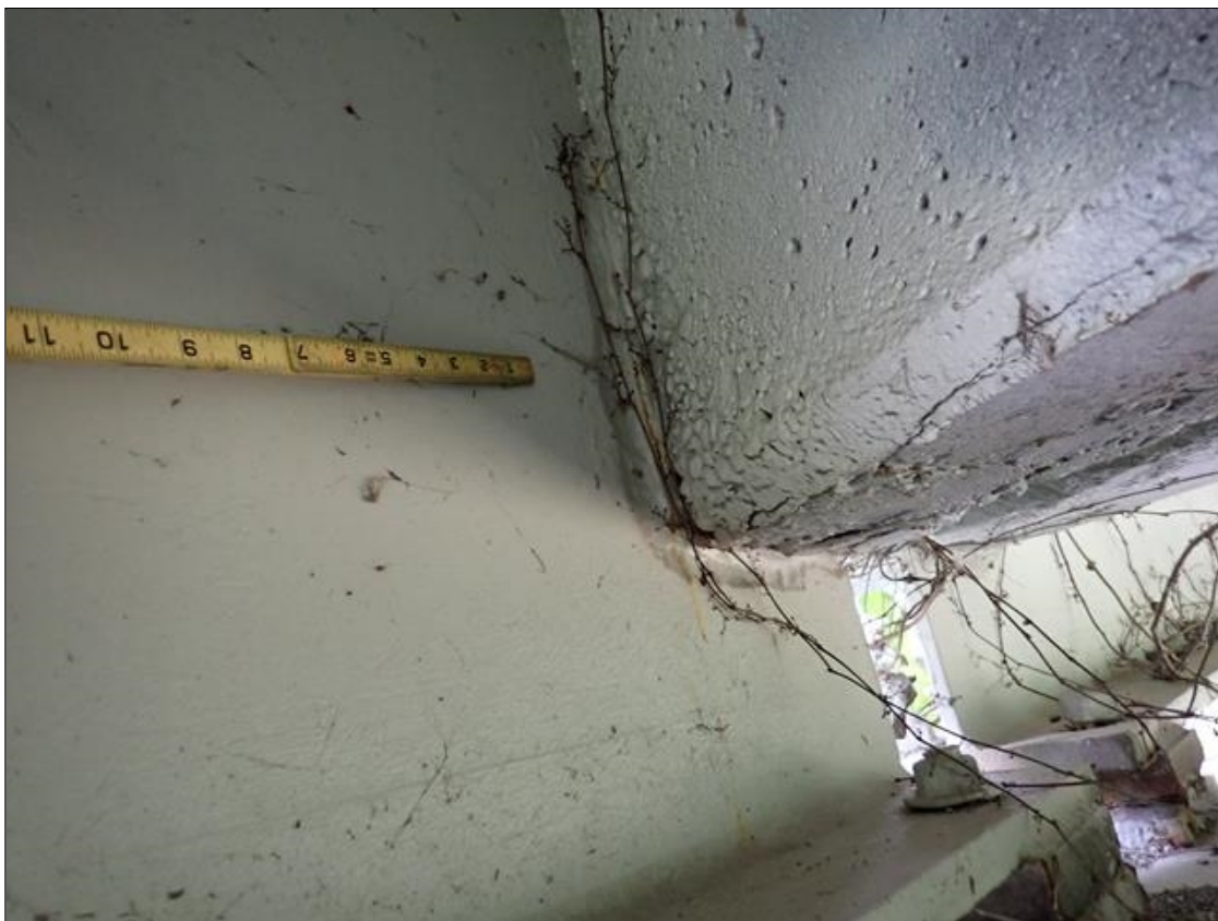
Span 8 Beam 4: (PAR) at bent 7, web adjacent to end diaphragm, painted over section loss (7/16 inch average remaining x 7 inch x 13 inch)
