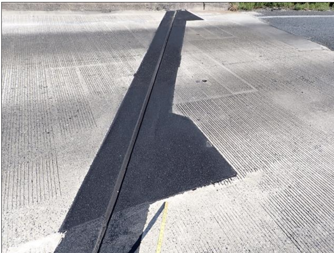
Approach 2: AT SOUTH END BETWEEN LANES AND RIGHT SHOULDER (2) SOUND PATCHES UP TO 2 FEET X 2 FEET.
