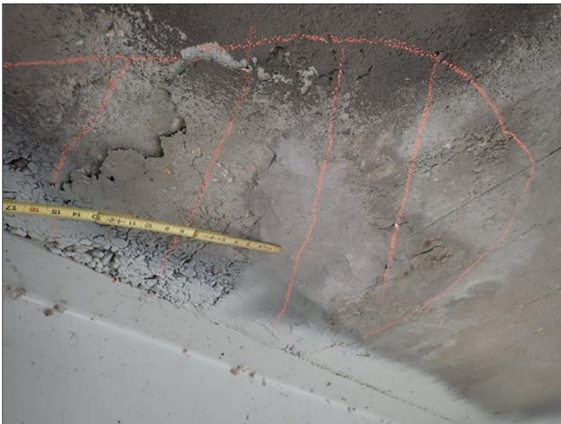
Span 7 Deck: underside in bay 2, near midspan, delamination/failed patch (3 foot x 26 inch)
