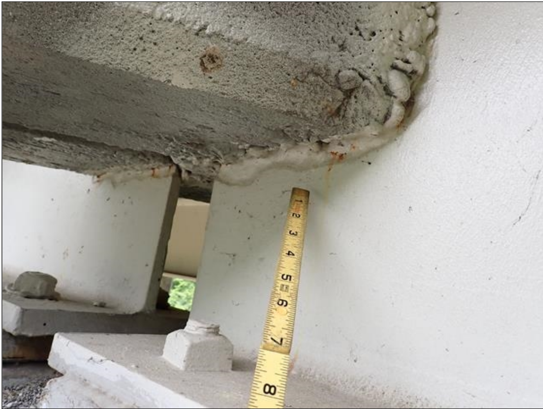
Span 5 Beam 4: (PAR) at bent 4, web adjacent to end diaphragm, painted over section loss (1/2 inch average remaining x 7 inch x 1 inch) with corrosion reactivating
