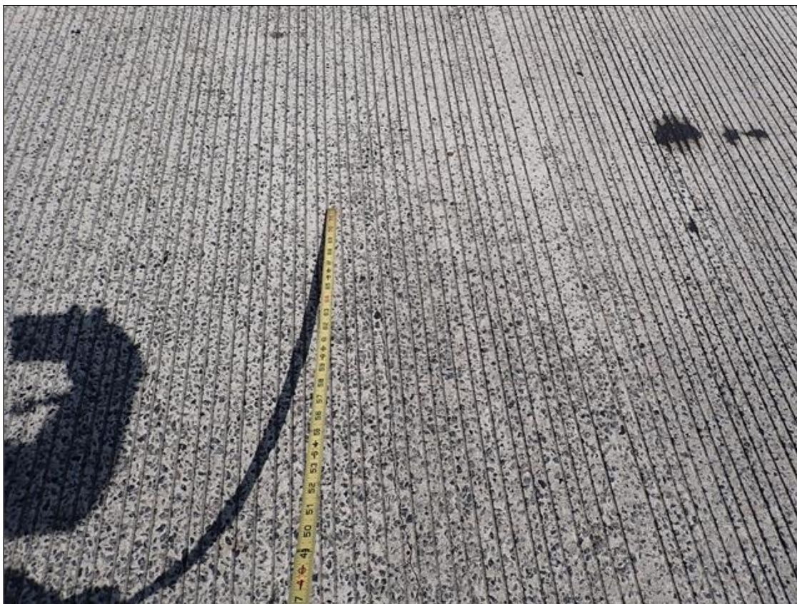
Span 6 Deck: throughout top of deck, longitudinal and transverse cracks (up to 1/32 inch x 16 foot) at random
