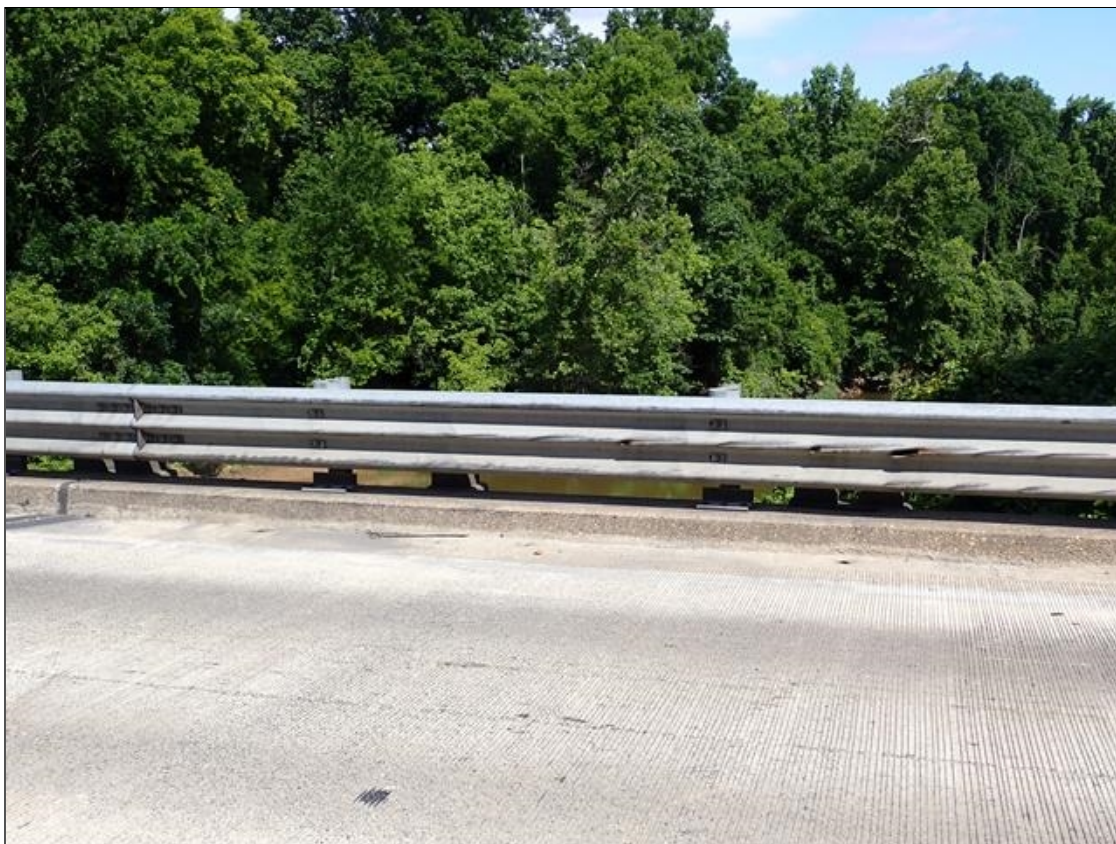
Span 7 Left Retrofit Bridge Rail: (PAR) IMPACT DAMAGE WITH SCRAPE MARKS AND THROUGH HOLES UP TO 4 INCH X 2 INCH IN RETROFIT RAIL AT SCATTERED LOCATIONS
