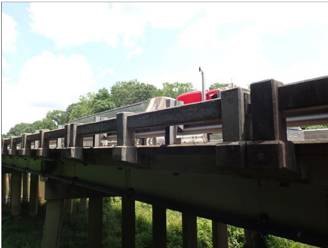
Span 1 Left Bridge Rail: BEGINNING 15 FEET FROM END BENT 1, 15 FEET LONG AREA OF SOUND PATCHING TO RAIL
