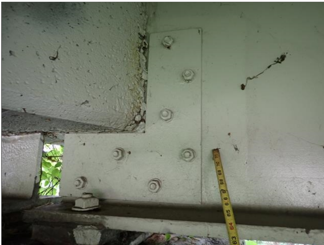
Span 8 Beam 1: at bent 7, web repair plate (1/4 inch thick x 15 inch x 18.5 inch)
