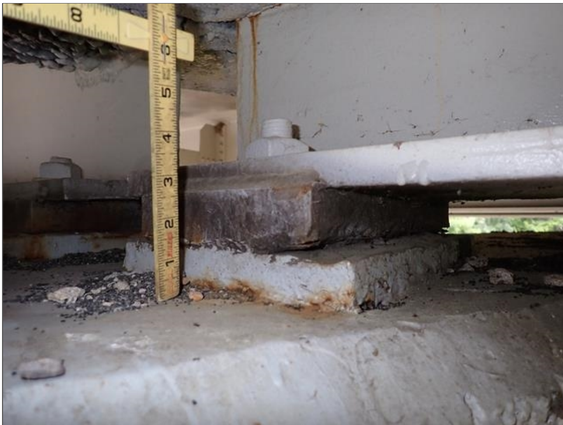
Span 6 Near Bearing 3: painted over section loss (less than 1/16 inch loss)
