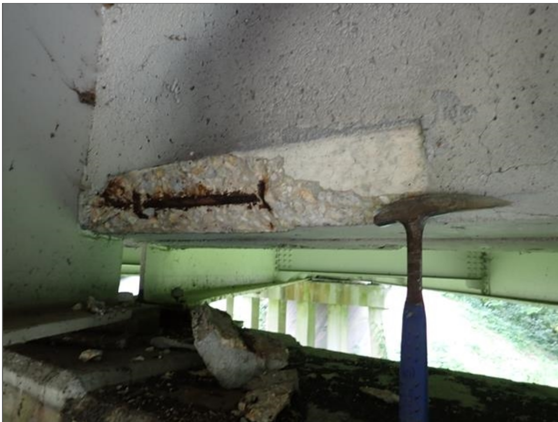
Span 3 Deck: (PAR) BAY 1 NEAR DIAPHRAGM ADJACENT TO BEAM 2, SPALL WITH EXPOSED REBAR 3 FEET X 5 INCHES X 3 INCH DEEP, 5 PERCENT SECTION LOSS.
