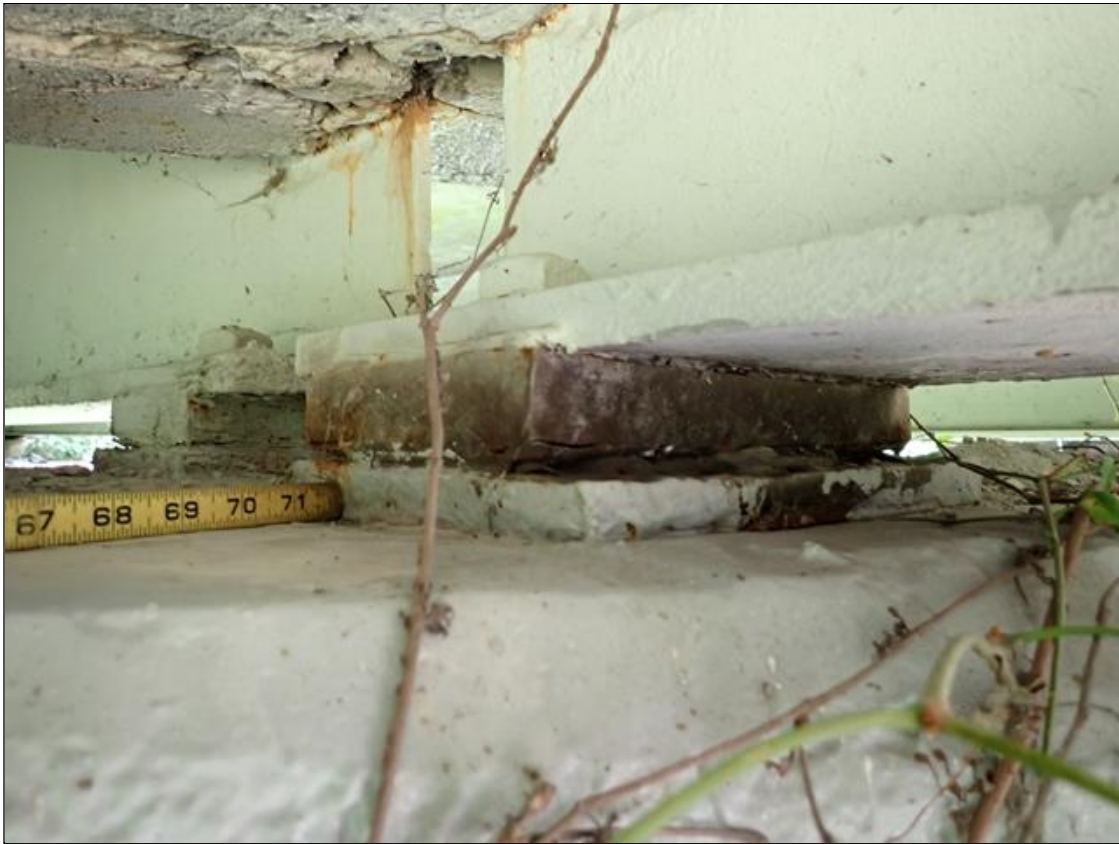
Span 7 Beam 3 - Farr Bearing 3: painted over section loss (less than 1/16 inch loss)
