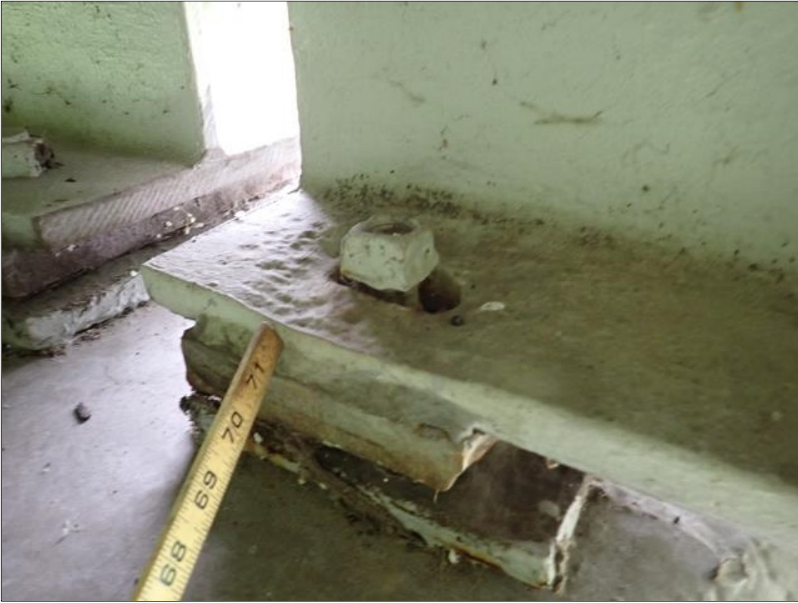
Span 1 Beam 4: (PAR) at bent 1, painted over section loss: web adjacent to end diaphragm (7/16 inch average remaining x 8 inch x 24 inch); bottom flange (0.87 inch average remaining x 5 inch)
