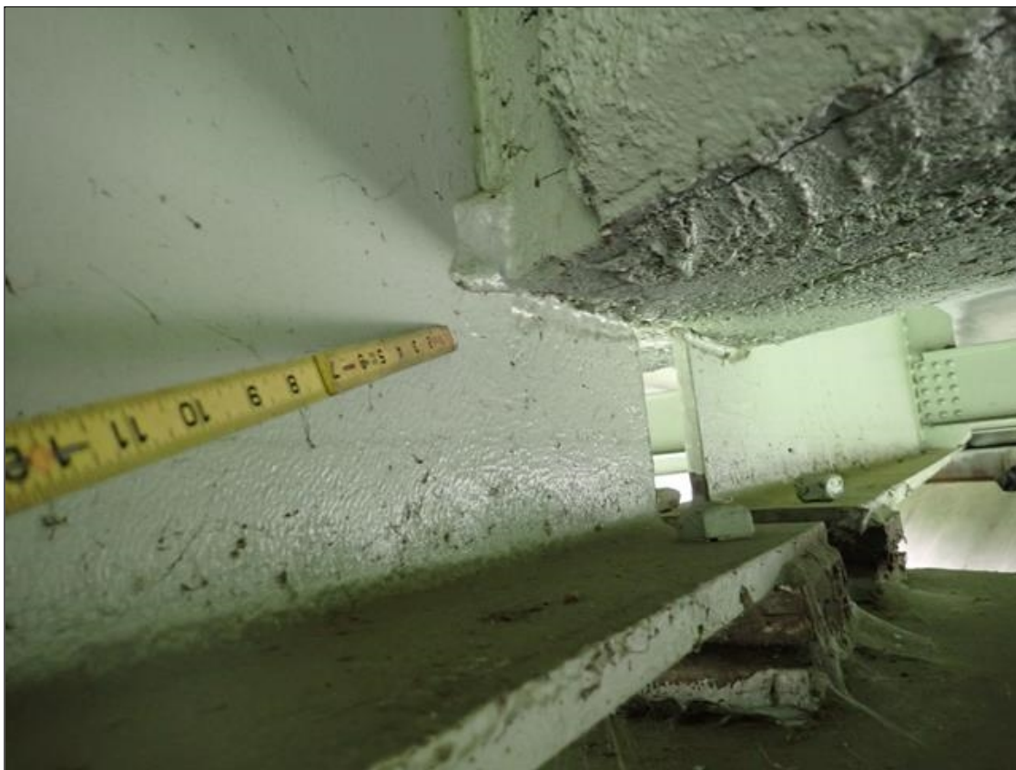
Span 2 Beam 2: (PAR) at bent 1, web adjacent to end diaphragm, painted over section loss (1/2 inch average remaining x 1 inch x 7 inch) with corrosion reactivating
