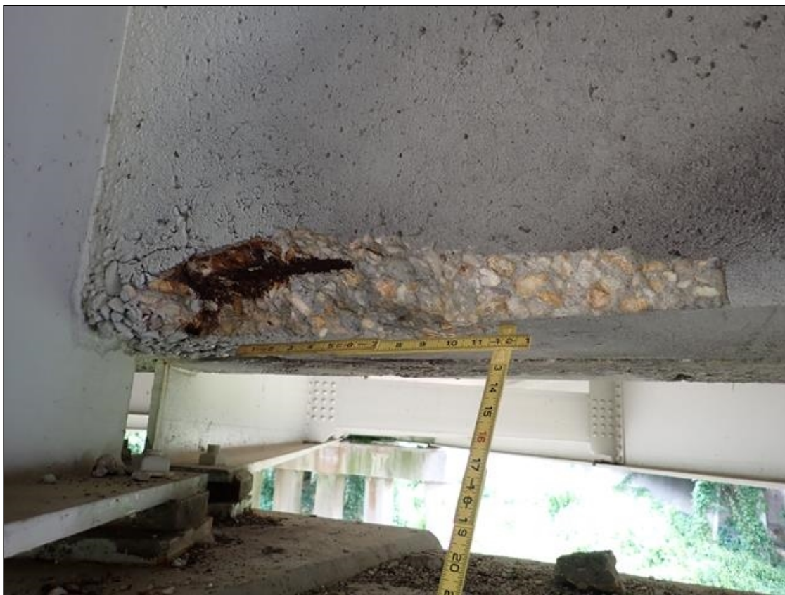
Span 5 Deck: (PAR) BAY 3 FAR DIAPHRAGM ADJACENT TO BEAM 3 AREA OF SPALLING AND DELAMINATION 2 FEET X 4 INCHES X UP TO 3 INCHES DEEP WITH EXPOSED RUSTED REBAR (APPROXIMATELY 80 PERCENT REMAINING)
