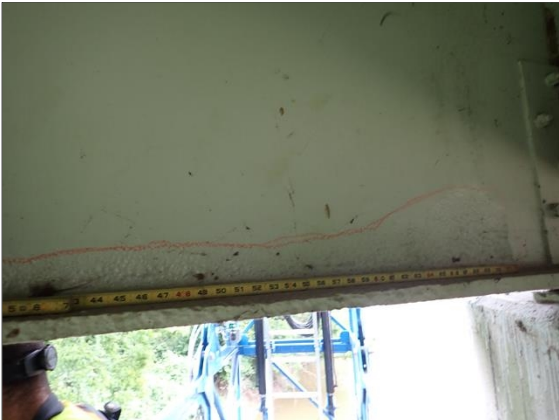
Span 3 Beam 1: (PAR) at bent 3, 2 foot from beam end, painted over section loss: lower web (1/2 inch average remaining remaining x 40 inch x 10 inch); bottom flange (0.87 inch x 40 inch)
