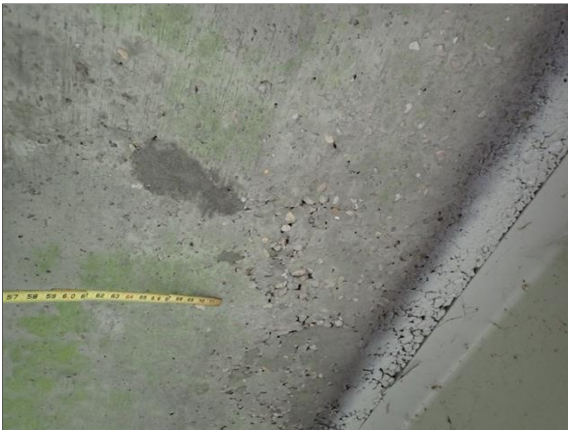
Span 8 Deck: throughout underside, areas of honeycomb (up to 7 foot x 3 foot x 1/2 inch deep)
