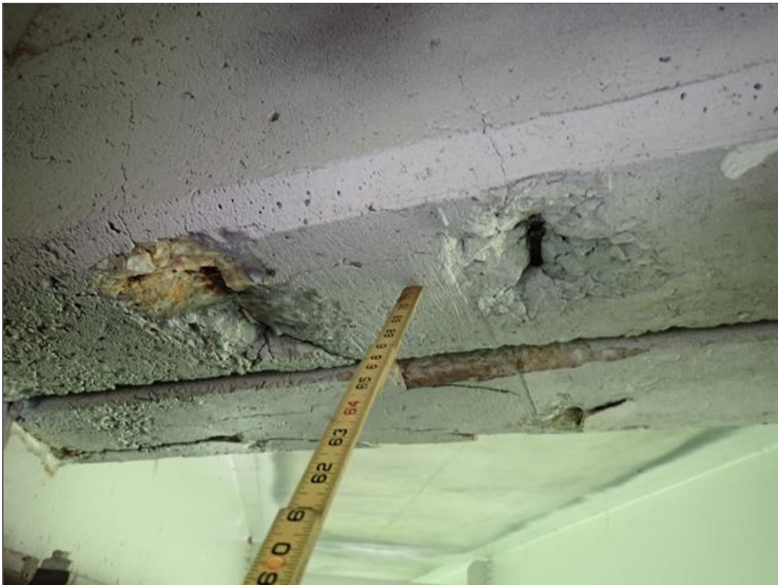
Span 1 Deck: (PAR) TWO (2) UP TO 8 INCHES DIAMETER X 3/4 INCH DEEP SPALLS WITH EXPOSED REBAR, 5 PERCENT SECTION LOSS, UNDERSIDE OF BAY 1 END DIAPHRAGM, AT BENT 1.
