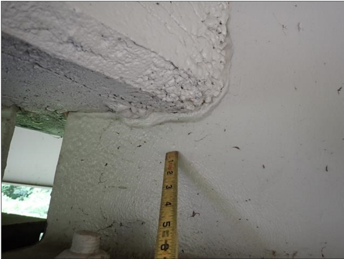
Span 4 Beam 2: (PAR) at bent 3, web adjacent to end diaphragm, painted over section loss (1/2 inch average remaining x 8 inch x 4 inch) with corrosion reactivating
