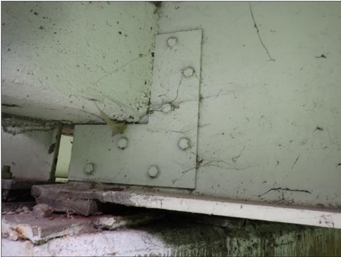
Span 2 Beam 1: 2025 new repair (3/8 inch thick x 15.5 inch x 18 inch), previously noted as: 10 INCHES LONG X 5 INCHES WIDE AREA OF SECTION LOSS BENEATH THE PAINTED SURFACE ABOVE THE BEARING AT BENT 2. 0.60 INCH SECTION REMAINING.
