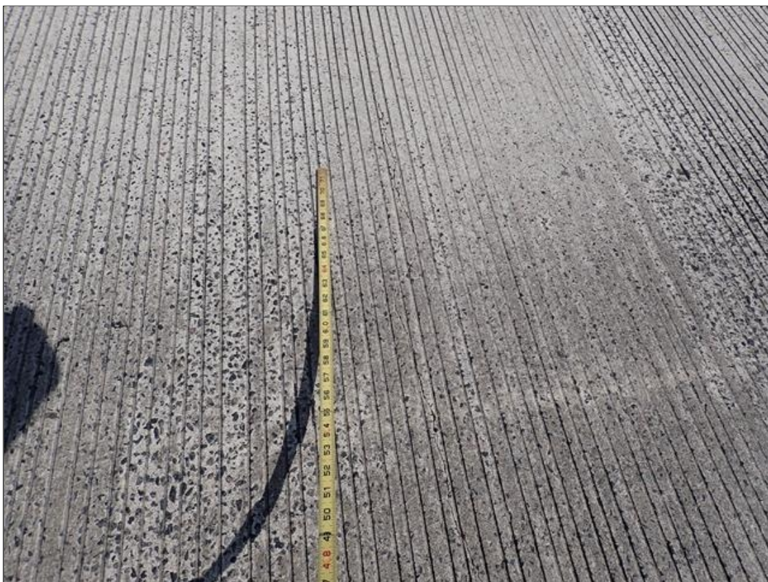
Span 7 Deck: throughout top of deck, longitudinal and transverse cracks (up to 1/32 inch x 16 foot) at random
