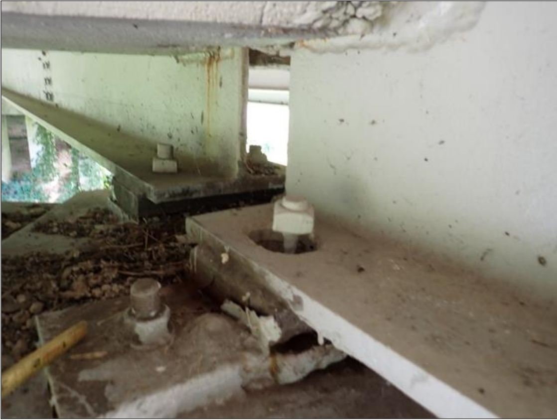
Span 6 Far Bearing 2: LEFT ANCHOR BOLT, PAINTED OVER SECTION LOSS (APPROXIMATELY 40 PERCENT REMAINING; BEARING ASSEMBLY HAS WELDED REPAIR WITH NEW ANCHOR BOLT.
