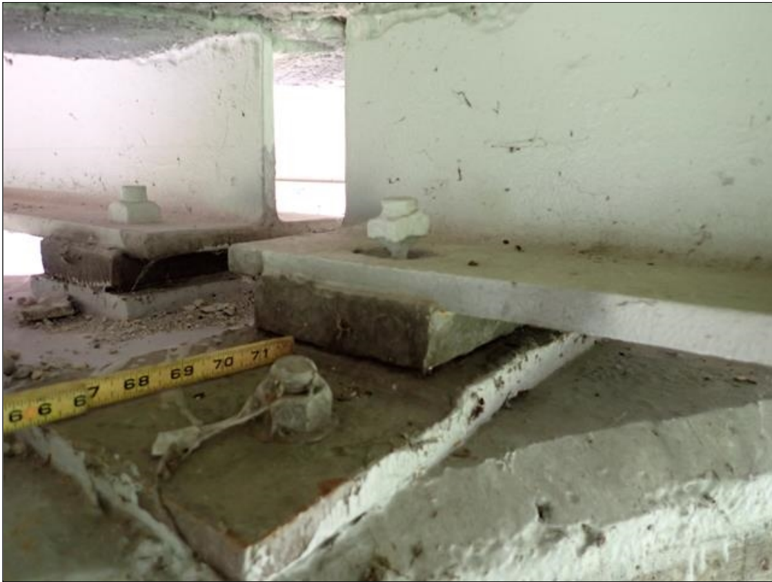
Span 3 Far Bearing 3: LEFT ANCHOR BOLT, PAINTED OVER SECTION LOSS (APPROXIMATELY 20 PERCENT REMAINING); WELDED REPAIR WITH NEW ANCHOR BOLT.
