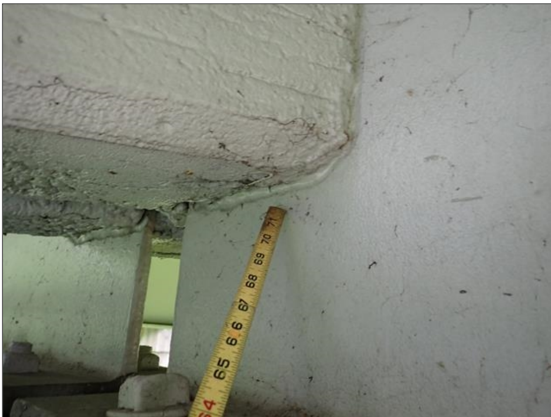
Span 1 Beam 1: at bent 1, web adjacent to end diaphragm, painted over section loss (9/16 inch average remaining x 7 inch x 16 inch) with corrosion reactivating
