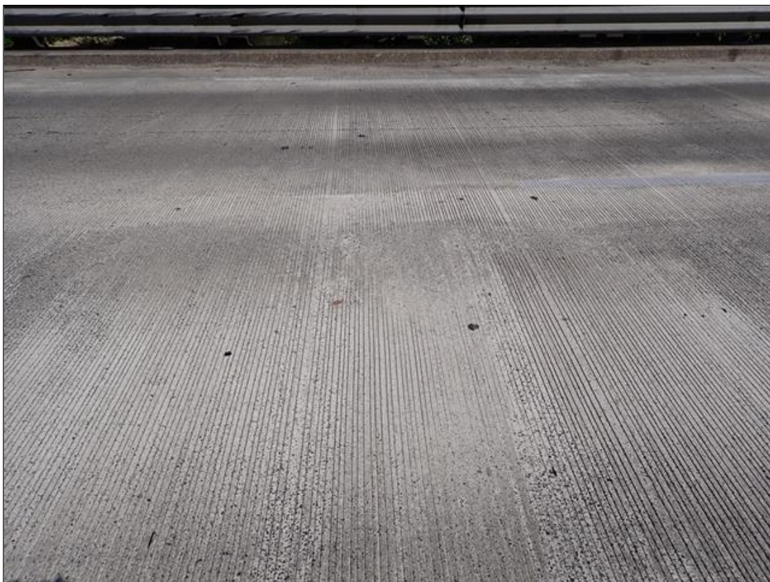
Span 7 Deck: throughout top of deck, wear with secure aggregate at random
