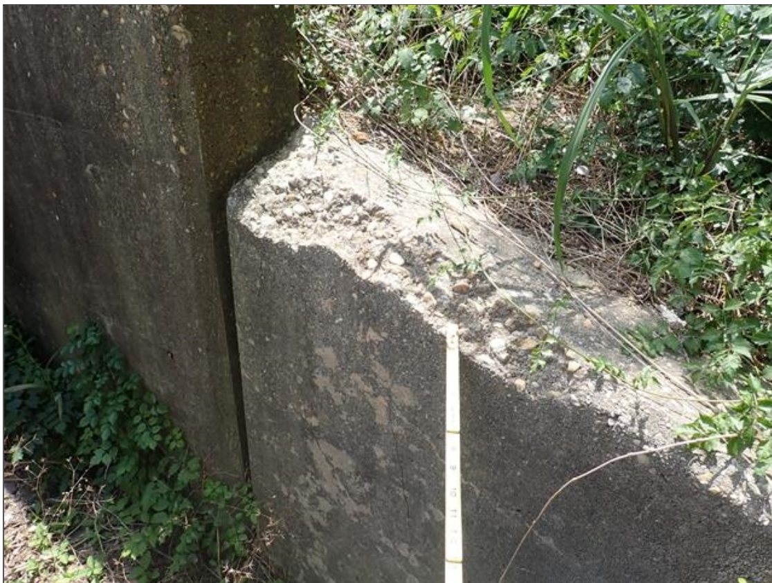
southwest wingwall extension, spall (28 inch x 10 inch x 2 inch deep)
