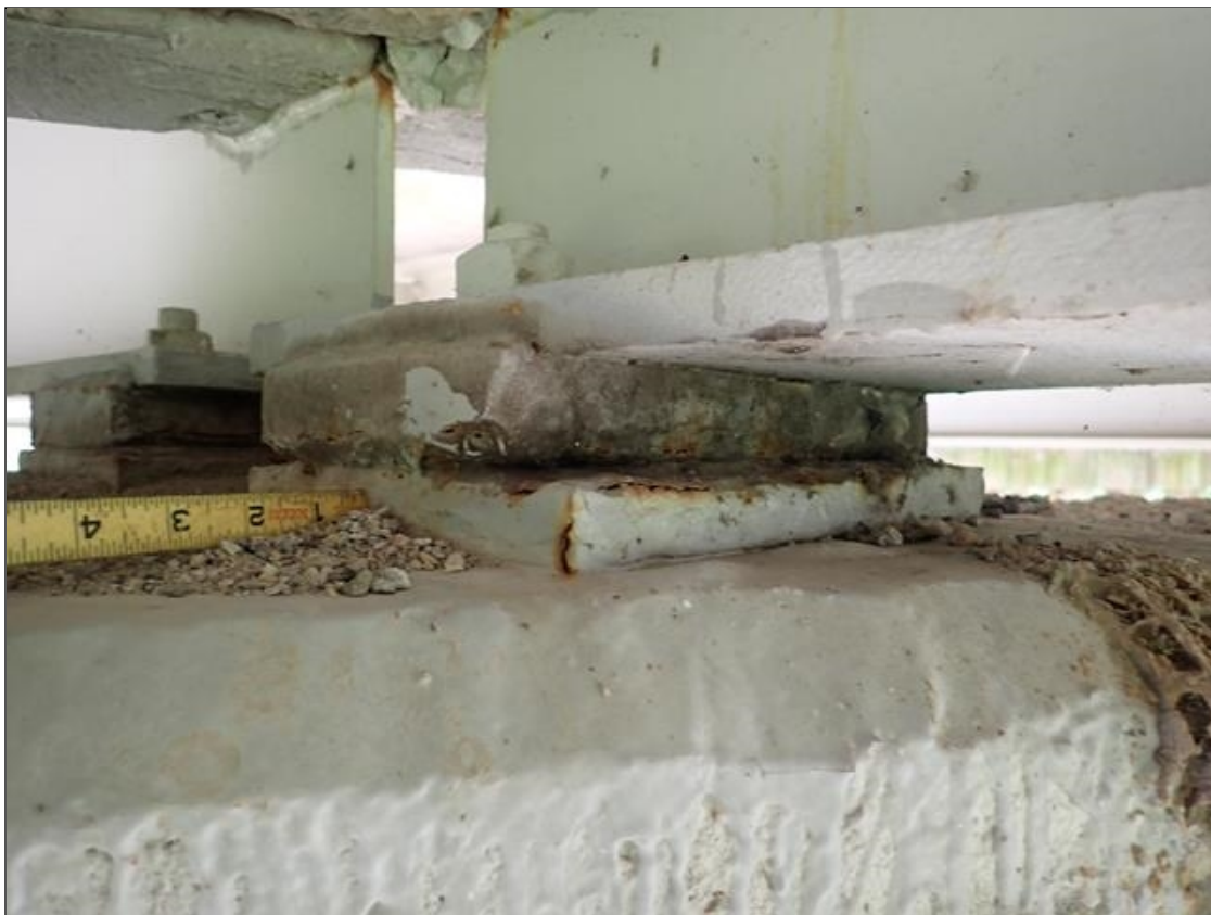
Span 4 Far Bearing 3: painted over section loss (less than 1/16 inch loss) with corrosion reactivating
