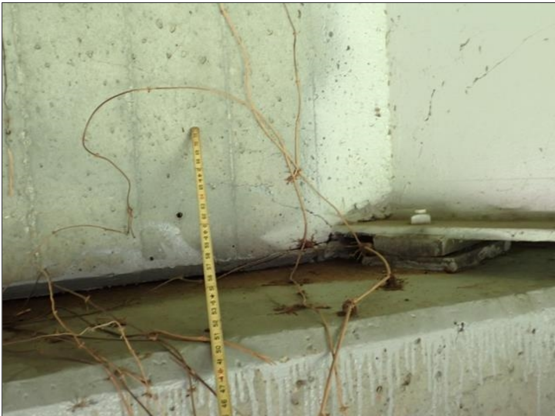
End Bent 1 Abutment: UP TO 1/16 INCH WIDE X 2 FEET LONG DIAGONAL CRACKS EXTENDING FROM BEARING AT ALL BEAMS.
