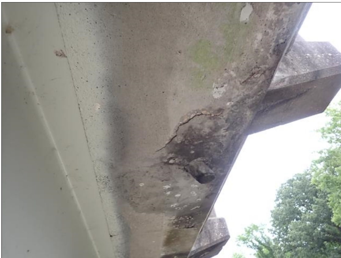
Span 6 Deck: 12 INCHES DIAMETER SOUND CONCRETE PATCH WITH ADJACENT DELAMINATION (18 INCH X 18 INCH) AT 2ND DRAIN PIPE IN EAST OVERHANG.
