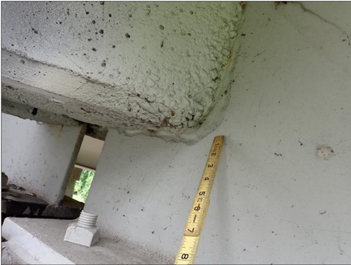
Span 7 Beam 4: (PAR) at bent 6, web adjacent to end diaphragm, painted over section loss (7/16 inch average remaining x 7 inch x 7 inch) with corrosion reactivating
