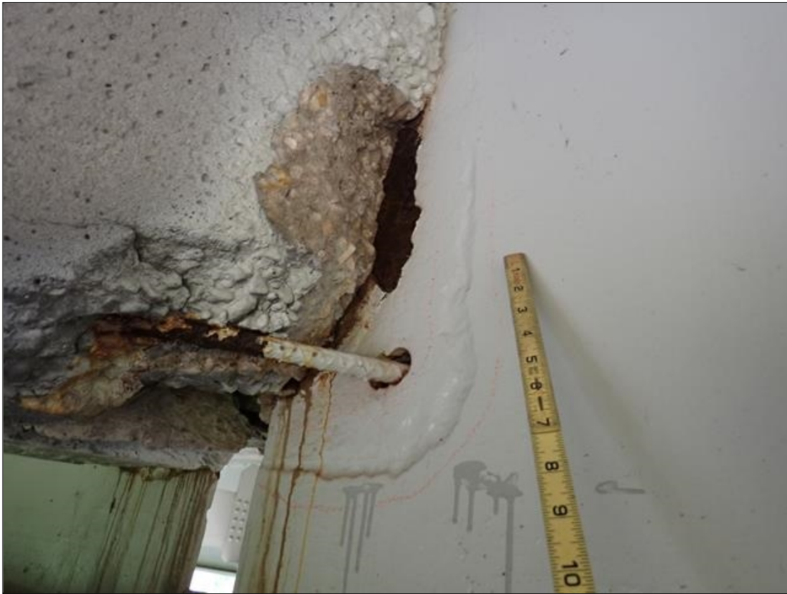
Span 6 Beam 3: (PAR) at bent 6, web adjacent to end diaphragm, corrosion with section loss (7/16 inch average remaining x 10 inch x 2 foot)
