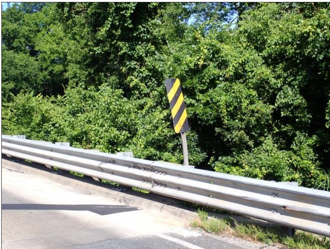
Span 8 Northwest delineator: bent/leaning to the south
