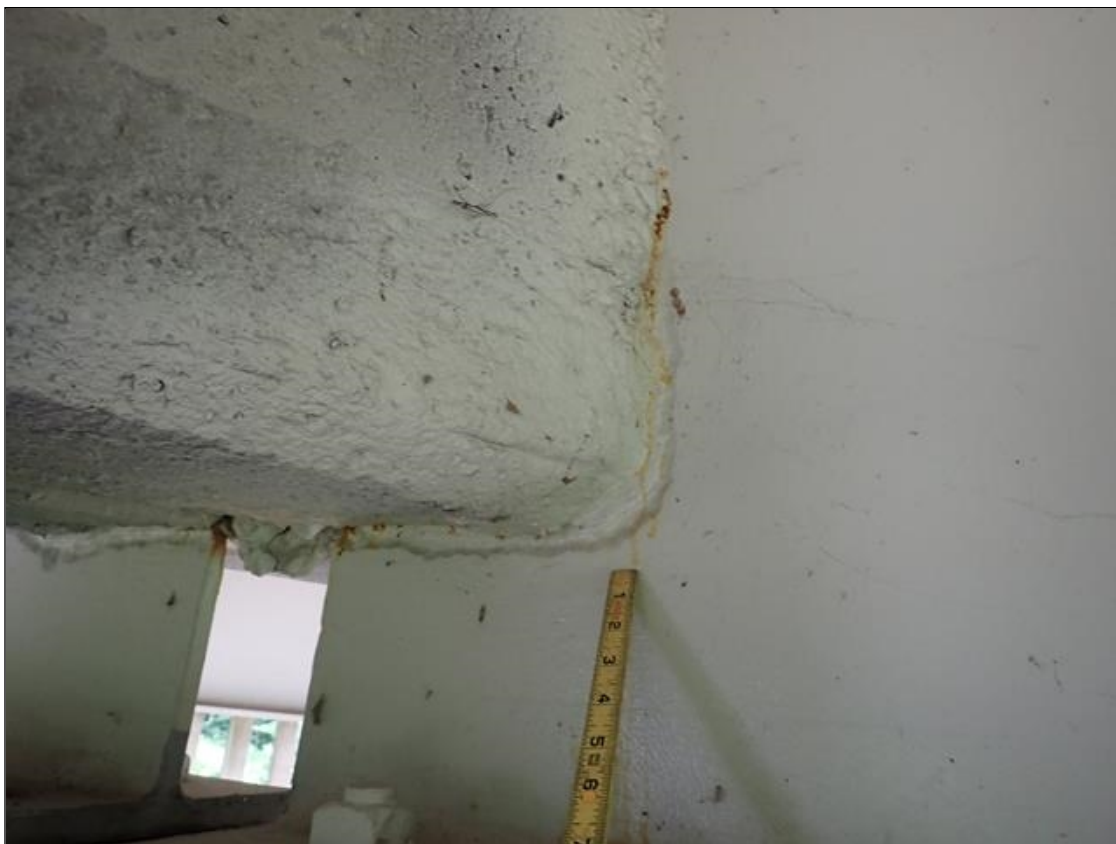
Span 4 Beam 3: (PAR) at bent 4, web adjacent to end diaphragm, painted over section loss (7/16 inch average remaining x 8 inch x 7 inch) with corrosion reactivating
