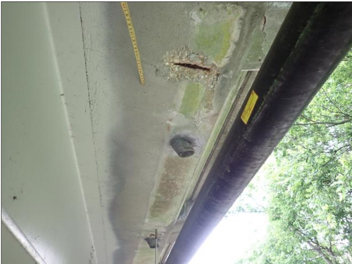
Span 1 Deck: (PAR) UP TO 12 INCHES DIAMETER X 1.5 INCHES DEEP SPALLS WITH EXPOSED REBAR WITH 5 PERCENT SECTION LOSS AT DRAINS 3 AND 4 IN LEFT OVERHANG.
