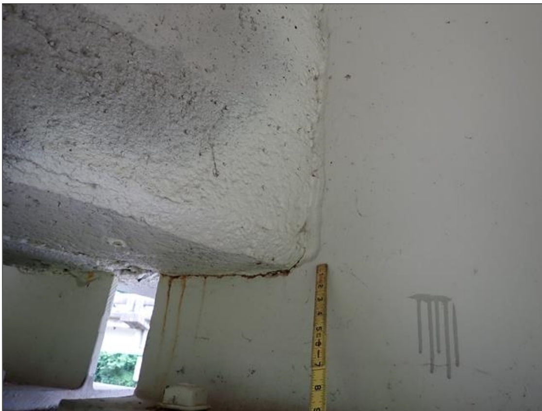
Span 4 Beam 4: (PAR) at bent 4, web adjacent to end diaphragm, painted over section loss (7/16 inch average remaining x 1 inch x 18 inch) with corrosion reactivating
