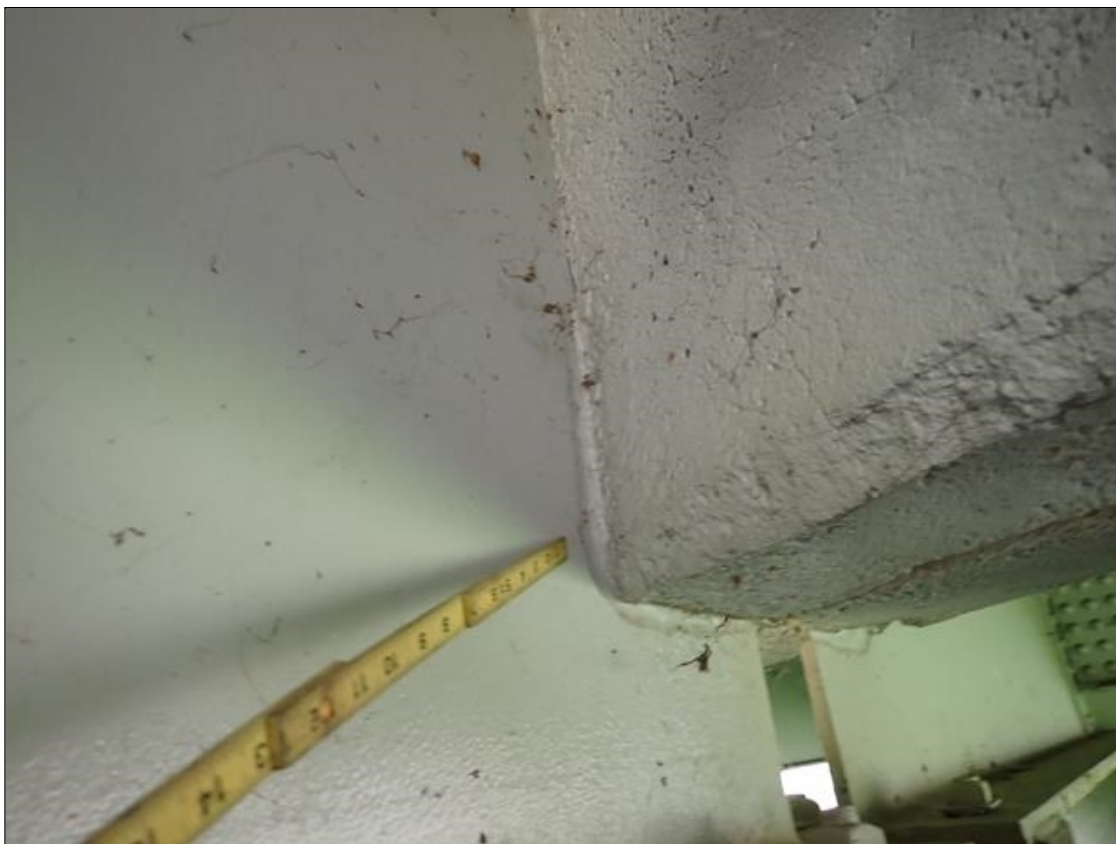
Span 7 Beam 2: (PAR) at bent 7, web adjacent to end diaphragm, painted over section loss (7/16 inch average remaining x 7 inch x 7 inch)
