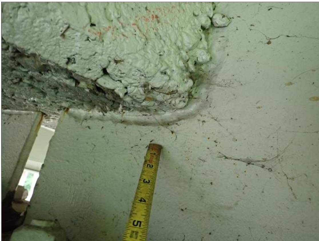
Span 2 Beam 2: (PAR) at bent 2, web adjacent to end diaphragm, painted over section loss (7/16 inch average remaining x 8 inch x 9 inch) with corrosion reactivating
