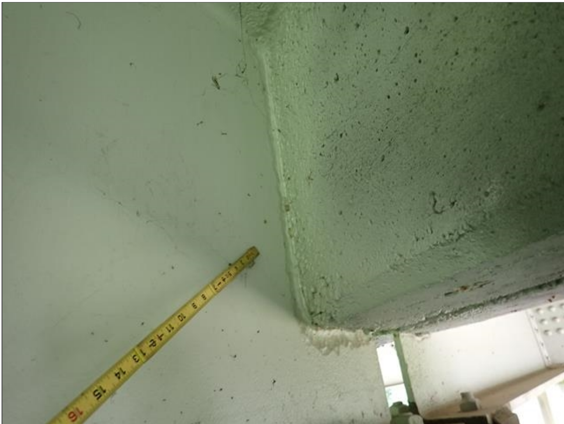
Span 3 Beam 2: (PAR) at bent 3, web adjacent to end diaphragm, painted over section loss (7/16 inch average remaining x 8 inch x 24 inch) with corrosion reactivating
