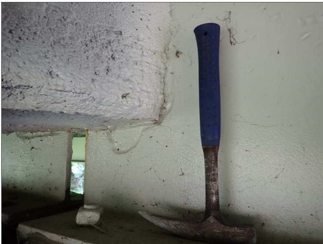
Span 3 Beam 2: (PAR) at bent 2, web adjacent to end diaphragm, painted over section loss (1/2 inch average remaining x 8 inch x 4 inch) with corrosion reactivating
