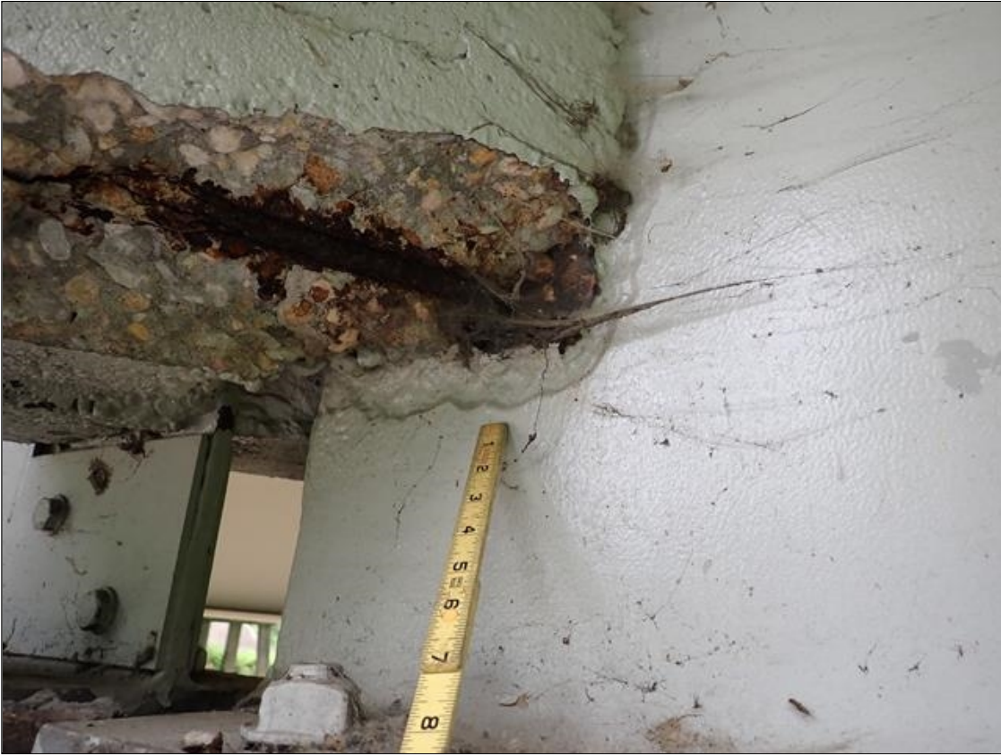
Span 4 Beam 1: (PAR) at bent 4, web adjacent to end diaphragm, painted over section loss (7/16 inch average remaining x 8 inch x 16 inch) with corrosion reactivating
