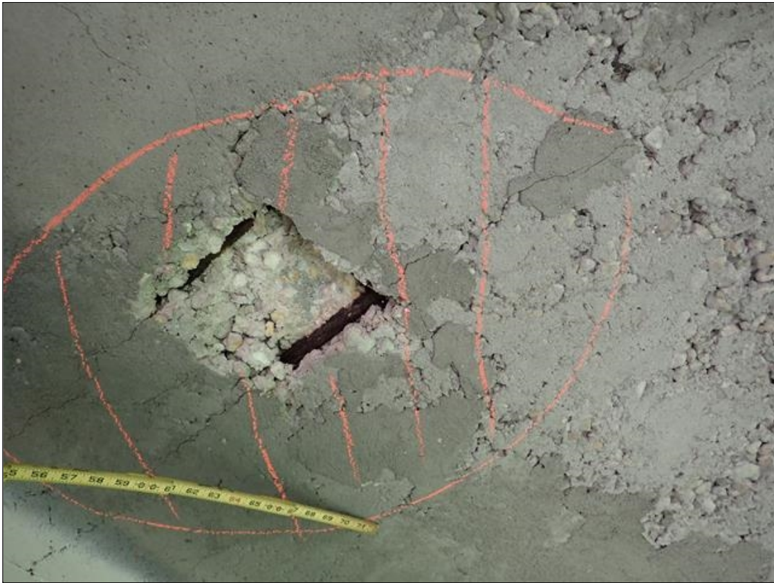
Span 7 Deck: (PAR) underside in bay 3 near midspan, spall/delamination (30 inch x 20 inch x 2 inch deep) with exposed rusted rebar (approximately 85 percent remaining)
