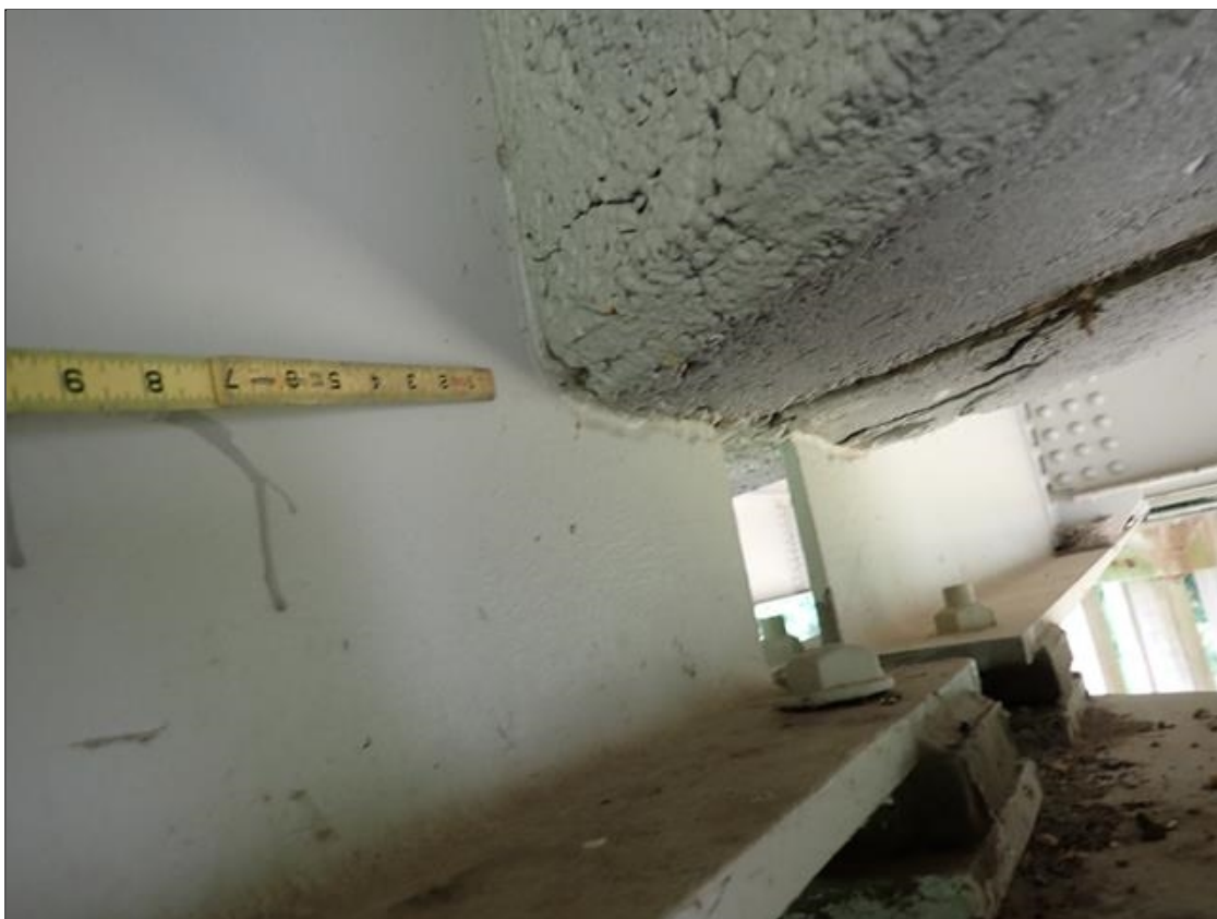
Span 4 Beam 2: at bent 4, web adjacent to end diaphragm, painted over section loss (9/16 inch average remaining x 7 inch x 1 inch)
