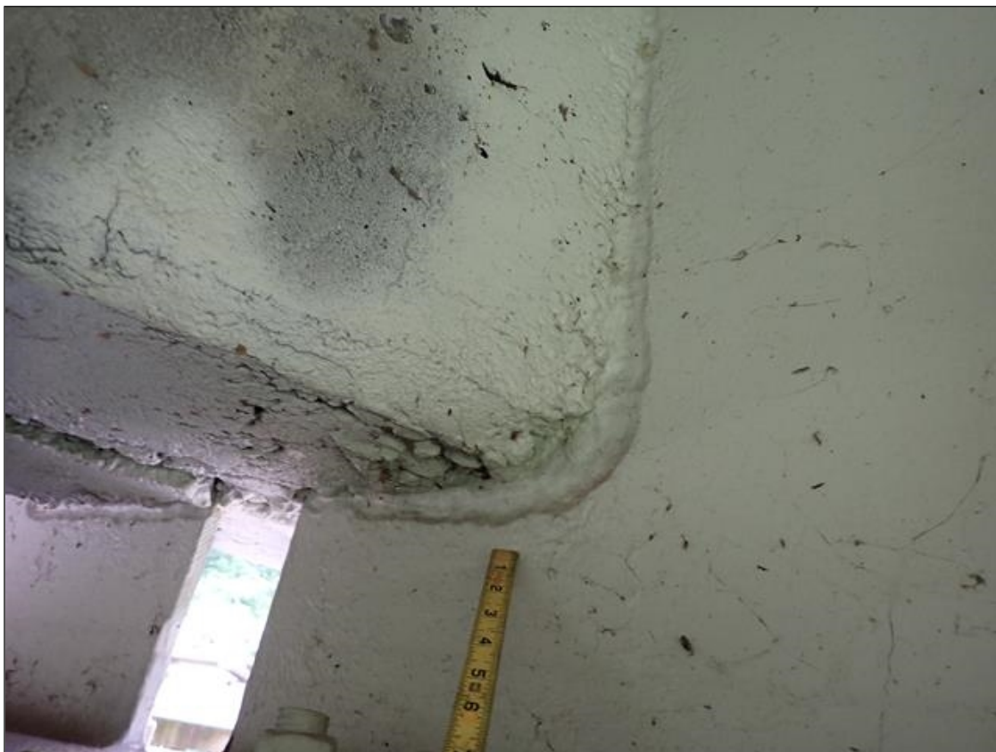
Span 3 Beam 4: (PAR) at bent 3, web adjacent to end diaphragm, painted over section loss (7/16 inch average remaining x 8 inch x 16 inch) with corrosion reactivating
