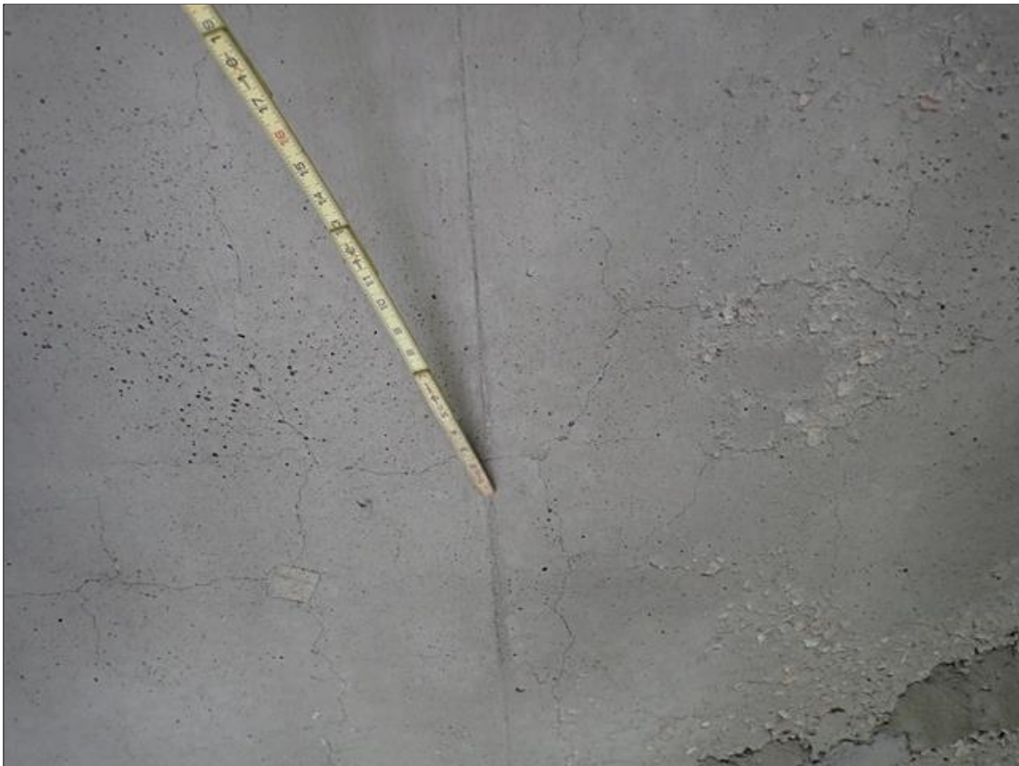
Span 7 Deck: UP TO 0.02 INCH WIDE RANDOM CRACKING IN DECK UNDERSIDE IN ALL BAYS, SCATTERED THROUGHOUT.
