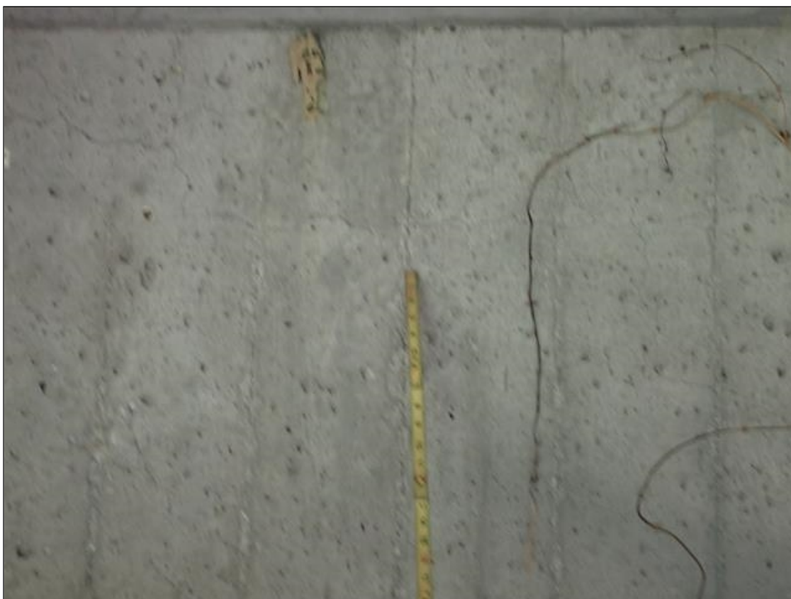
End Bent 1 Abutment: UP TO 0.03 INCH WIDE RANDOM CRACKING IN BACKWALL FOR FULL LENGTH.
