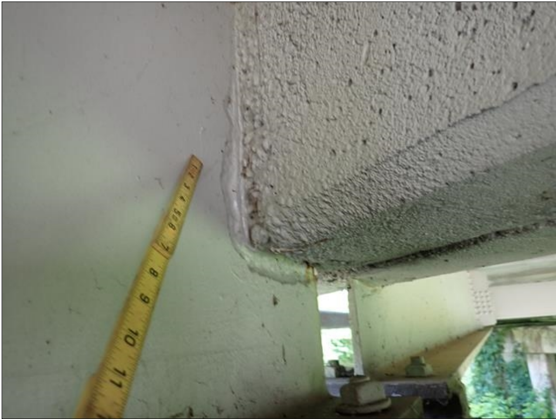
Span 6 Beam 1: (PAR) at bent 6, web adjacent to end diaphragm, painted over section loss (1/4 inch average remaining x 7 inch x 8 inch) with corrosion hole (up to 1/8 inch diameter) and corrosion reactivating
