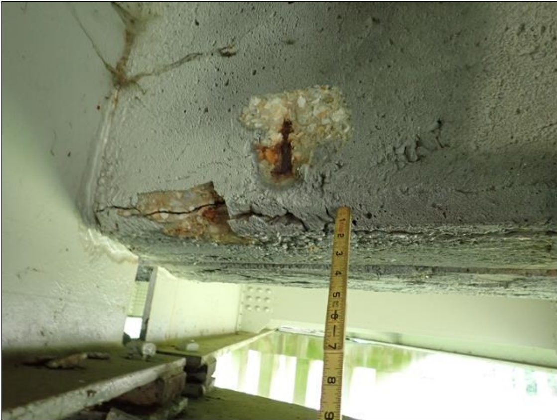
Span 1 Deck: (PAR) BAY 2 FAR DIAPHRAGM ADJACENT TO BEAM 2 AREA OF DELAMINATION AND SPALLING WITH EXPOSED REBAR 1.5 FEET X 8 INCHES X UP TO 3 INCHES DEEP, 5 PERCENT SECTION LOSS.
