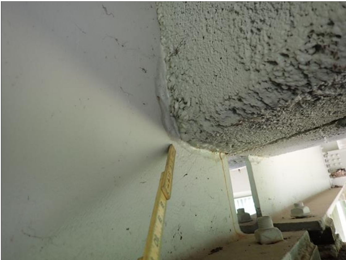
Span 6 Beam 2: (PAR) at bent 5, web adjacent to end diaphragm, painted over section loss (7/16 inch average remaining x 7 inch x 8 inch) with corrosion reactivating
