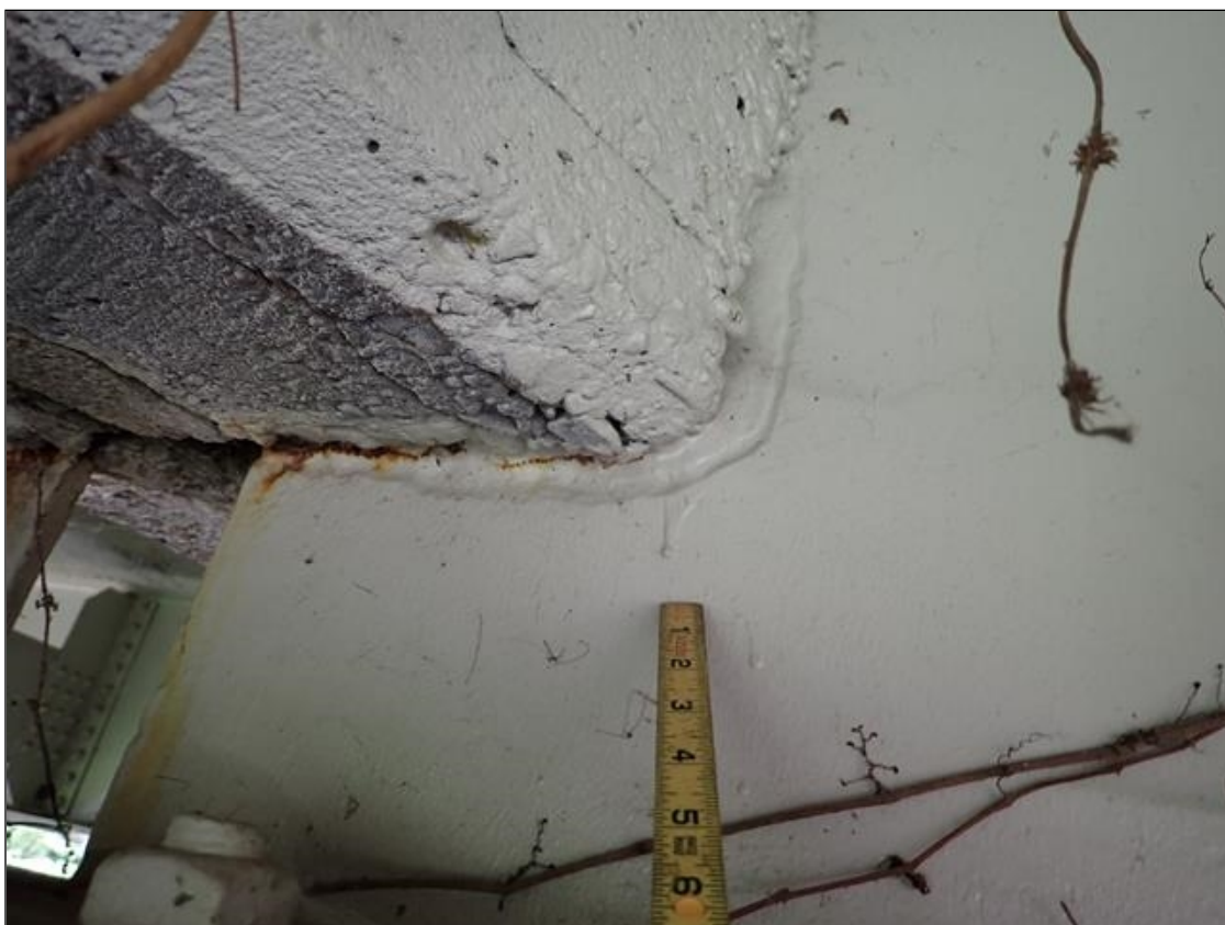
Span 8 Beam 3: (PAR) at bent 7, web adjacent to end diaphragm, painted over section loss (7/16 inch average remaining x 8 inch x 8 inch) with corrosion reactivating
