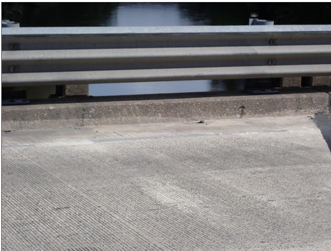
Span 5 Left Bridge Rail: BOTTOM OF CURB NEAR BENT 5 JOINT, (2) UP TO 6 INCH DIAMETER X 1 INCH DEEP SPALLS WITH EXPOSED PAINTED REBAR
