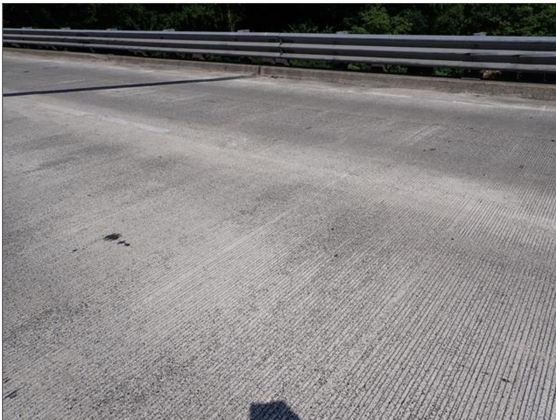
Span 6 Deck: throughout top of deck, wear with secure aggregate at random
