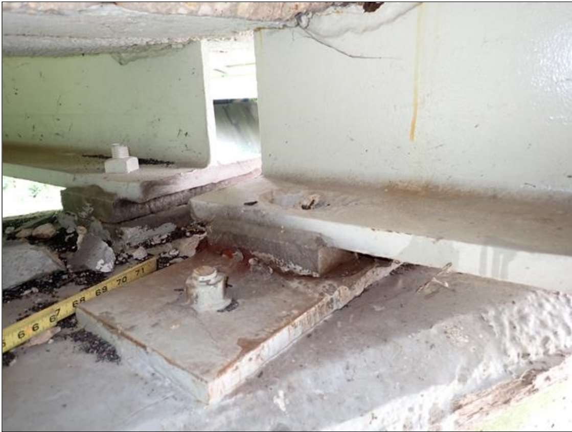
Span 6 Far Bearing 4: LEFT ANCHOR BOLT, MISSING; BEARING ASSEMBLY HAS WELDED REPAIR WITH NEW ANCHOR BOLT.
