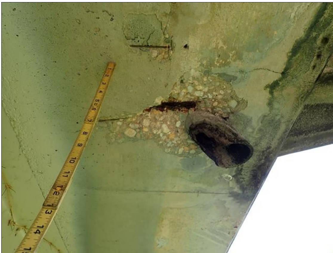
Span 1 Deck: (PAR) UP TO 1 FOOT WIDE X 9 INCHES LONG X UP TO 1 INCH DEEP SPALL WITH EXPOSED REINFORCEMENT IN RIGHT OVERHANG, LOCATED AT THIRD DRAIN PIPE. 15 PERCENT SECTION LOSS IN EXPOSED REINFORCEMENT.
