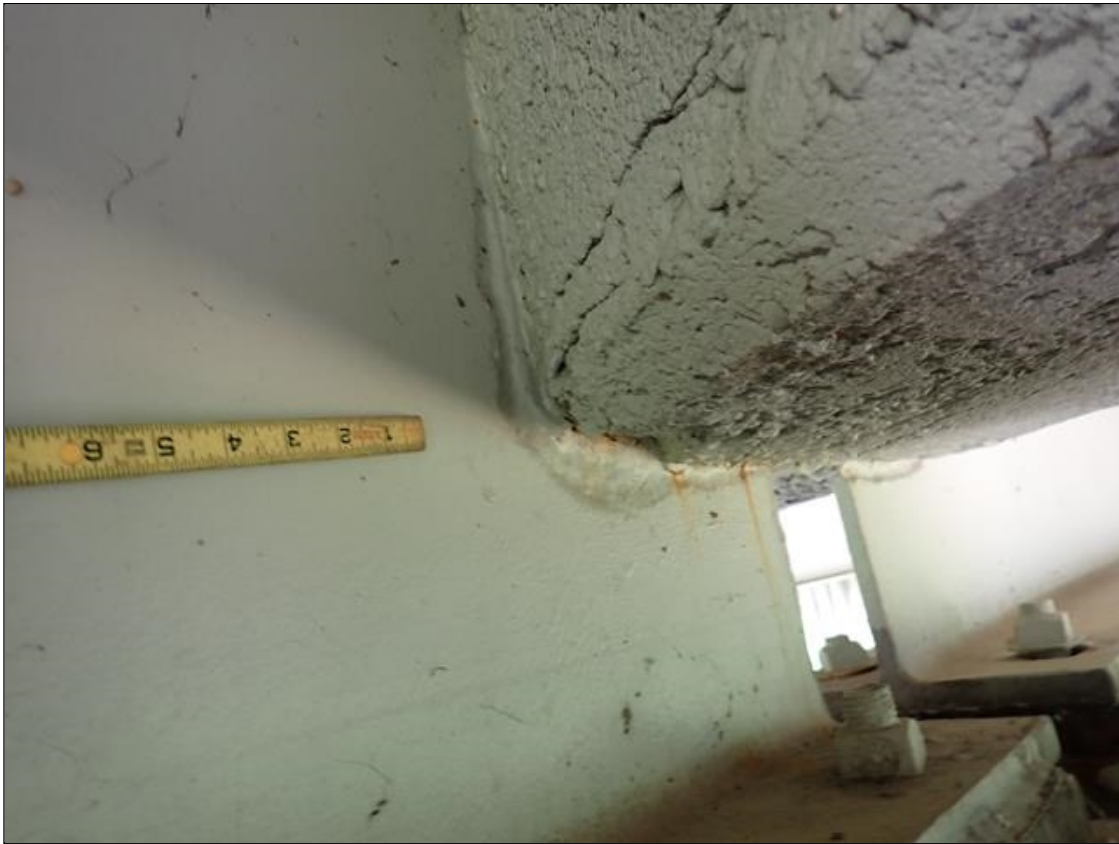
Span 6 Beam 3: (PAR) at bent 5, web adjacent to end diaphragm, painted over section loss (7/16 inch average remaining x 7 inch x 8 inch) with corrosion reactivating
