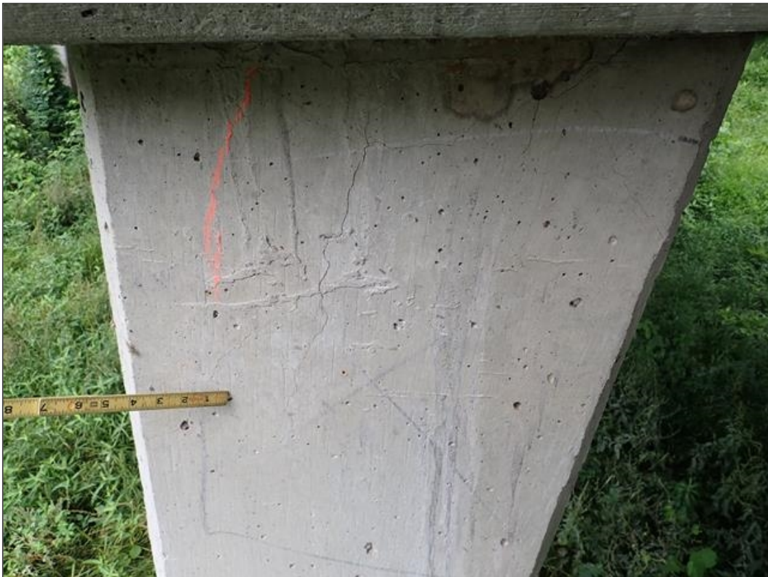
Bent 2 Pile 7: north face at top, delamination (26 inch x 18 inch) with crack (up to 1/64 inch)
