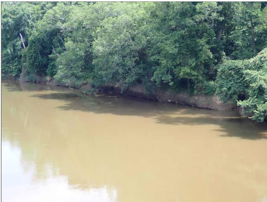
along channel embankments, cutbank erosion (up to 4 foot x 2 foot deep)
