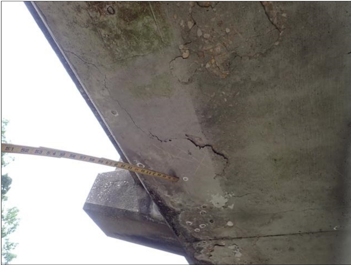
Span 6 Deck: THREE (3) AREAS OF DELAMINATED CONCRETE UP TO 18 INCH X 10 INCH IN EAST OVERHANG AT BENT 6.
