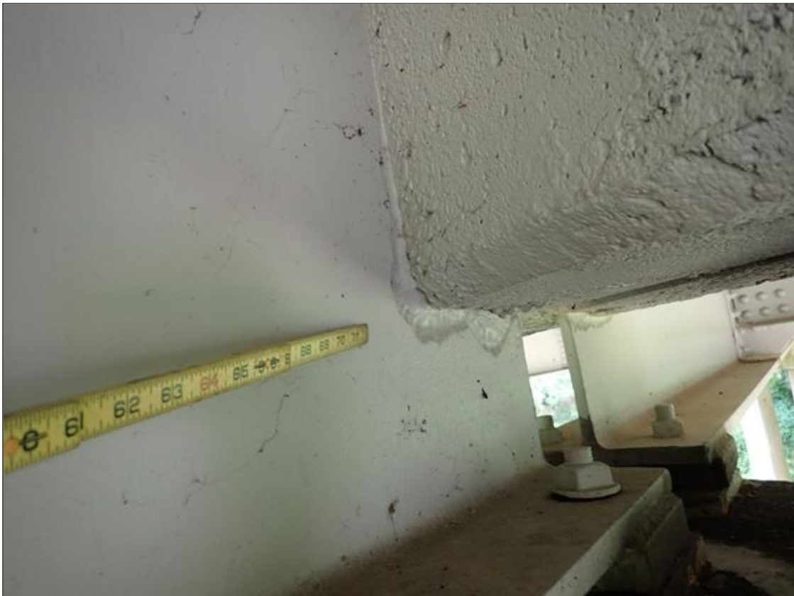
Span 5 Beam 2: (PAR) at bent 5, web adjacent to end diaphragm, painted over section loss (7/16 inch average remaining x 2.5 inch x 8 inch) with corrosion reactivating
