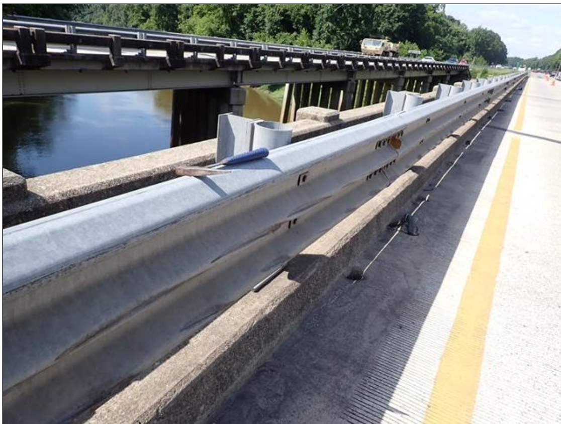
Span 6 Right Retrofit Bridge Rail: (PAR) IMPACT DAMAGE WITH SCRAPE MARKS AND THROUGH HOLES UP TO 4 INCH X 2 INCH IN RETROFIT RAIL AT SCATTERED LOCATIONS
