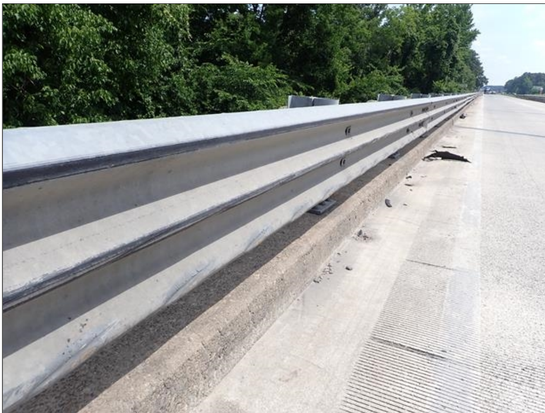
Span 2 Left Retrofit Bridge Rail: (PAR) IMPACT DAMAGE WITH SCRAPE MARKS AND DENTS UP TO 1 INCH DEEP IN RETROFIT RAIL AT SCATTERED LOCATIONS
