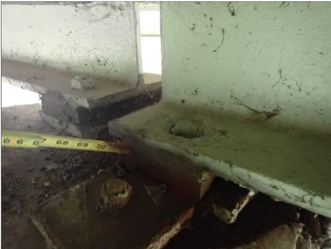
Span 2 Far Bearing 3: BOTH ANCHOR BOLTS, MISSING; WELDED BEARING REPAIR WITH ANCHOR ROD.
