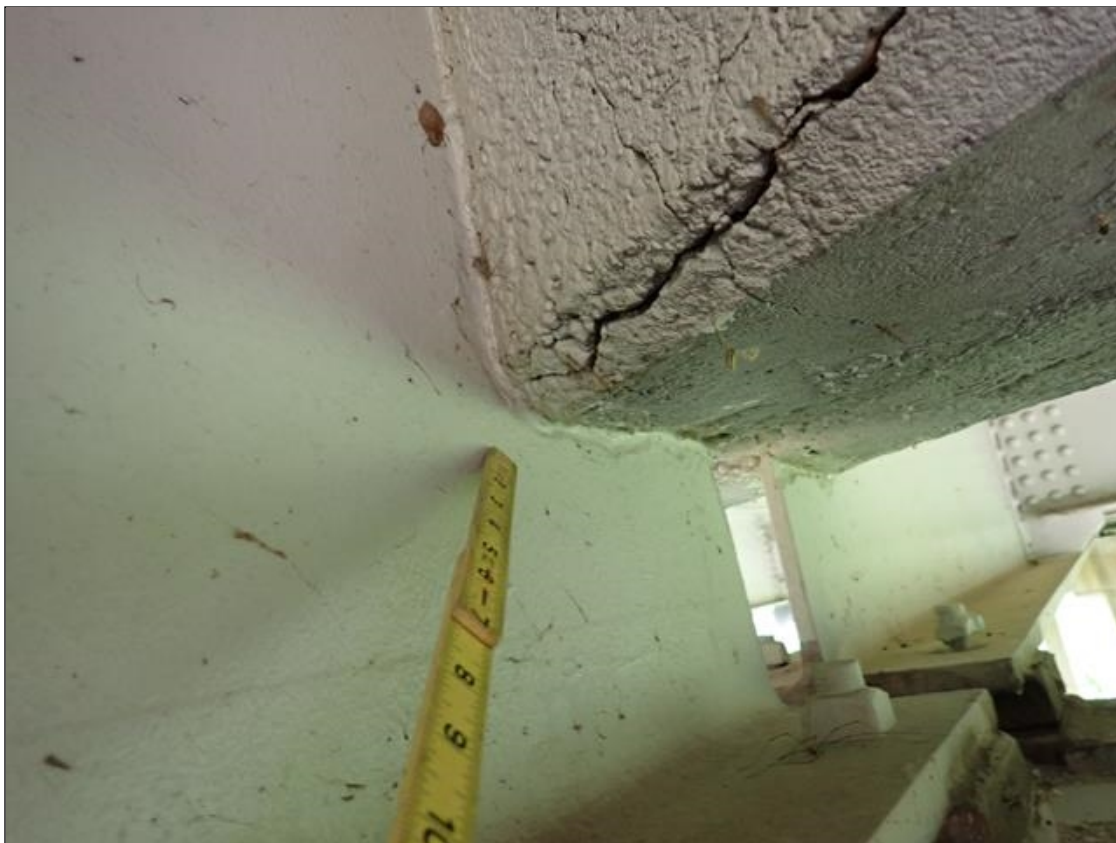
Span 4 Beam 3: (PAR) at bent 3, web adjacent to end diaphragm, painted over section loss (1/2 inch average remaining x 8 inch x 3 inch)
