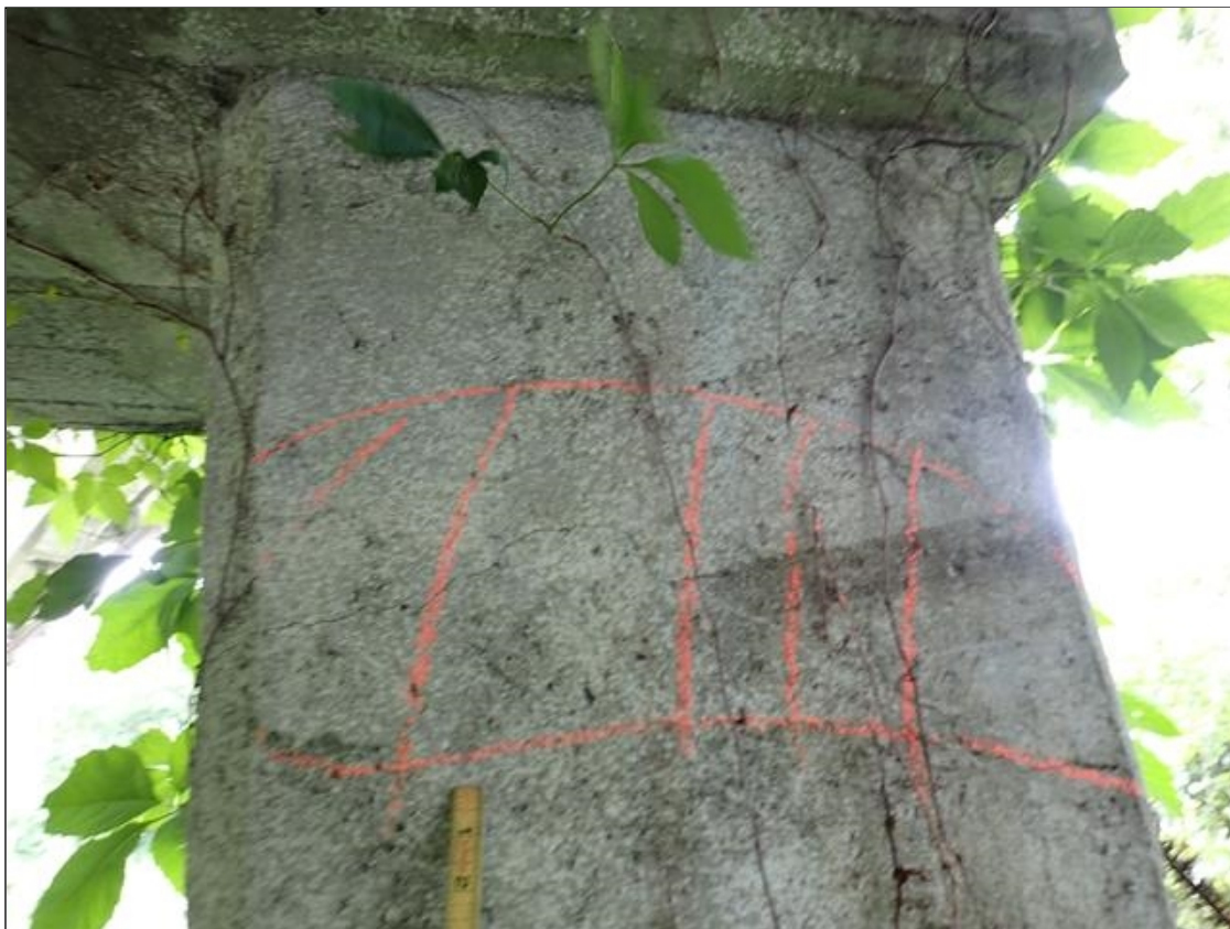
Bent 7 Pile 1: 18 INCH X 8 INCH DELAMINATION IN NORTH FACE FACE NEAR CAP
