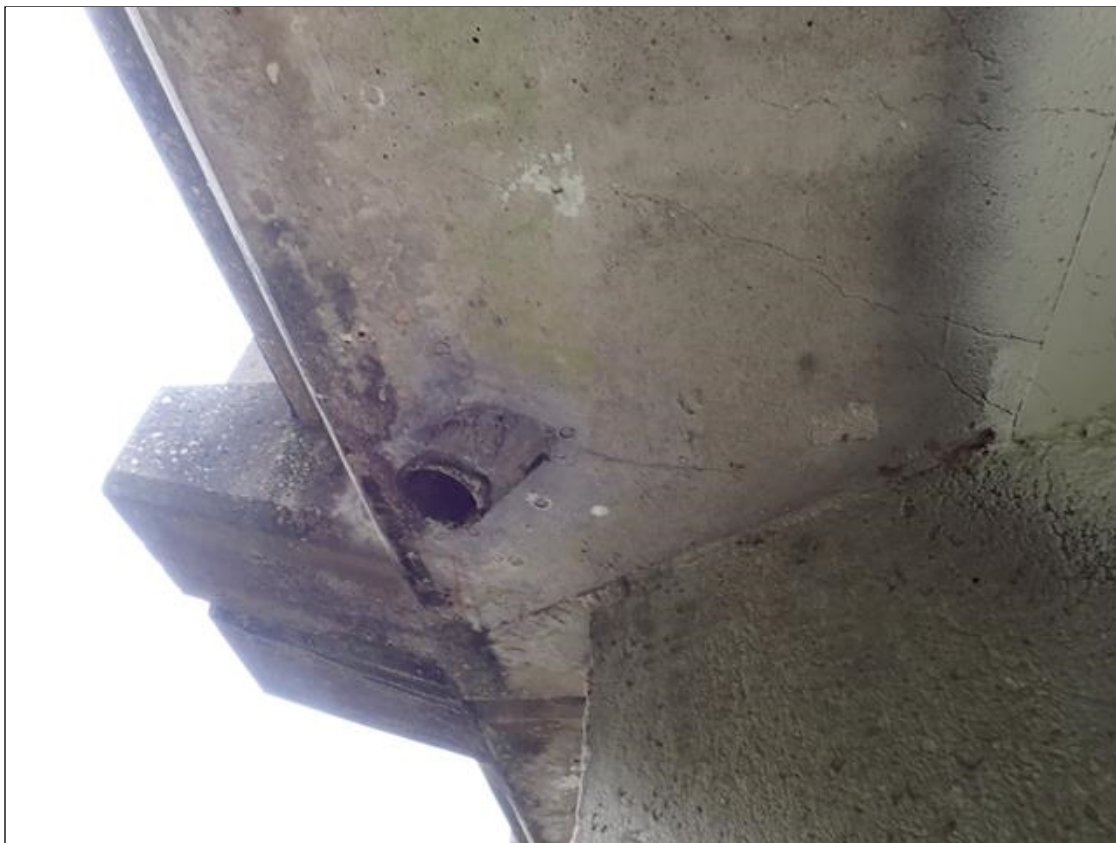
Span 6 Deck: (not found 2025) 12 INCHES DIAMETER SOUND CONCRETE PATCH IN EAST OVERHANG AT DRAIN ONE.
