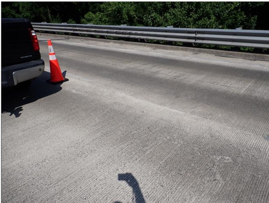
Span 8 Deck: throughout top of deck, wear with secure aggregate at random
