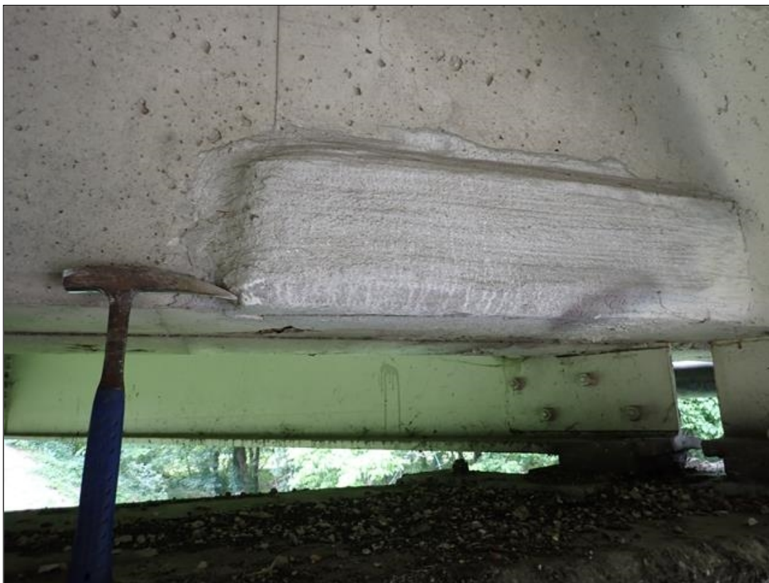
Span 3 Deck: 3 FEET LONG X 1 FOOT HIGH UNSOUND CONCRETE PATCH, BAY 1 END DIAPHRAGM, AT BENT 2.
