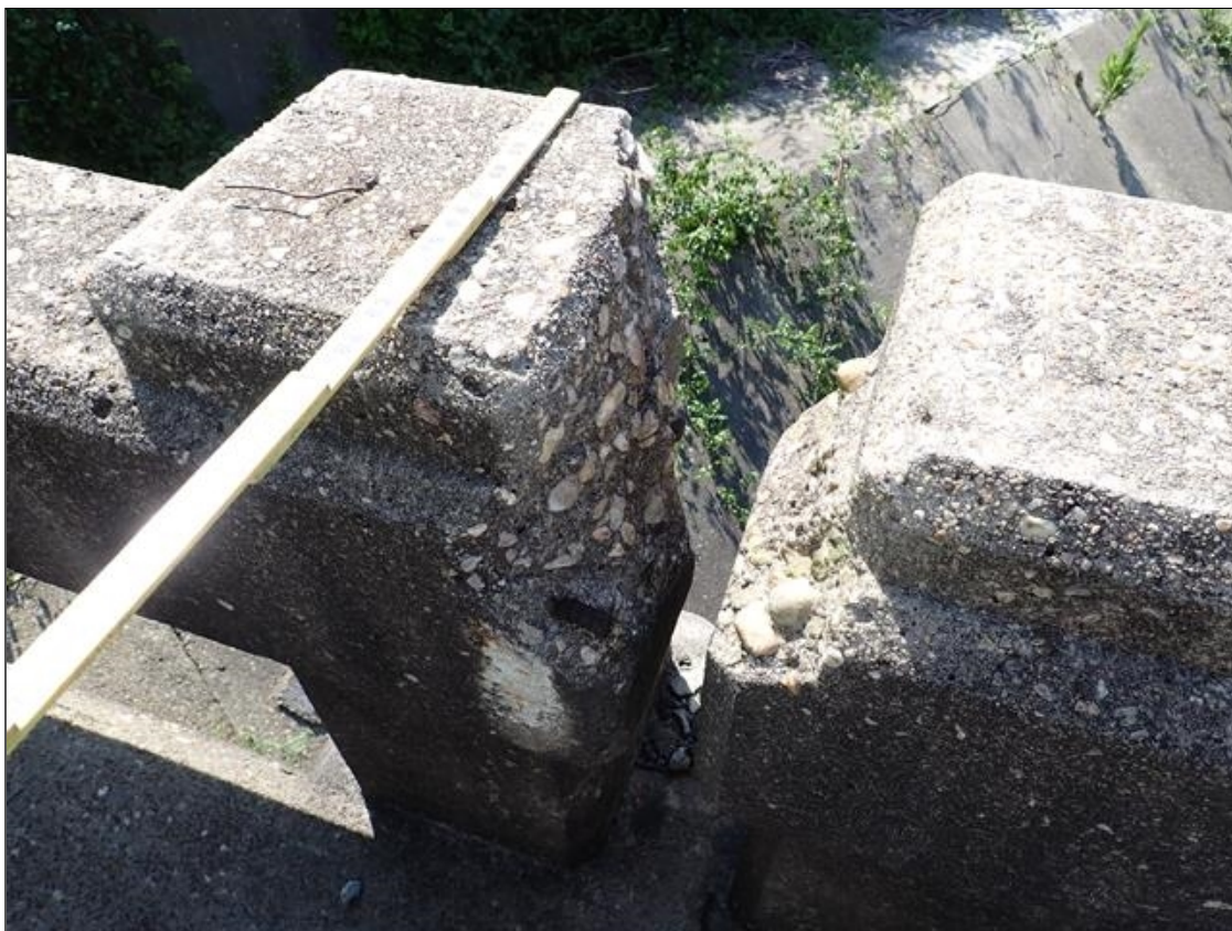
Span 8 Right Bridge Rail: at posts 6 and 7 from bent 7, spalls (up to 16 inch x 12 inch x 2 inch deep) with exposed rusted rebar
