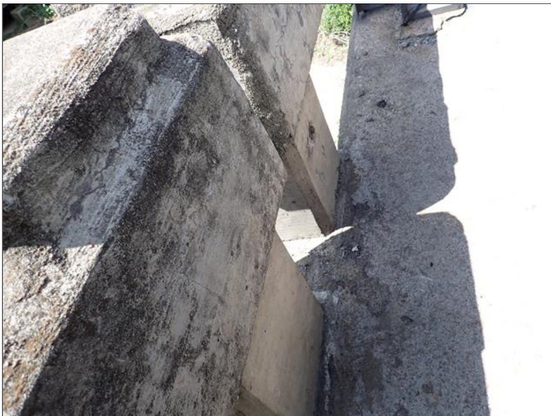
Span 1 Right Bridge Rail: BEGINNING 8 FEET FROM END BENT 1, 20 FEET OF SOUND PATCHING WITH CRACKS (HAIRLINE) AND EFFLORESCENCE
