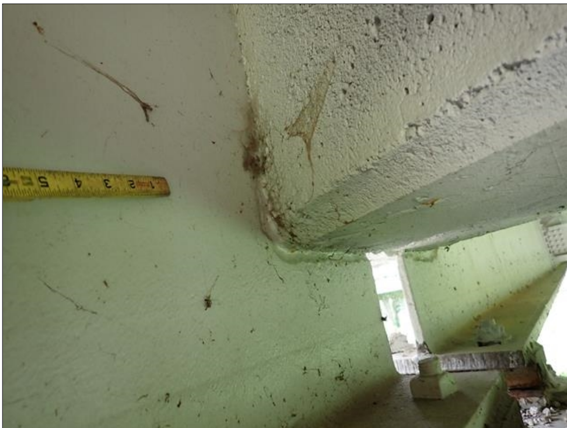
Span 4 Beam 4: (PAR) at bent 3, web adjacent to end diaphragm, painted over section loss (7/16 inch average remaining x 8 inch x 4 inch)
