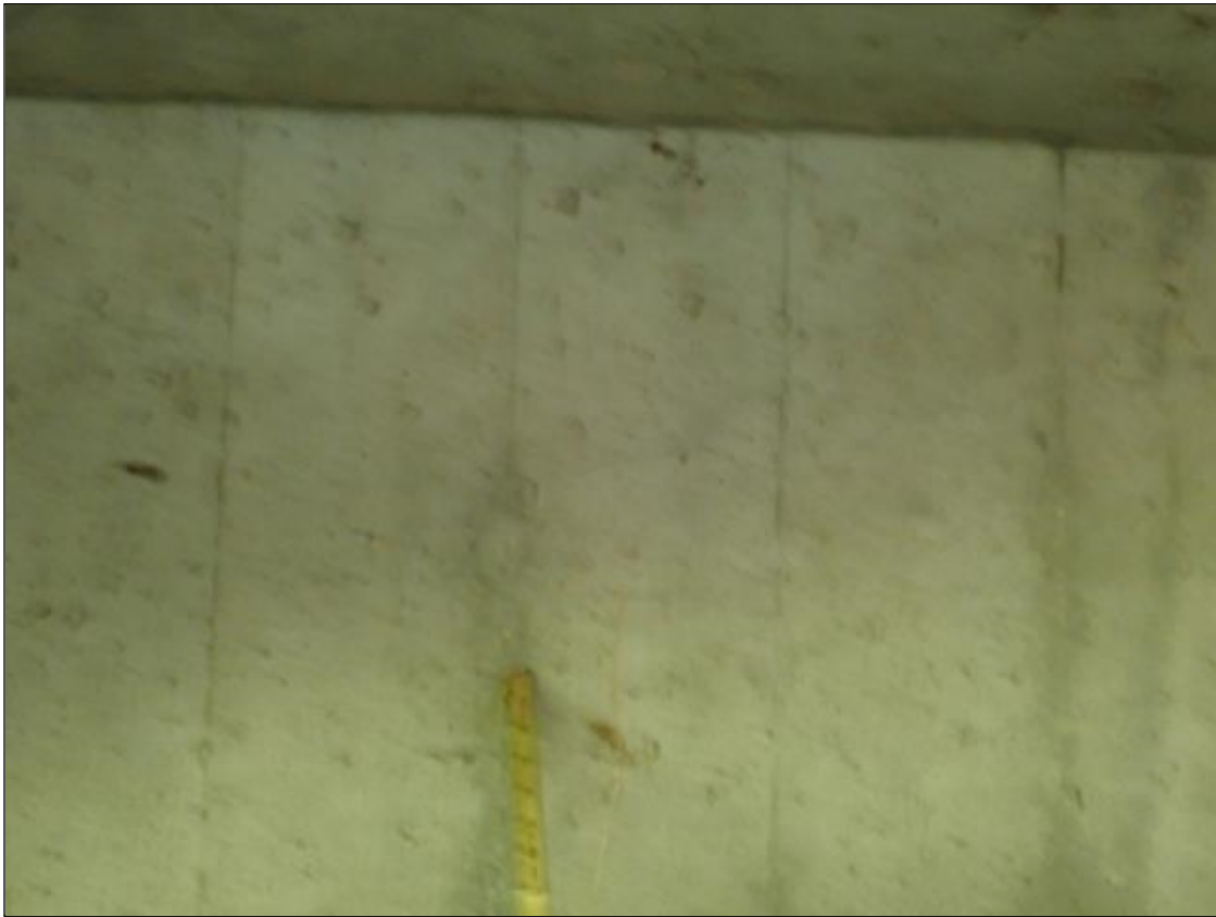
End Bent 2 Cap 1: along abutment, vertical and horizontal cracks (up to 1/32 inch x 4 foot) at random
