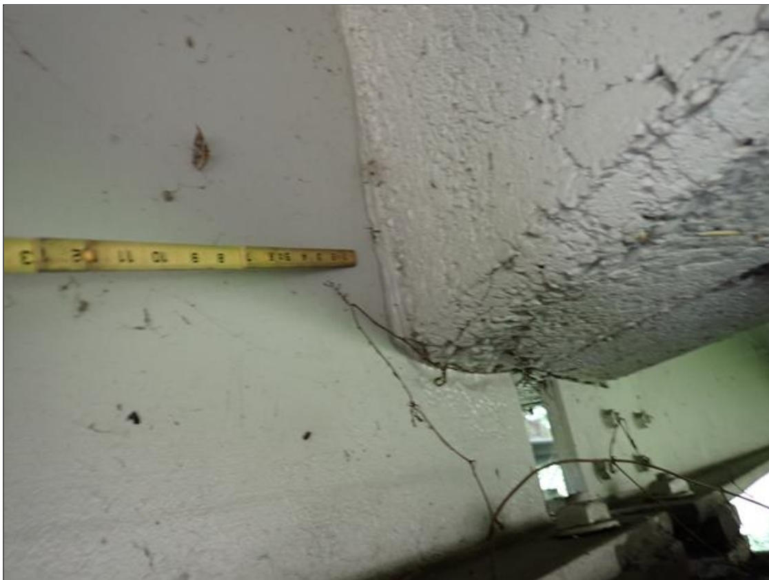
Span 7 Beam 1: (PAR) at bent 7, web adjacent to end diaphragm, painted over section loss (7/16 inch average remaining x 7 inch x 7 inch)
