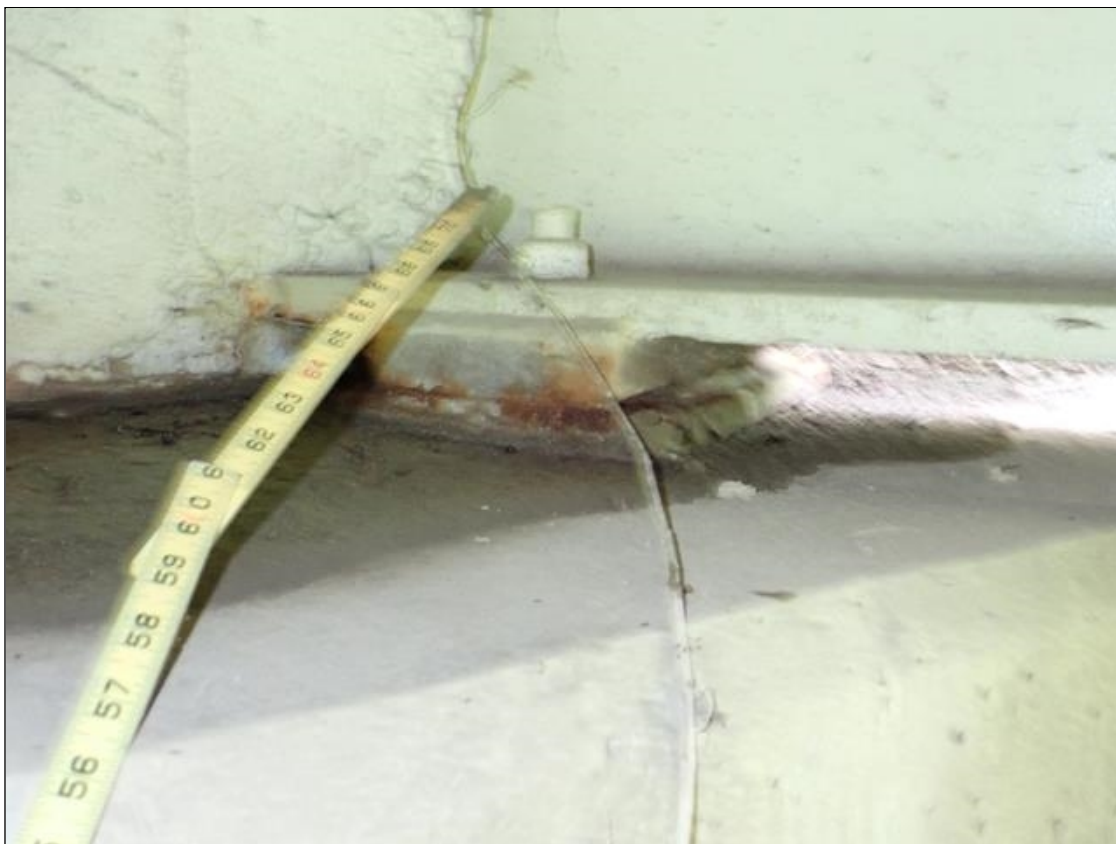
Span 8 Far Bearing 4: painted over section loss (approximately 80 percent remaining) with corrosion reactivating
