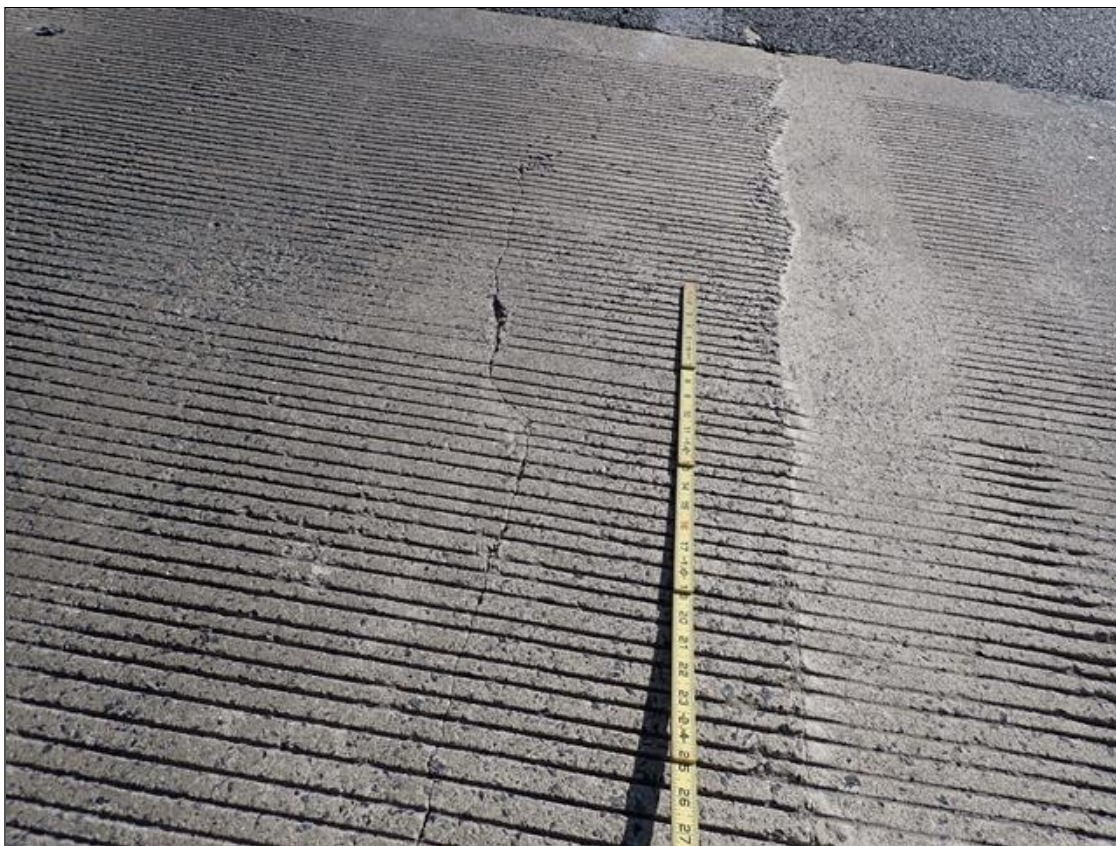
Approach 2: UP TO 0.05 INCH WIDE DIAGONAL AND LONGITUDINAL CRACKS IN BOTH TRAVEL LANES.
