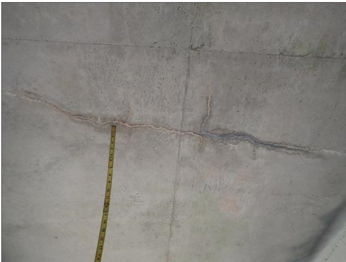
Span 6 Deck: 8 FEET LONG X HAIRLINE TRANSVERSE CRACKS WITH EFFLORESCENCE, UNDERSIDE OF DECK, AT RANDOM THROUGHOUT BAY 1. SIMILAR IN BAY 3.
