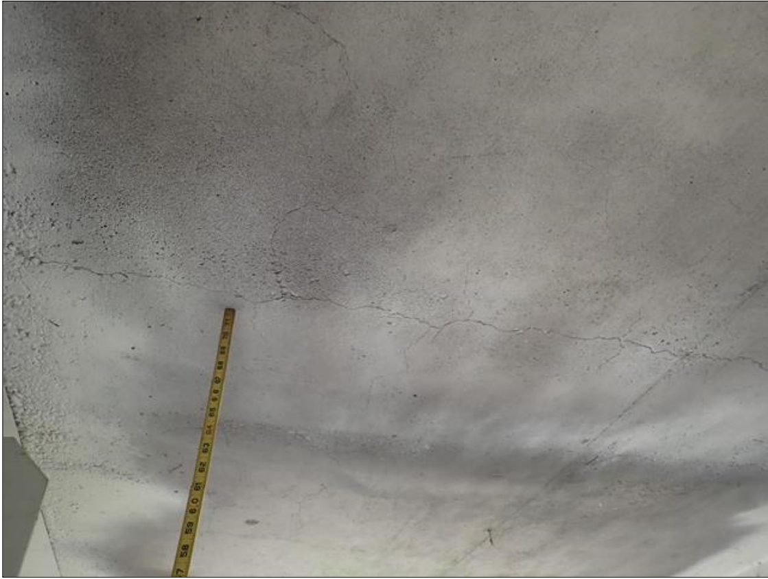
Span 5 Deck: UP TO 1/32 INCH WIDE RANDOM CRACKING IN DECK UNDERSIDE IN ALL BAYS, SOME WITH EFFLORESCENCE, SCATTERED THROUGHOUT.
