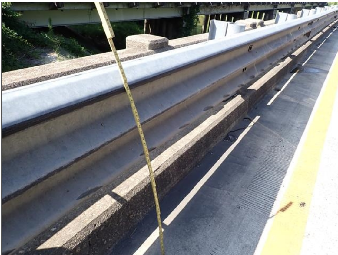
Span 8 Right Retrofit Bridge Rail: (PAR) IMPACT DAMAGE WITH SCRAPE MARKS AND THROUGH HOLES UP TO 4 INCH X 2 INCH IN RETROFIT RAIL AT SCATTERED LOCATIONS
