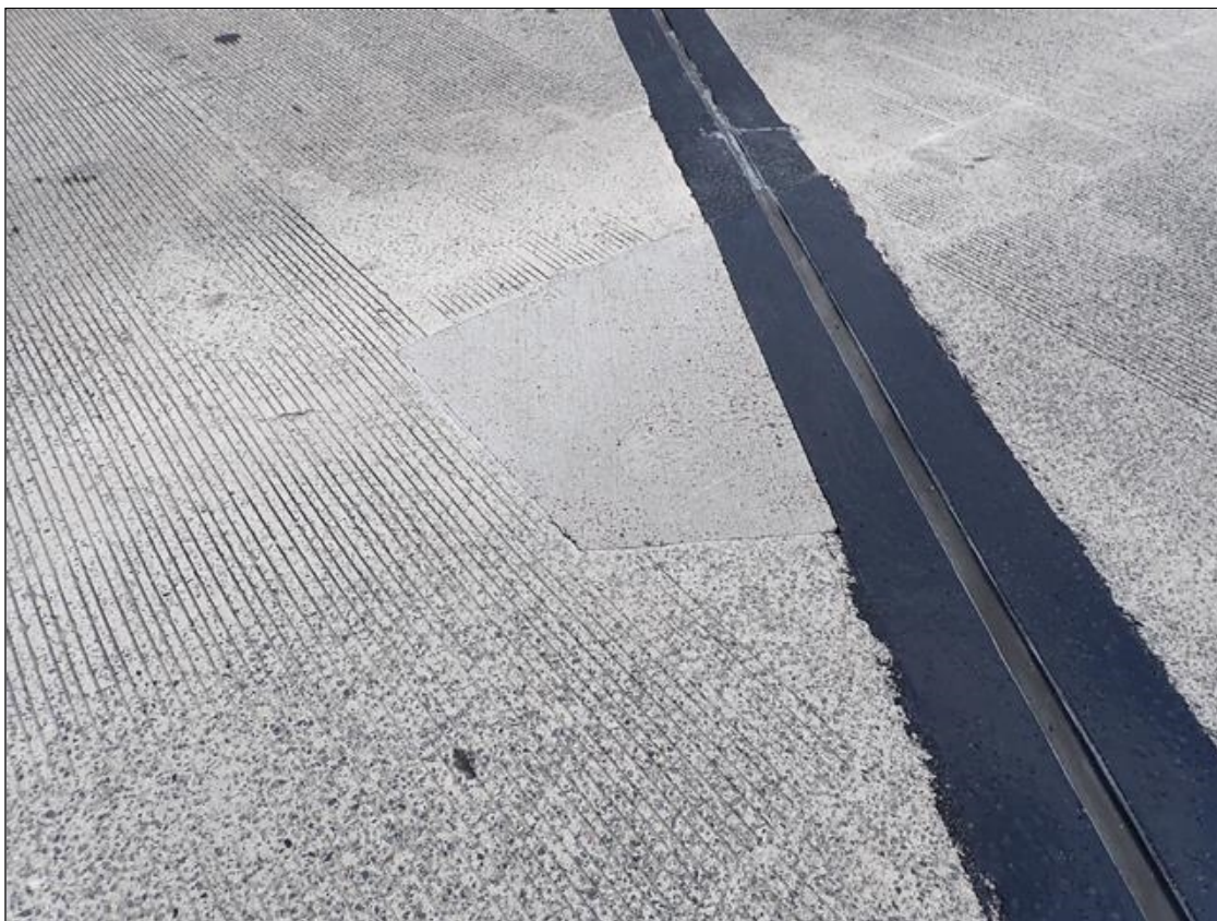
Span 4 Deck: 3 FEET LONG X 2 FEET WIDE SOUND CONCRETE PATCH IN LEFT TRAVEL LANE AT BENT 4.
