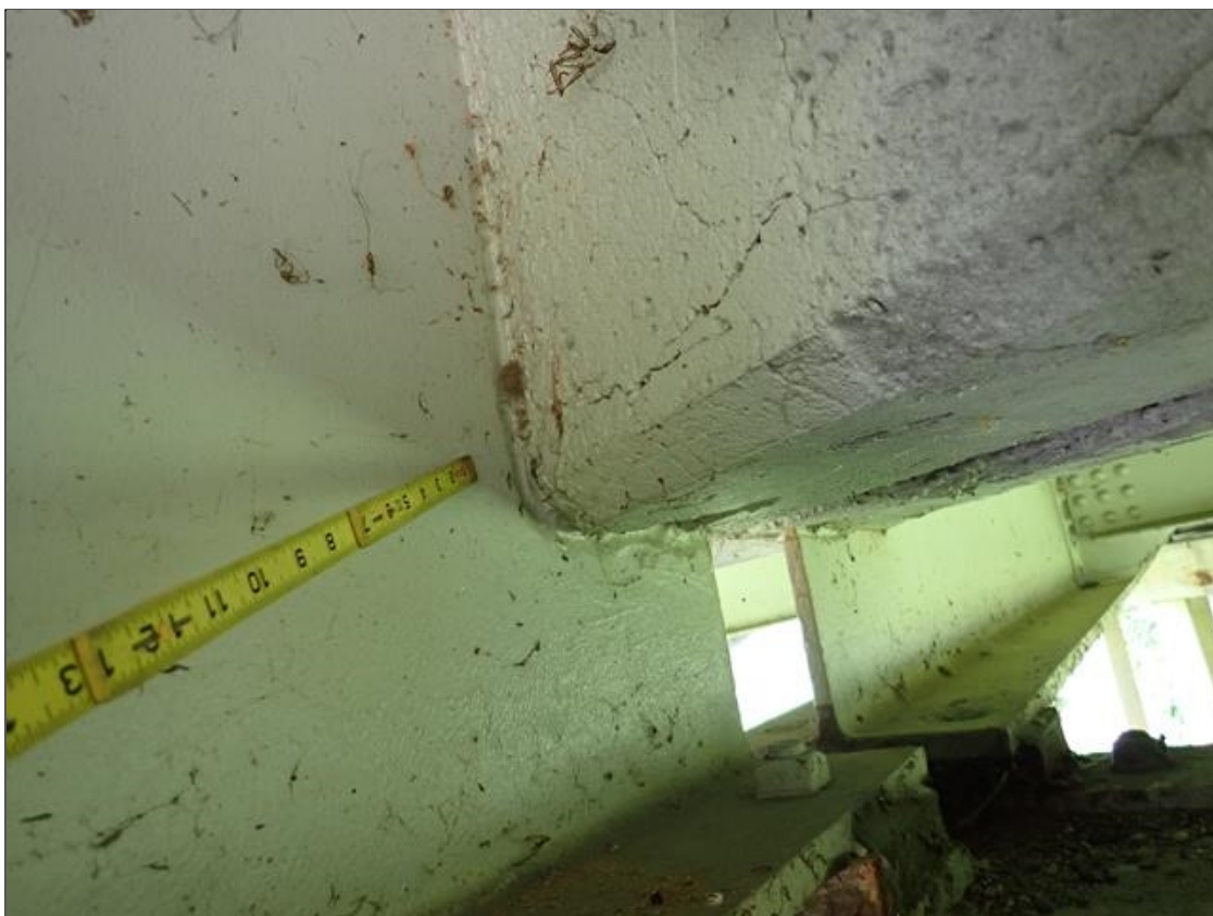
Span 3 Beam 3: (PAR) at bent 2, web adjacent to end diaphragm, painted over section loss (7/16 inch average remaining x 4 inch x 8 inch) with corrosion reactivating
