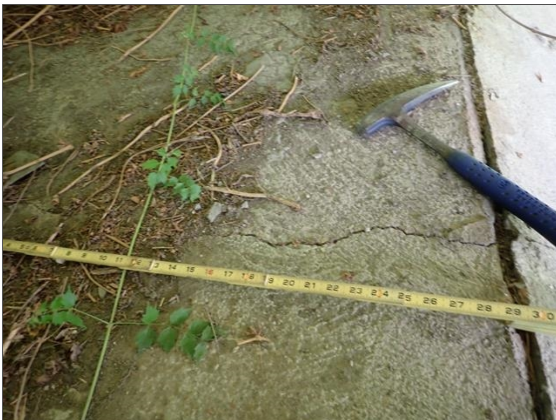
end bent 1 slope protection, below bay 3, transverse cracks (up to 1/16 inch x 4 foot)
