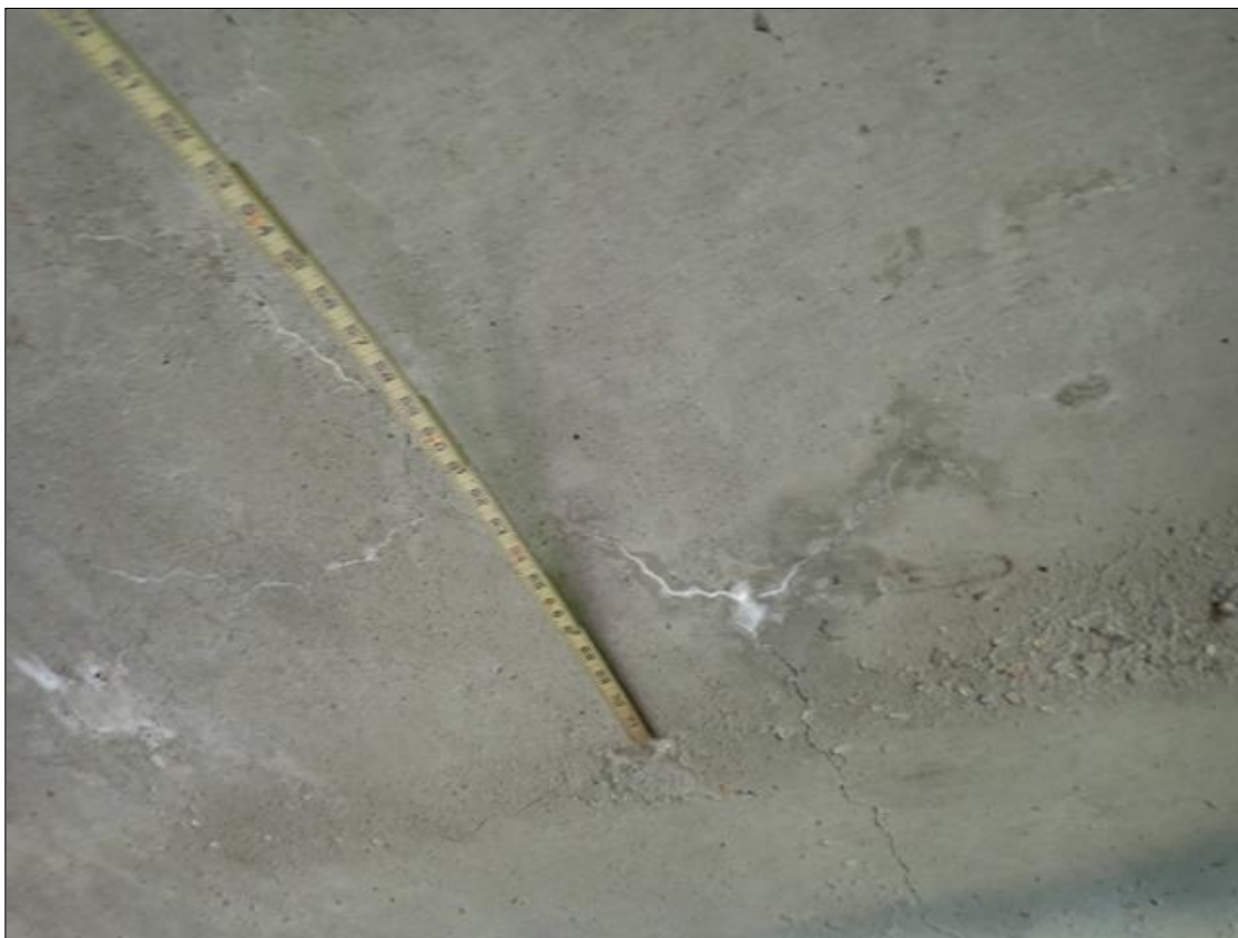
Span 1 Deck: UP TO 0.02 INCH WIDE RANDOM CRACKING SOME WITH EFFLORESCENCE IN DECK UNDERSIDE IN ALL BAYS, SCATTERED THROUGHOUT.
