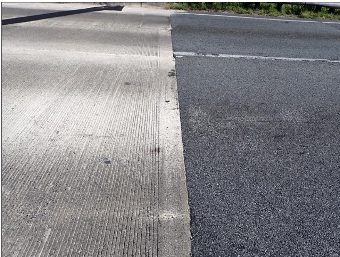
Approach 2: (not found 2025) ASPHALT AT SOUTH END SETTLED FULL WIDTH X UP TO 1 1/2 INCH.
