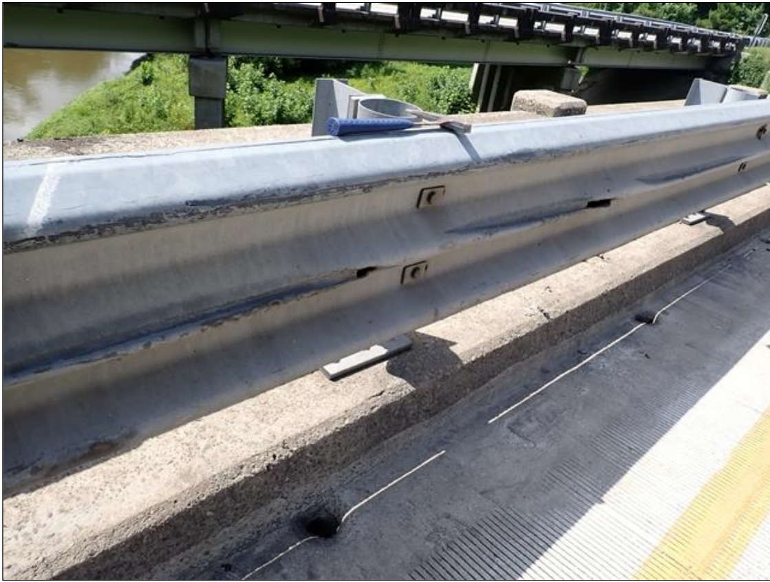
Span 2 Right Retrofit Bridge Rail: (PAR) IMPACT DAMAGE WITH SCRAPE MARKS AND THROUGH HOLES UP TO 4 INCH X 2 INCH IN RETROFIT RAIL AT SCATTERED LOCATIONS
