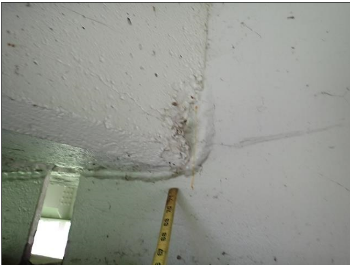
Span 1 Beam 2: (PAR) at bent 1, web adjacent to end diaphragm, painted over section loss (7/16 inch average remaining x 8 inch x 12 inch)
