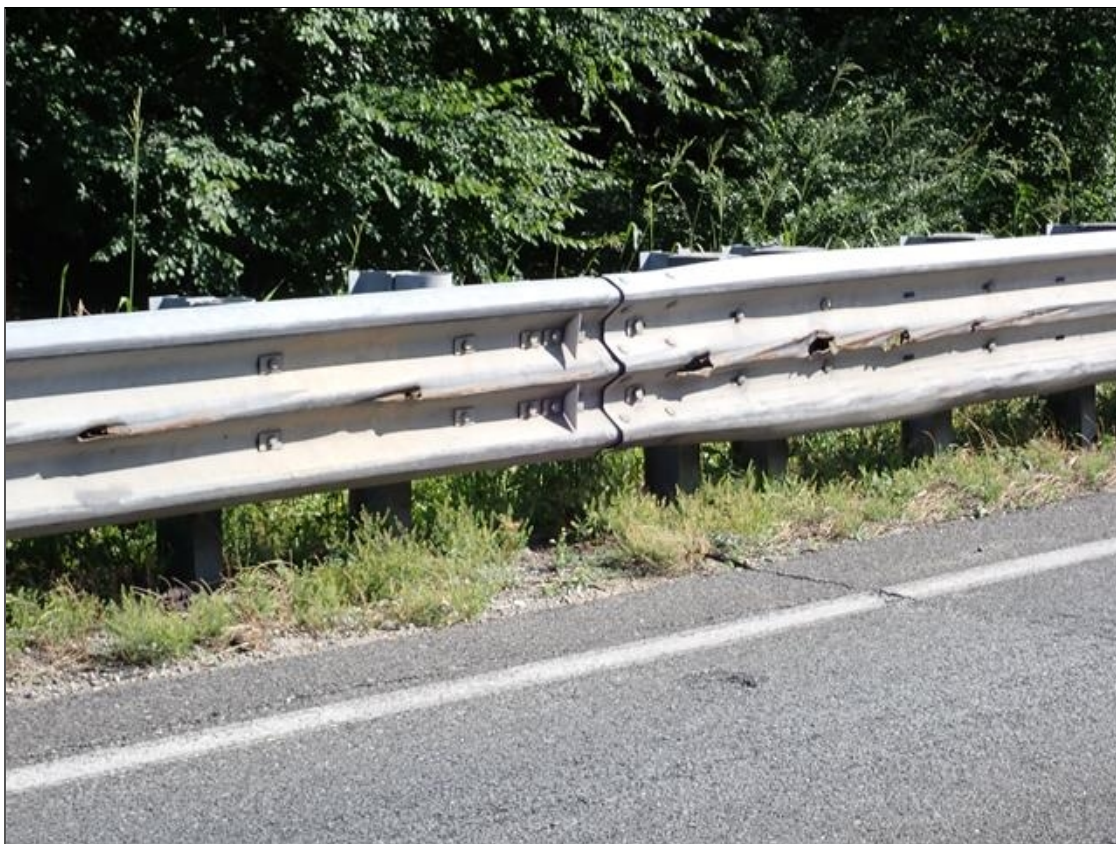
(PAR) northwest guardrail near bridge, impact damage (25 foot) with holes (up to 4 inch x 3 inch)
