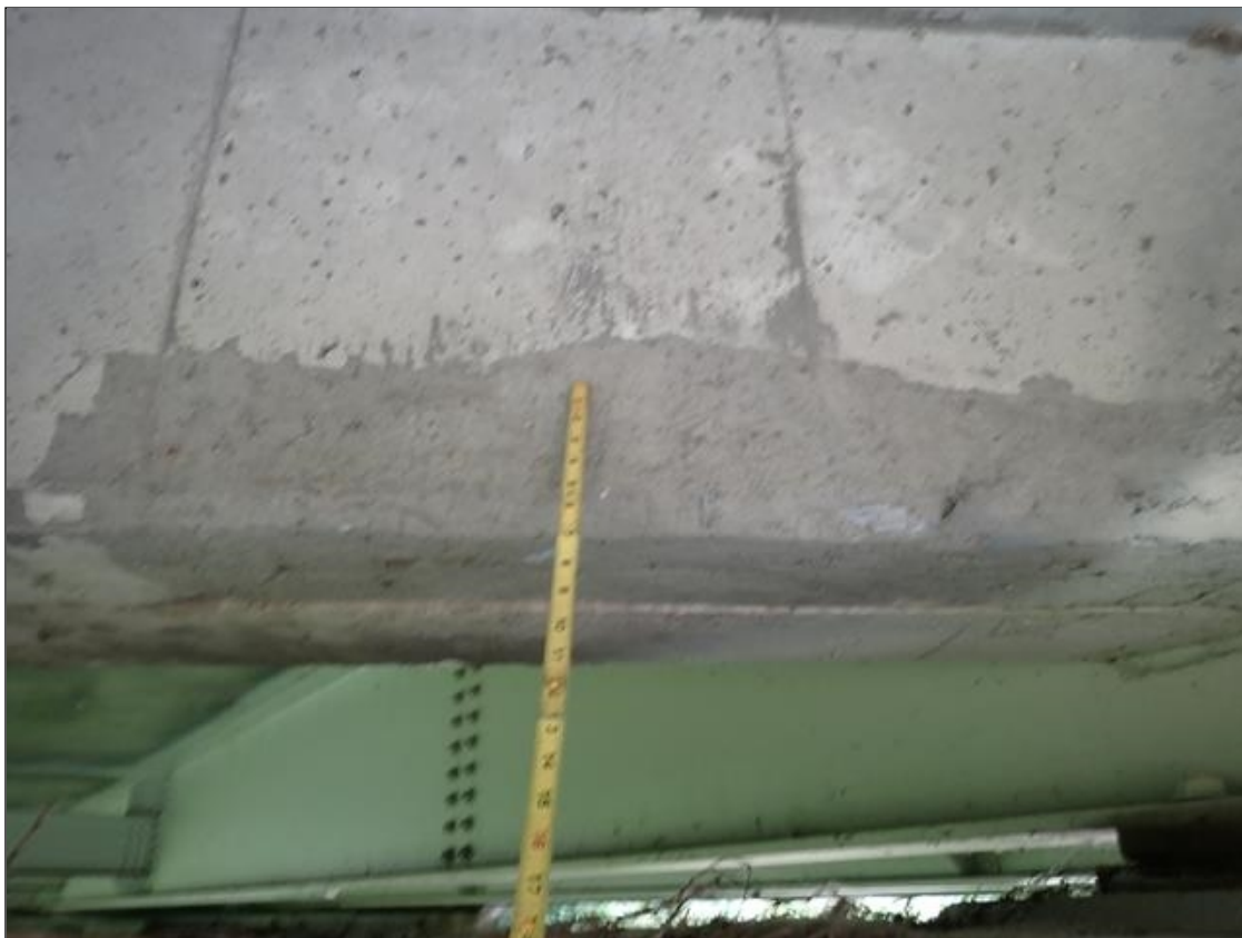
Span 7 Deck: 20 INCHES WIDE X 18 INCHES HIGH SOUND CONCRETE PATCHED AREA, BAY 1 END DIAPHRAGM, OVER BENT 7, NEXT TO BEAM 2.
