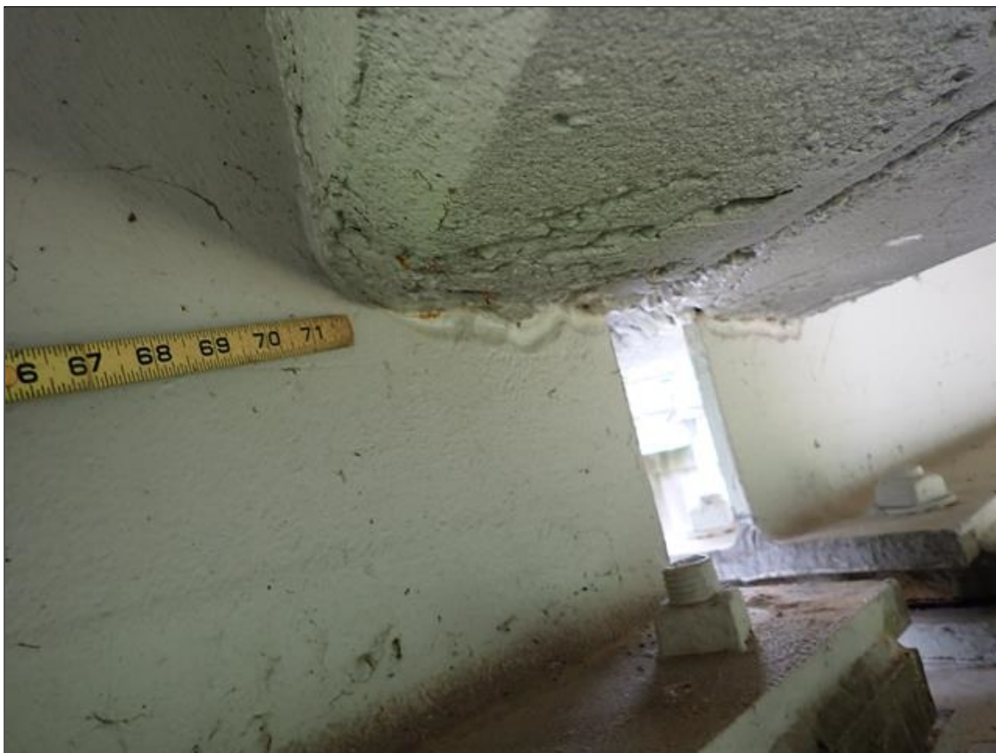
Span 6 Beam 4: (PAR) at bent 5, web adjacent to end diaphragm, painted over section loss (7/16 inch average remaining x 5 inch x 1 inch) with corrosion reactivating
