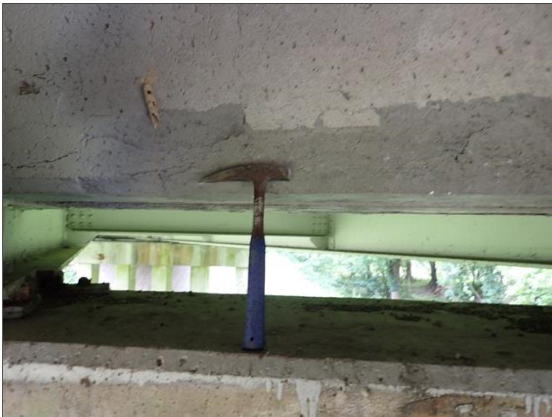
Span 3 Deck: 7 FEET LONG X 6 INCHES HIGH UNSOUND CONCRETE PATCH IN BAY 2 END DIAPHRAGM, AT BENT 2.
