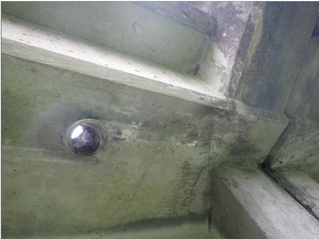
Span 2 Deck: 1 FOOT WIDE X 2 FEET HIGH SOUND CONCRETE PATCH IN DIAPHRAGM OUTSIDE OF BEAM 4 AT BENT 2.
