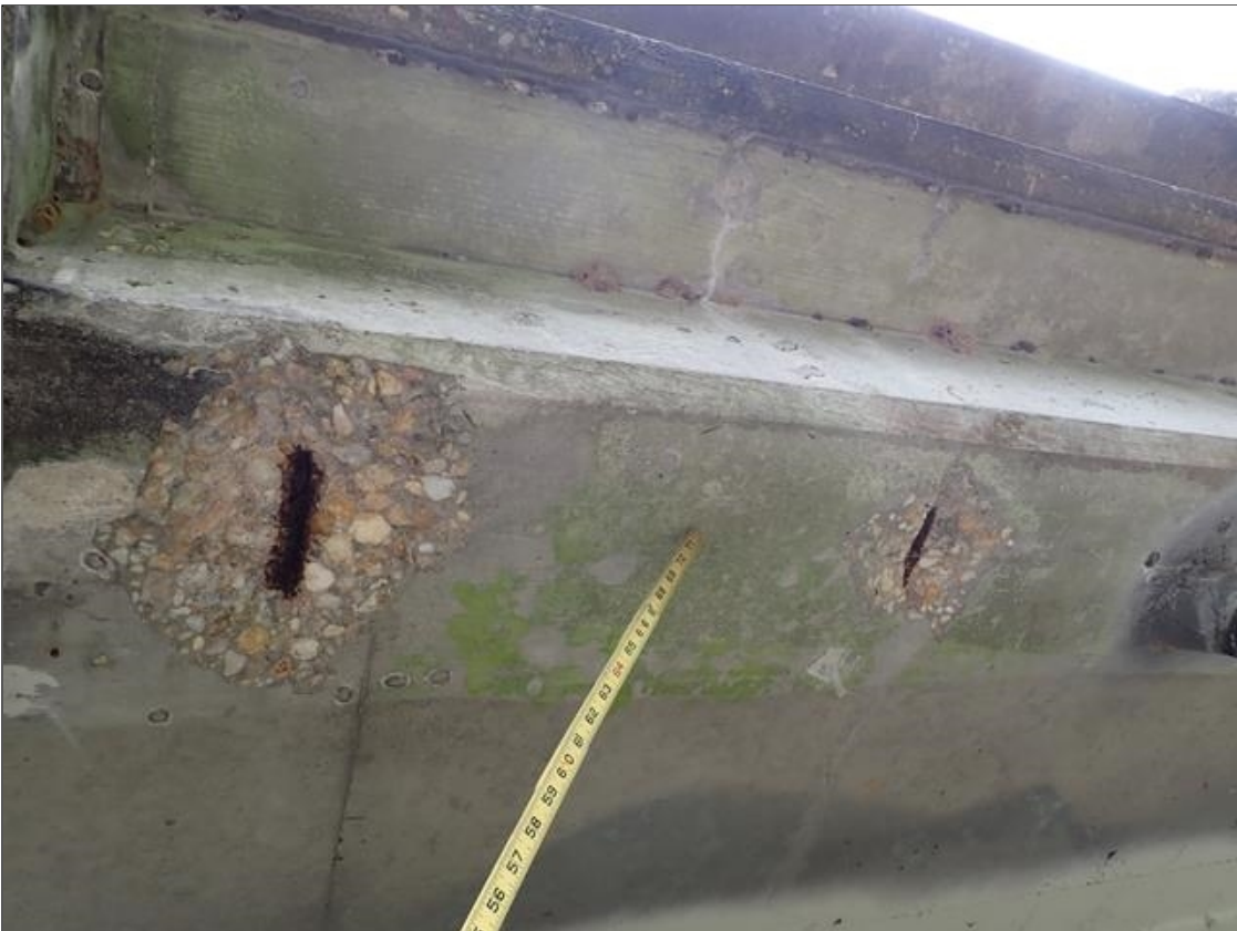
Span 4 Deck: (PAR) LEFT OVERHANG NEAR MIDSPAN 2 SPALLS WITH EXPOSED REBAR UP TO 10 INCHES DIAMETER X 1 INCH DEEP, 5 PERCENT SECTION LOSS.
