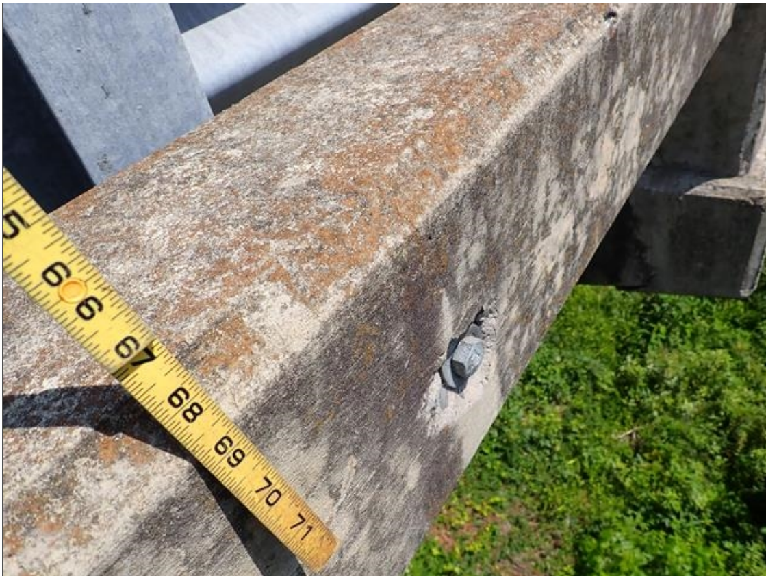
Span 1 Right Bridge Rail: 4 INCH X 3 INCH X 1 INCH DEEP SPALLS IN EXTERIOR FACE AT ANCHOR BOLT CONNECTION TO RETROFIT RAIL AT ISOLATED LOCATIONS
