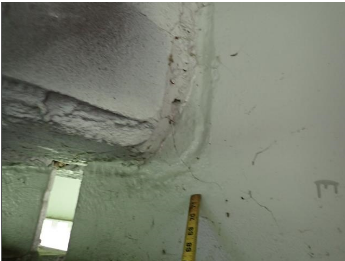
Span 1 Beam 3: (PAR) at bent 1, web adjacent to end diaphragm, painted over section loss (7/16 inch average remaining x 8 inch x 18 inch)
