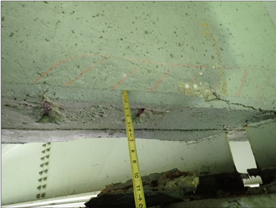
Span 2 Deck: THREE (3) 6 INCHES DIAMETER X 3/4 INCH DEEP SPALLS WITH EXPOSED REINFORCING AND AREA OF DELAMINATION 3 FEET X 7 INCHES, UNDERSIDE AND FACE OF BAY 1 END DIAPHRAGM, AT BENT 2.
