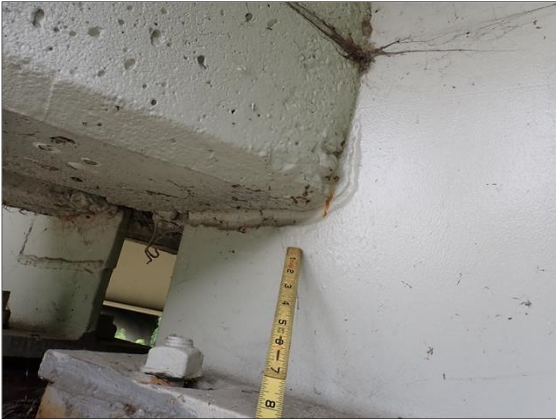
Span 5 Beam 1: (PAR) at bent 5, web adjacent to end diaphragm, painted over section loss (7/16 inch average remaining x 8 inch x 10 inch) with corrosion reactivating
