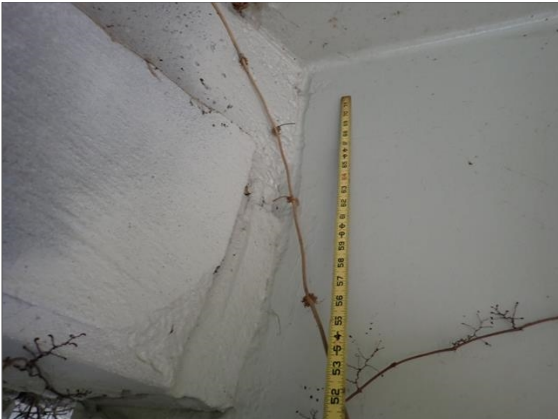
Span 7 Beam 4: (PAR) at bent 7, web adjacent to end diaphragm, painted over section loss (7/16 inch average remaining x 1 inch x 24 inch)
