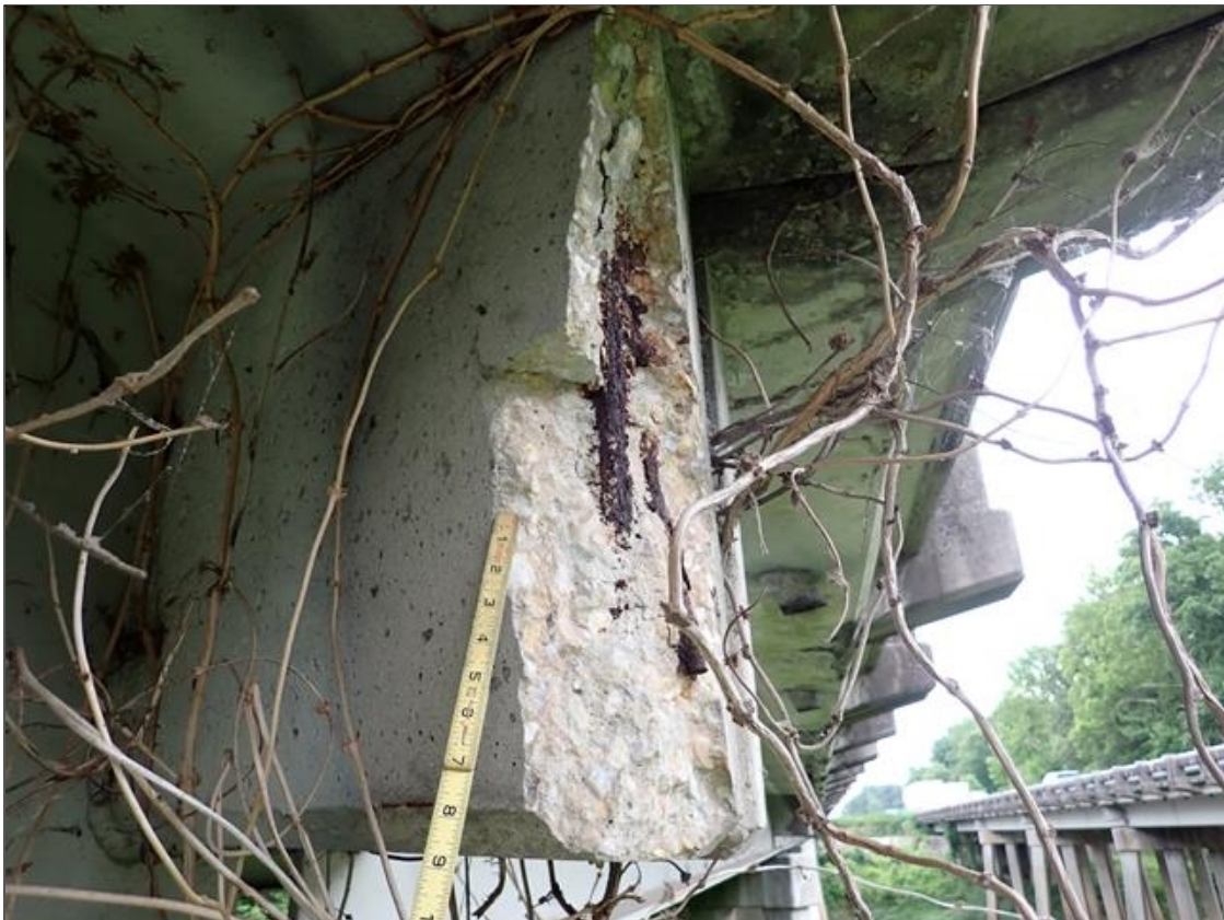
Span 1 Deck: (PAR) FAR END DIAPHRAGM AT RIGHT OVERHANG SPALL WITH EXPOSED REBAR 6 INCHES X 2 FEET X 4 INCH DEEP, 5 PERCENT SECTION LOSS.
