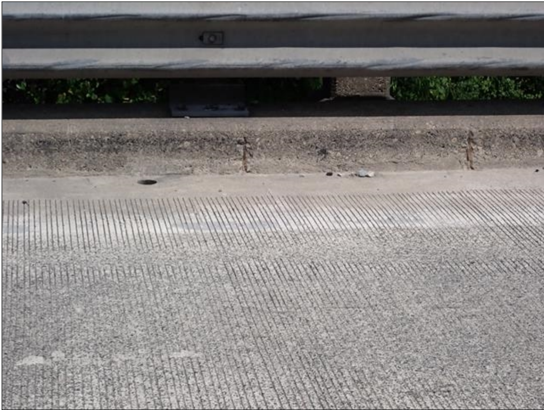
Span 3 Left Bridge Rail: 6 FEET AND 10 FEET FROM BENT 3 JOINT, BOTTOM OF CURB, TWO (2) SPALLS UP TO 8 INCHES DIAMETER X 1 INCH DEEP WITH EXPOSED REINFORCEMENT. NO MEASUREABLE SECTION LOSS IN EXPOSED REINFORCEMENT.
