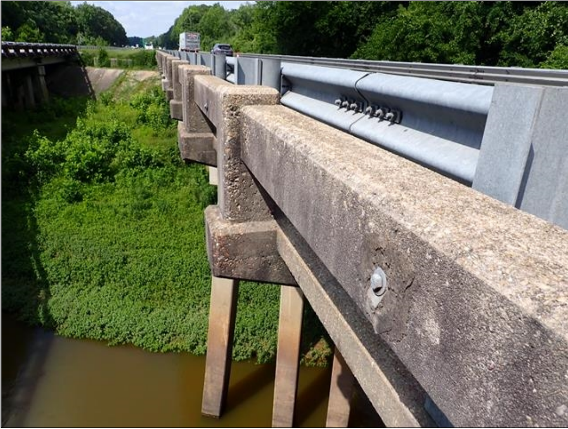
Span 4 Right Bridge Rail: (not found 2025) AT MIDSPAN EXTERIOR FACE, 1.5 FEET LONG X 9 INCHES HIGH X UP TO 1.5 INCHES DEEP SPALL
