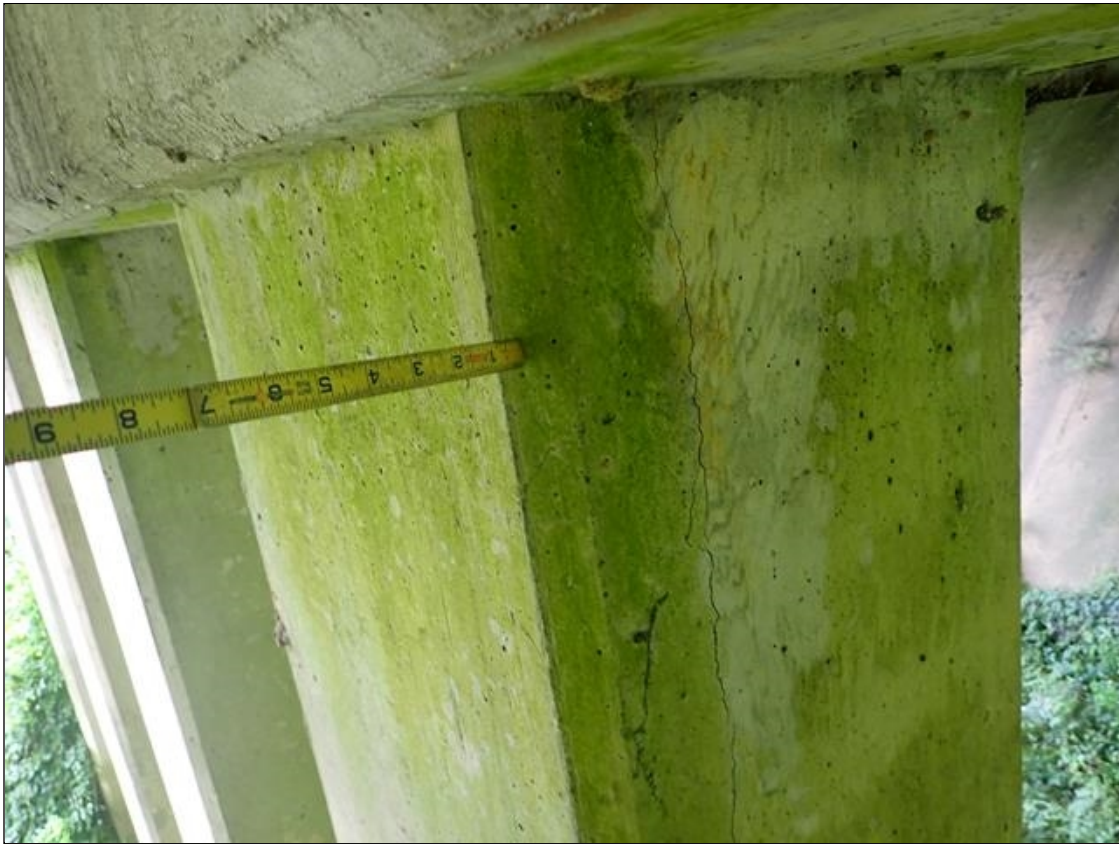
Bent 1 Pile 4: west face at cap, vertical crack (1/32 inch x 32 inch)
