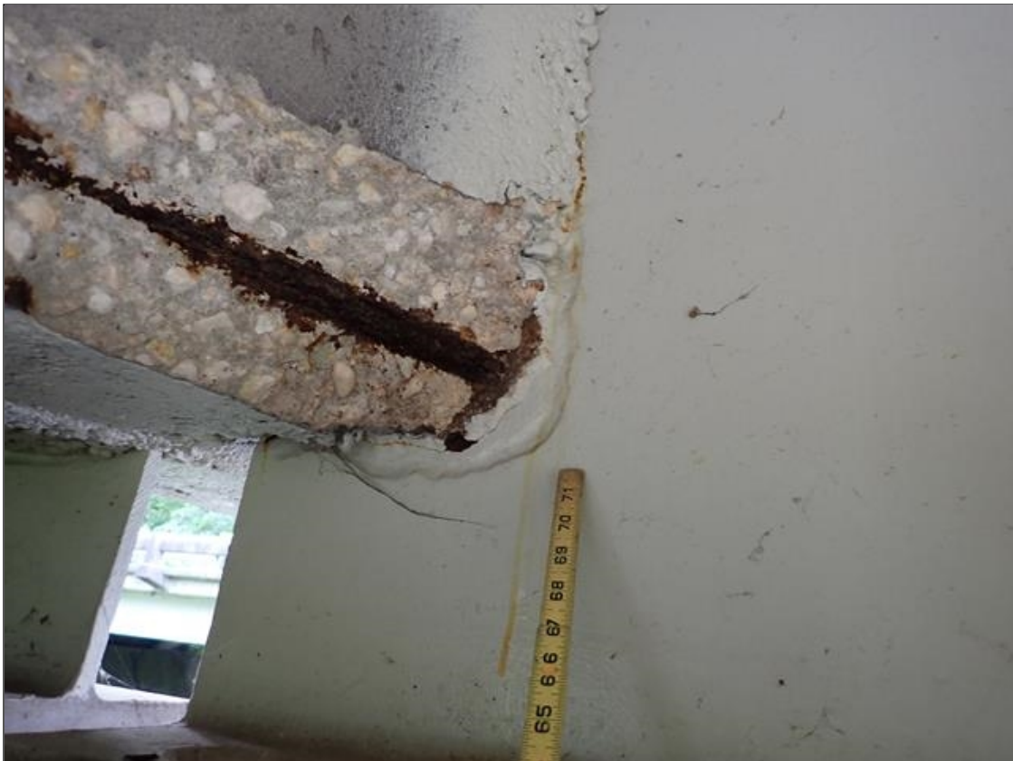
Span 6 Beam 4: (PAR) at bent 6, web adjacent to end diaphragm, corrosion with section loss (7/16 inch average remaining x 8 inch x 7 inch)
