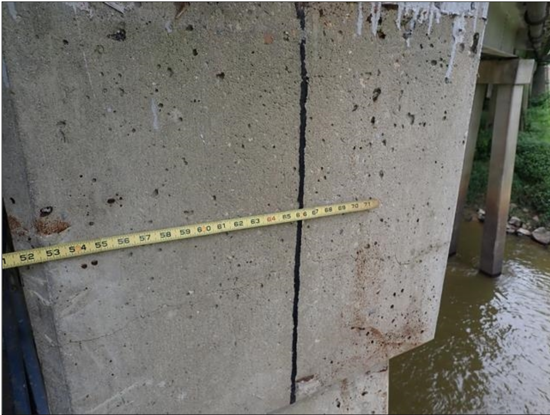
Bent 4 Cap 1: 30 INCHES LONG X 1/32 INCH WIDE HORIZONTAL CRACK, CENTER OF WEST END.
