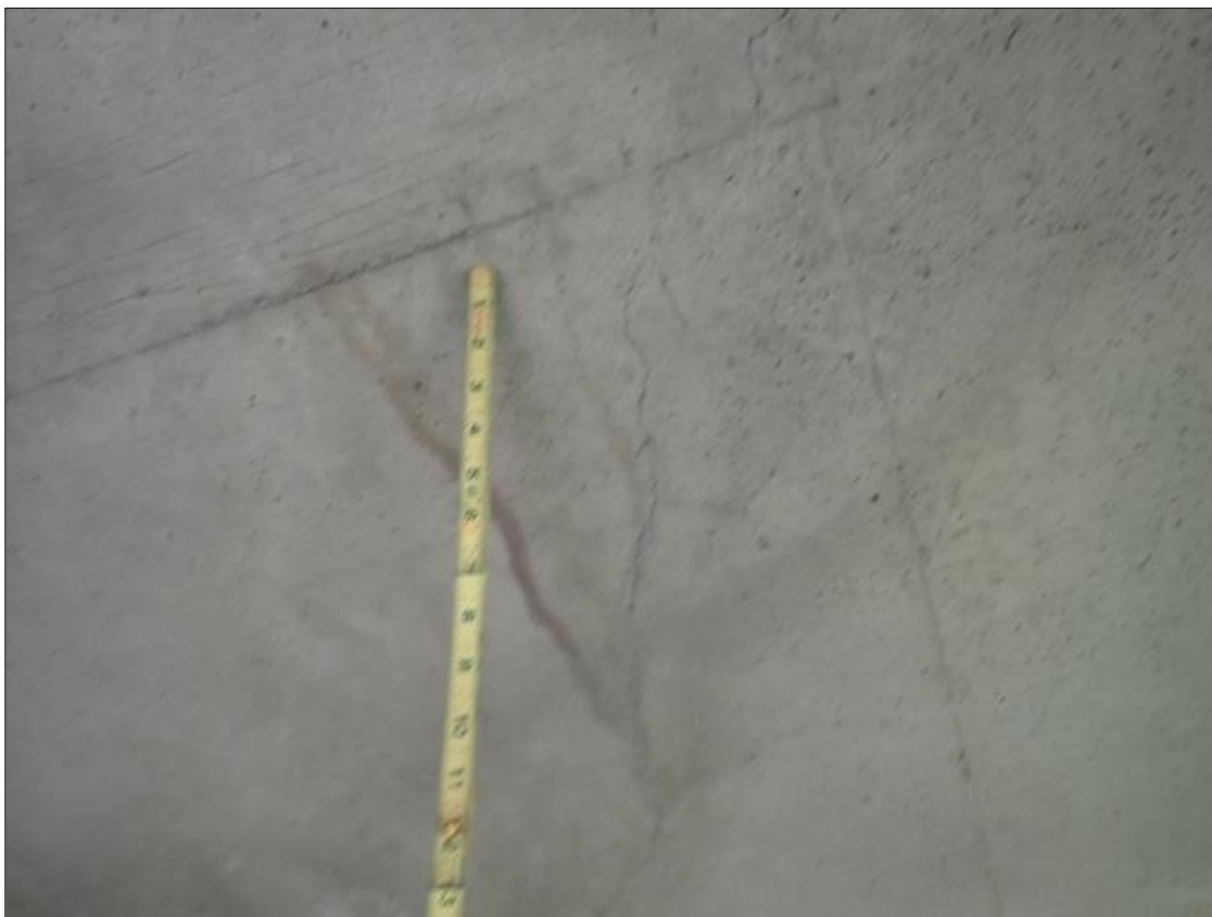
Span 3 Deck: 7 FEET LONG X 1/64 INCH WIDE DIAGONAL CRACK WITH EFFLORESCENCE IN UNDERSIDE OF DECK, BAY 3 AT BENT 2.
