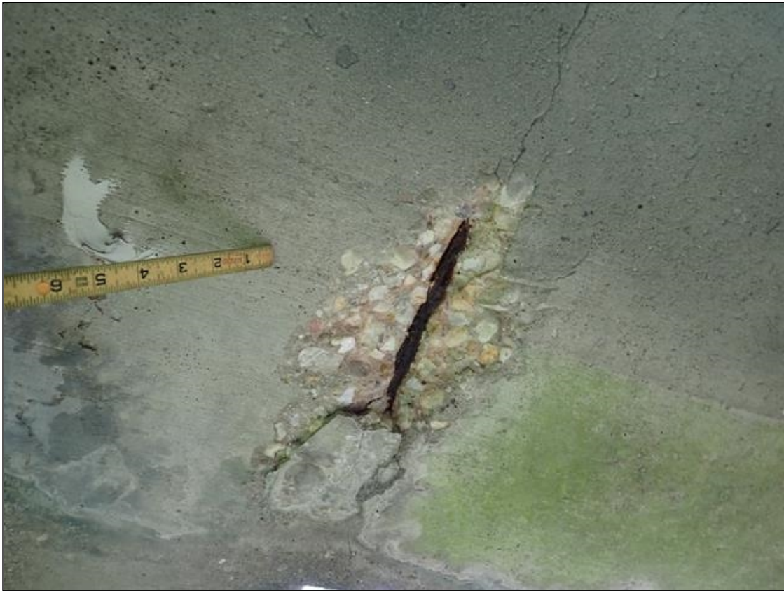
Span 2 Deck: (PAR) 15 FEET FROM BENT 2 IN LEFT OVERHANG SOFFIT SPALL WITH EXPOSED REBAR 6 INCHES X 8 INCHES X 1 INCH DEEP 5 PERCENT SECTION LOSS.
