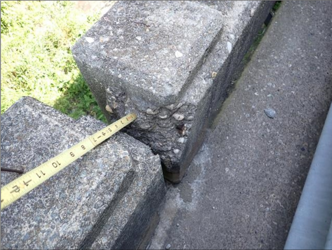
Span 8 Left Bridge Rail: TOP OF RAIL AT FIRST RAIL JOINT FROM END BENT 2, 8 INCHES WIDE X 8 INCHES HIGH X UP TO 3 INCHES DEEP SPALL WITH EXPOSED REINFORCEMENT
