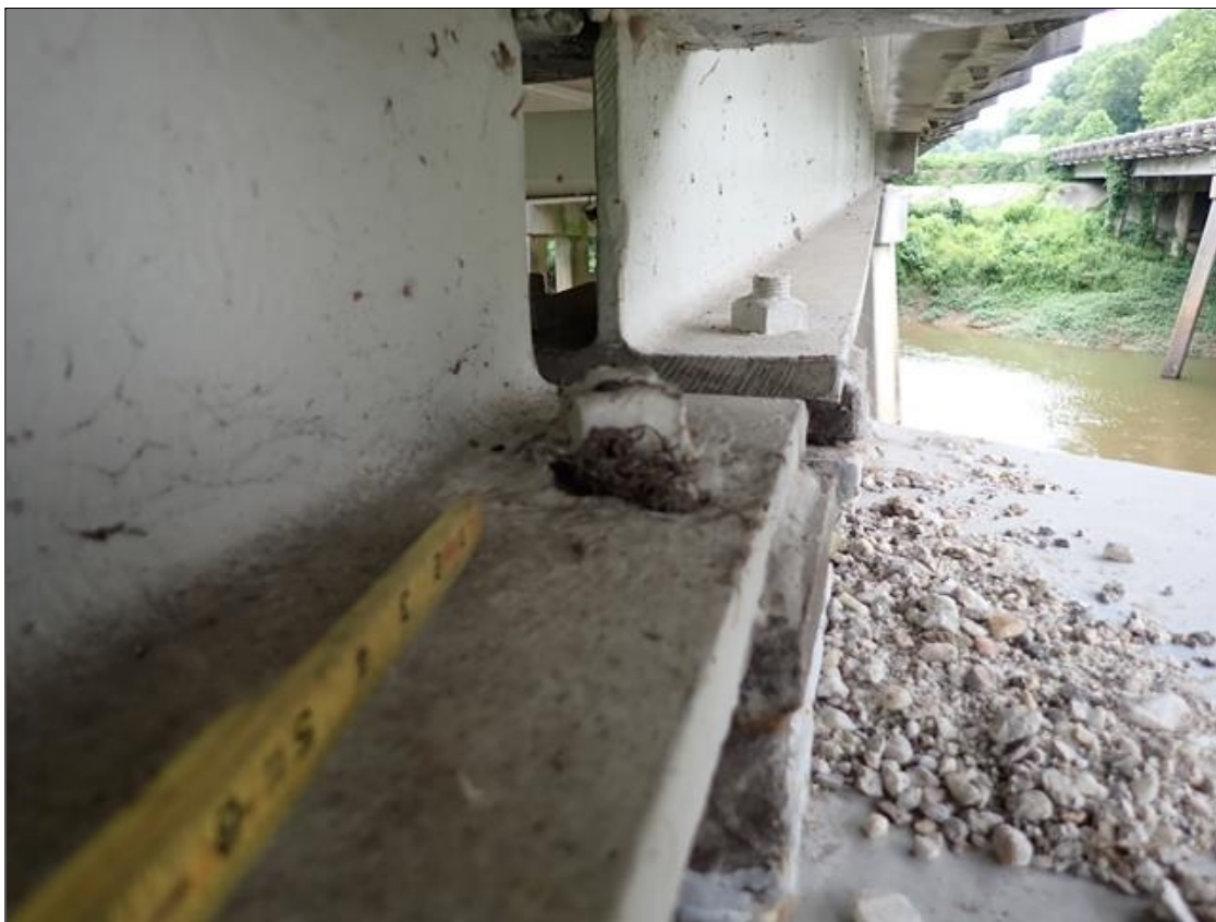
Span 3 Beam 4: (not found 2025) RIGHT ANCHOR BOLT NUT LOOSE.
