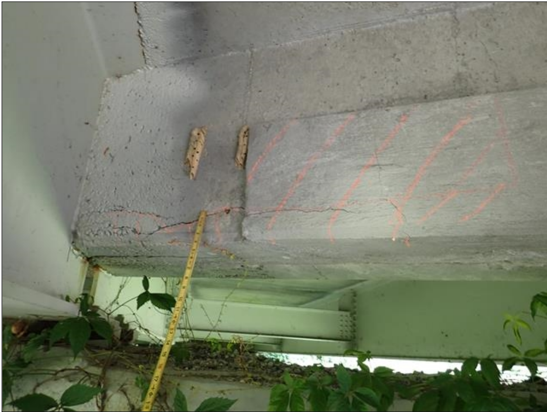
Span 7 Deck: AT BENT 7 BAY 3 DIAPHRAGM UNSOUND PATCH 7 FEET X 1 FOOT WITH 45 INCH X 18 INCH AREA OF DELAMINATION AND CRACKS UP TO 1/32 INCH
