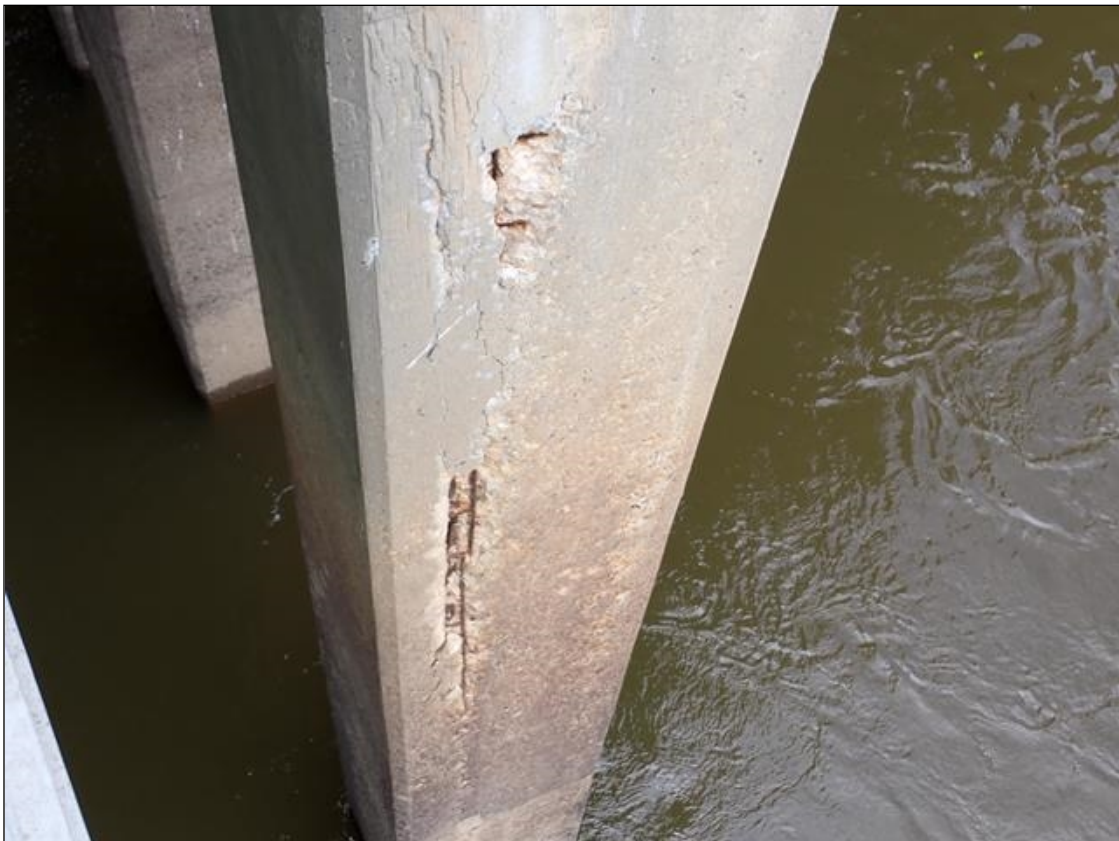
Bent 3 Pile 7: (PAR) starting at cap, east and south faces, delamination/spall (16 foot x 18 inch x 2 inch deep) with exposed rusted rebar (approximately 80 percent remaining) and cracks (up to 1/32 inch)
