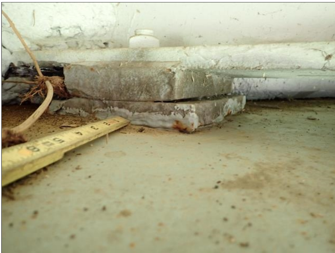
Span 1 Near Bearing 3: painted over section loss (less than 1/16 inch loss) with corrosion reactivating
