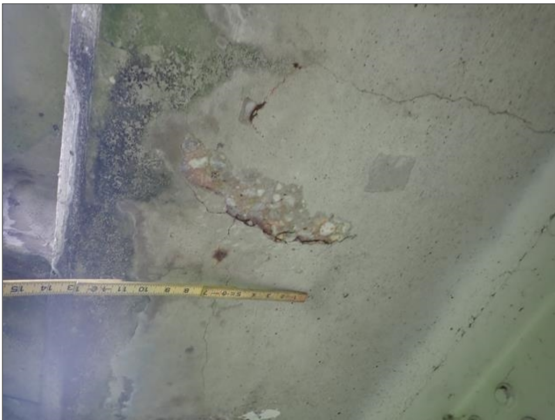
Span 2 Deck: RIGHT OVERHANG SOFFIT NEAR DRAIN 3, 4 INCHES X 8 INCHES X 1/2 INCH DEEP SPALL.
