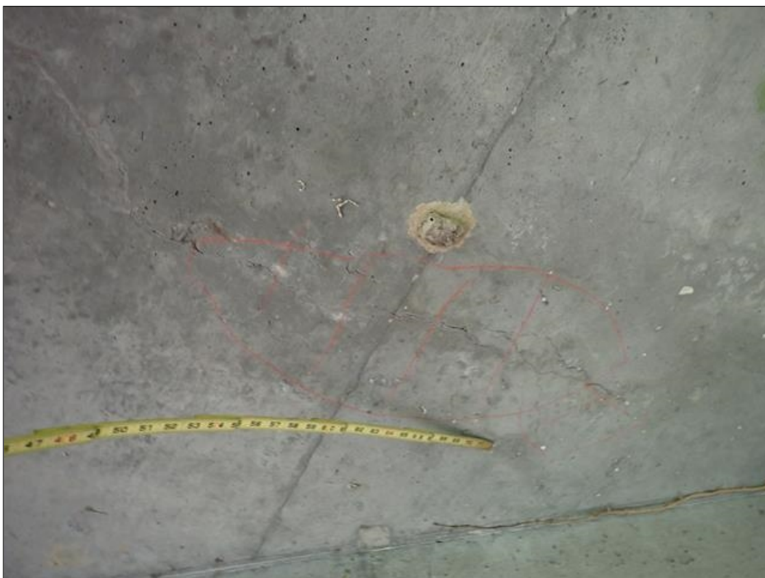
Span 8 Deck: underside in bay 3 adjacent to bent 7, delamination (30 inch x 12 inch) with cracks (up to 1/32 inch)
