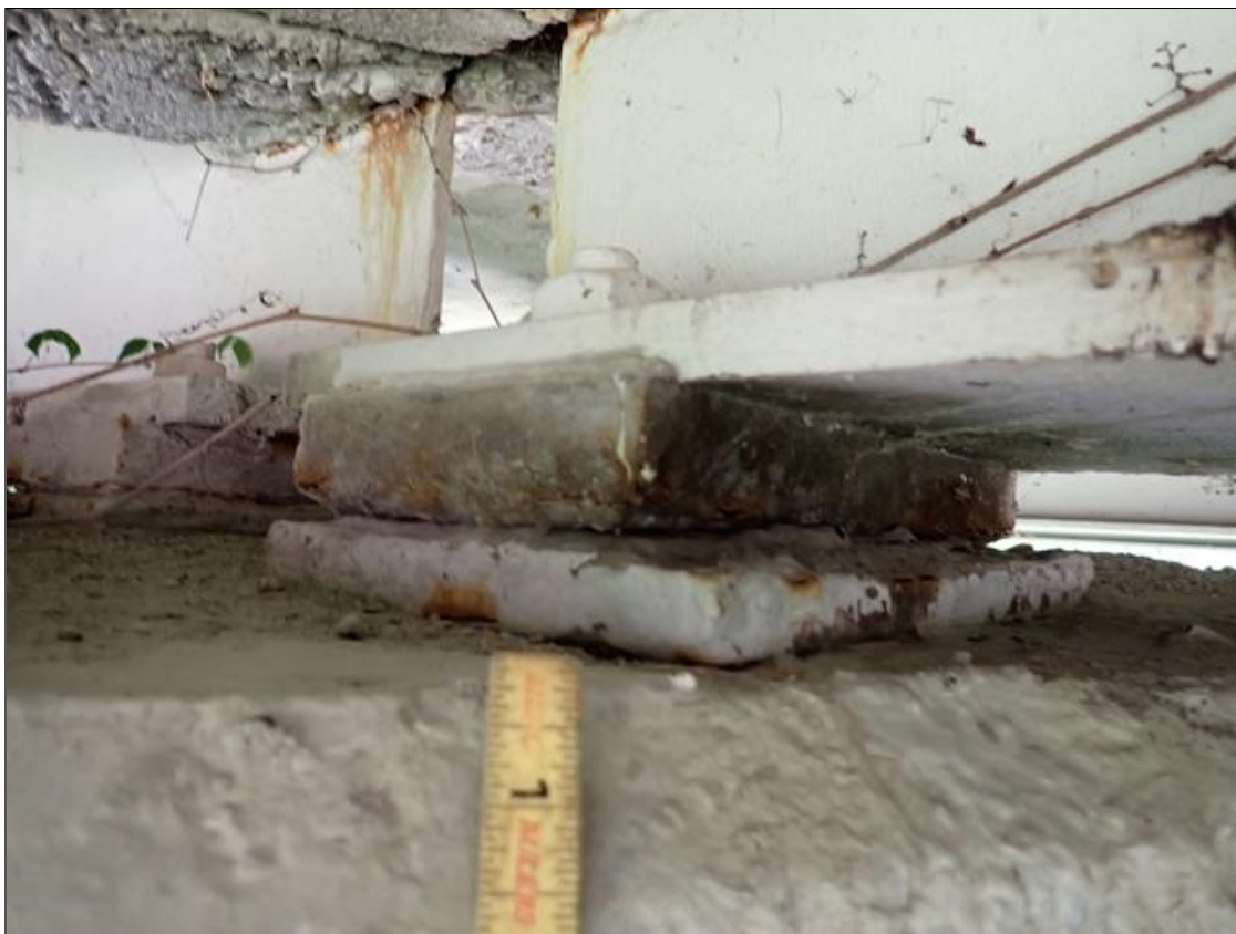
Span 8 Near Bearing 3: painted over section loss (approximately 85 percent remaining)
