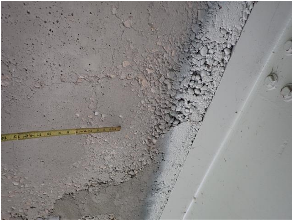
Span 7 Deck: SCATTERED AREAS OF HONEYCOMBING UP TO 3/4 INCH DEEP IN DECK UNDERSIDE IN ALL BAYS.
