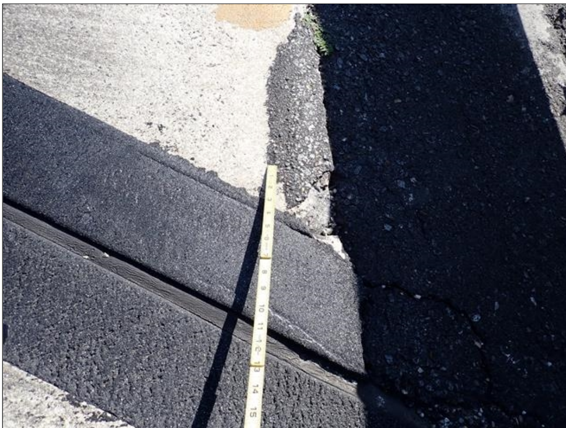
Approach 2: at southeast corner, spall (6 inch x 4 inch x 1.5 inch deep)
