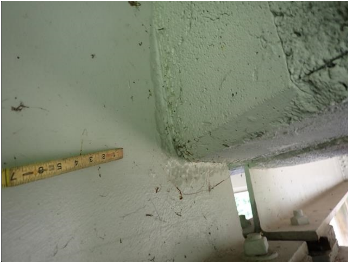
Span 3 Beam 3: (PAR) at bent 3, web adjacent to end diaphragm, painted over section loss (7/16 inch average remaining x 8 inch x 12 inch)
