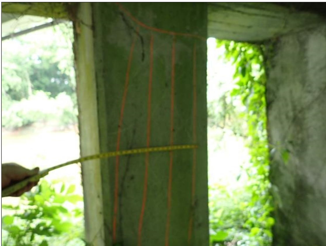
Bent 7 Pile 2: UP TO 5 FEET HIGH X 2 FEET WIDE AREA OF DELAMINATION IN NORTH AND SOUTH FACES, STARTING AT CAP
