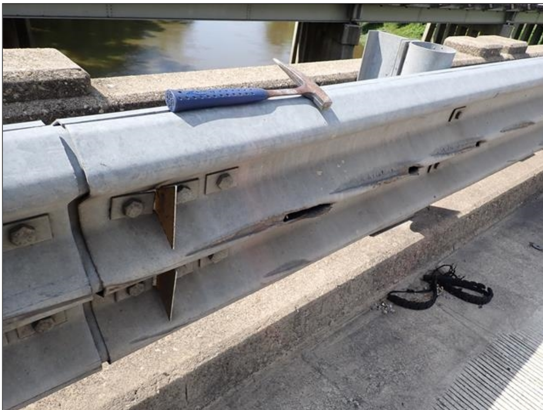
Span 5 Right Retrofit Bridge Rail: (PAR) IMPACT DAMAGE WITH SCRAPE MARKS AND THROUGH HOLES UP TO 4 INCH X 2 INCH IN RETROFIT RAIL AT SCATTERED LOCATIONS
