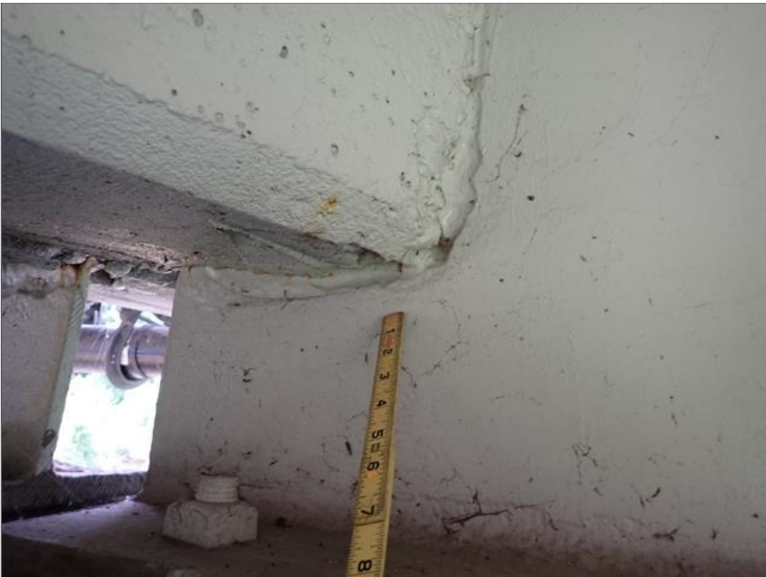
Span 7 Beam 1: (PAR) at bent 6, web adjacent to end diaphragm, painted over section loss (7/16 inch average remaining x 7 inch x 10 inch)
