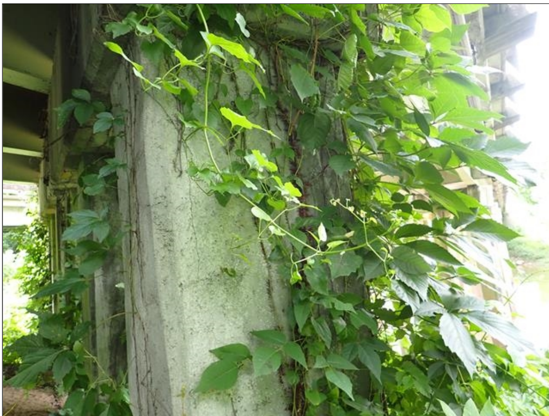
Bent 7 Pile 1: along pile, vegetation growth
