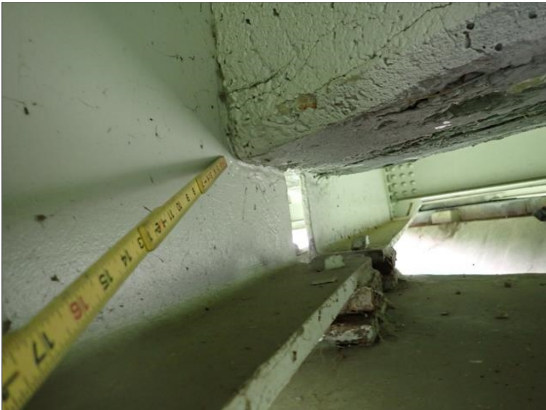
Span 2 Beam 3: (PAR) at bent 1, web adjacent to end diaphragm, painted over section loss (9/16 inch average remaining x 1 inch x 7 inch)
